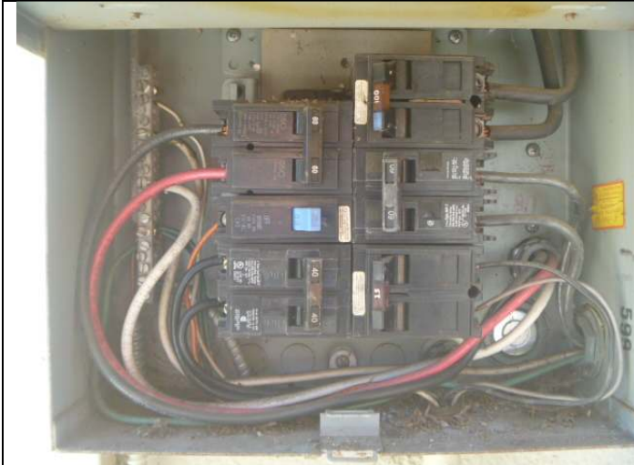
Main service panel.
