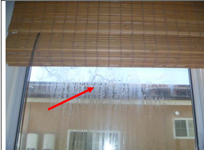
Fogged window pane (dual pane type) in the south front bedroom.
