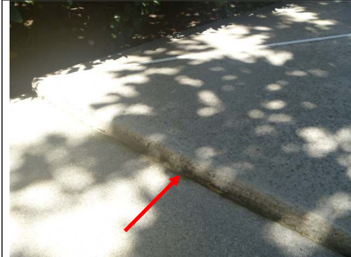
Uneven joint at the left rear of the pool deck.
