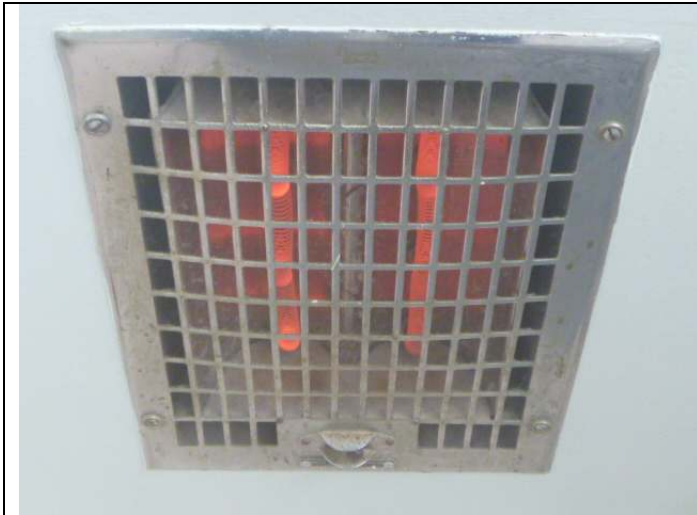
South bathroom old wall heater coil.
