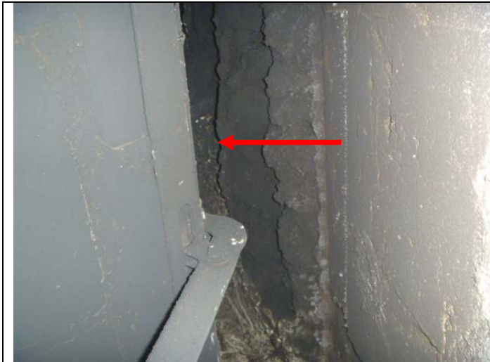
Fireplace damper in the open position.
