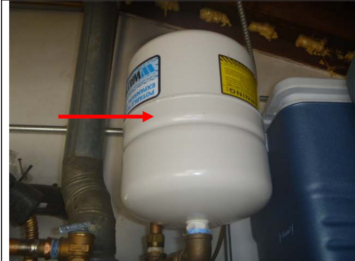
Thermal expansion tank above the water heater.
