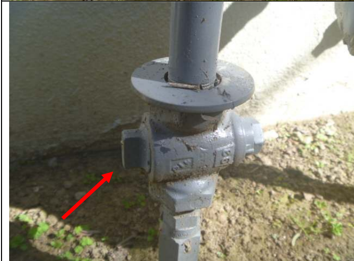
Gas shut off valve.
