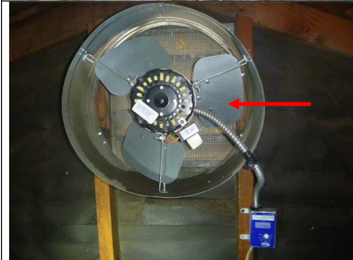
Attic ventilation fan.
