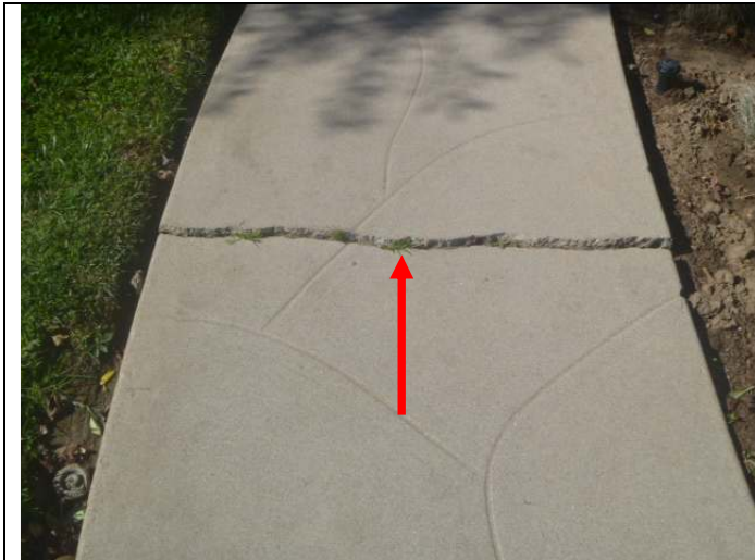
Front walkway crack and unevenness.
