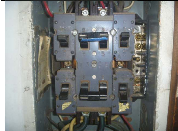
A closer view of the breakers. Note: The obsolete circuit breaker set.
