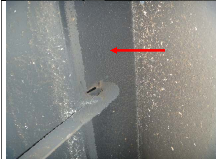
Fireplace damper in the closed position.
