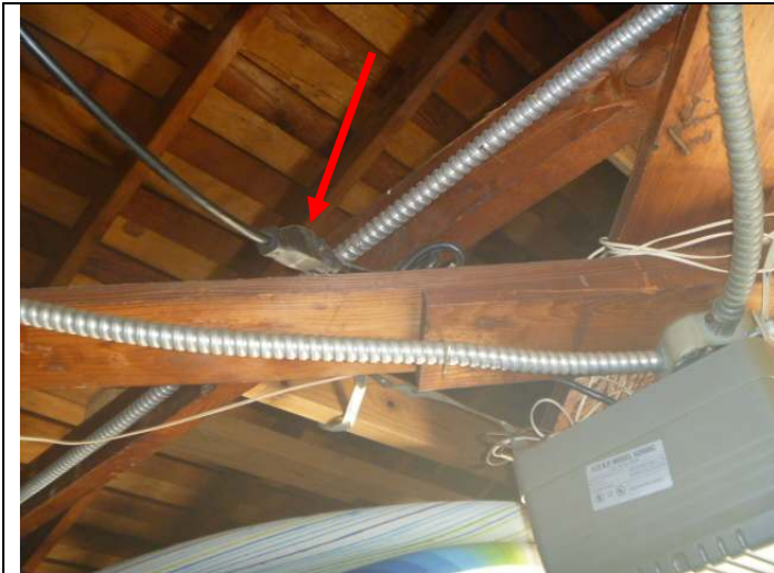
Extension cord wiring to the garage door opener.
