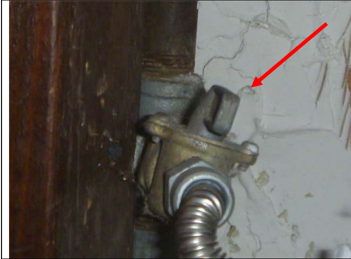
Old dryer gas valve below the water heater.
