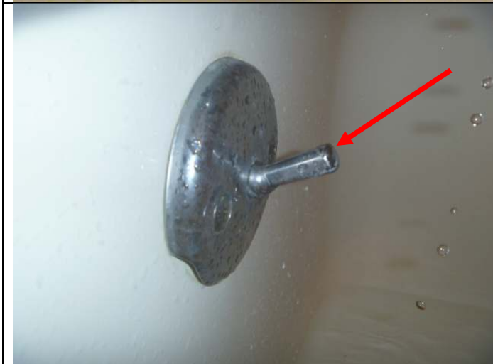
North bathroom tub stopper control. Note: The stopper is inoperative.
