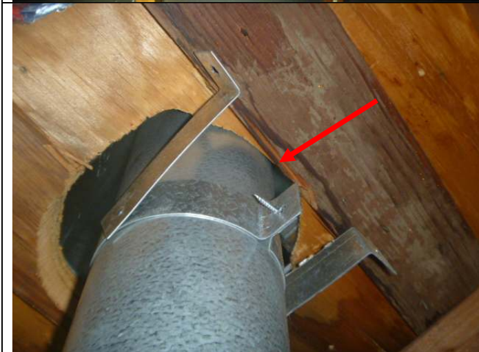
Central heater vent pipe without the proper (1" minimum) clearance at the roof sheathing.
