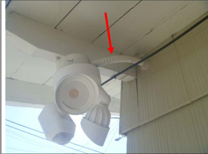
Flexible conduit wiring under the garage right front eave. Note: The wiring is not rated for exterior use, however, this is possibly the original installation.
