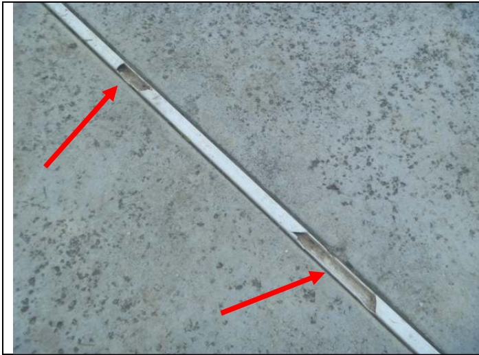
Damaged vinyl along the pool deck expansion joints.
