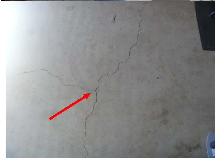
Minor cracks in the garage slab floor.
