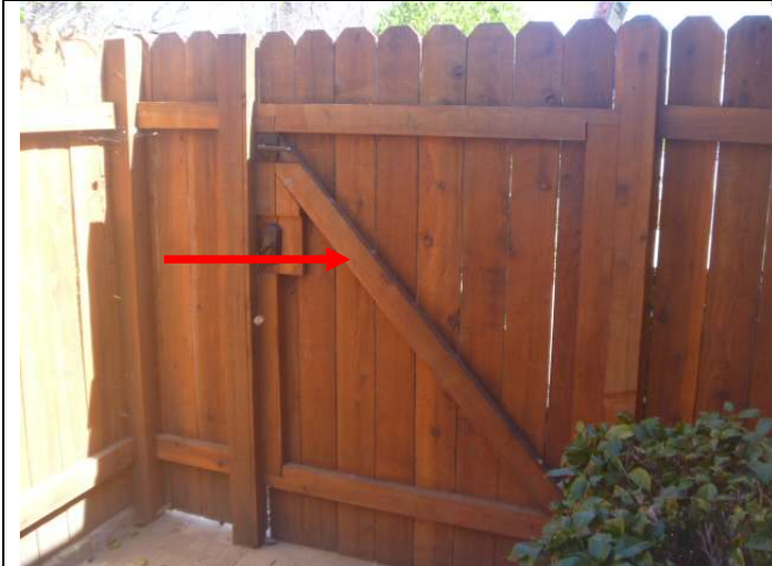
North side gate with pool area access. Note: The gate is not properly self-closing.
