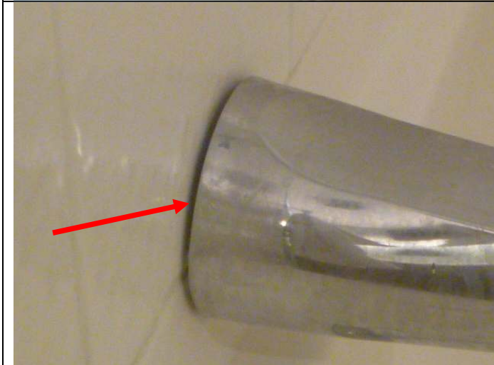
Gap at the north bathroom tub spout.
