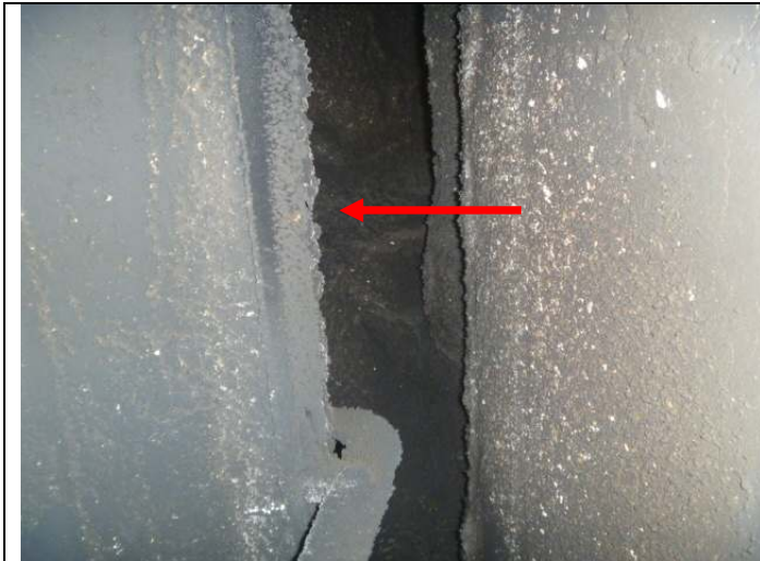
Fireplace damper in the open position.
