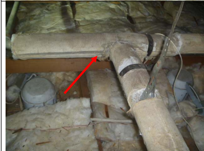
Asbestos pipe insulation in the attic.
