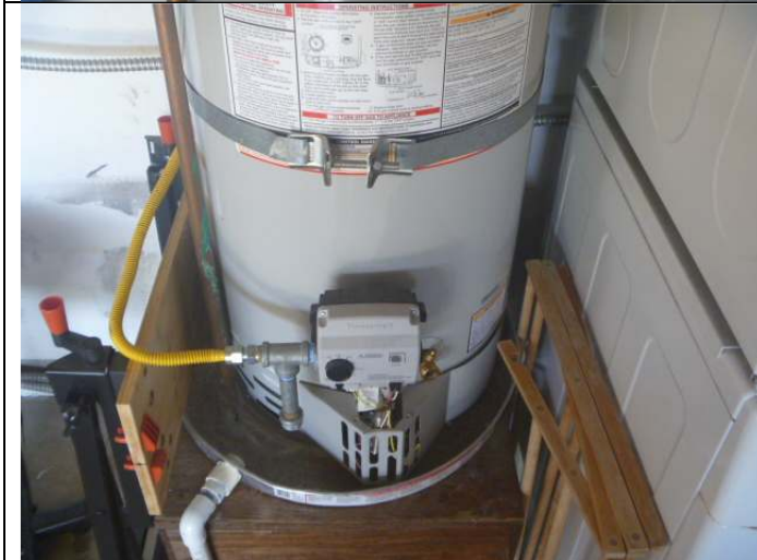
Water heater lower section.
