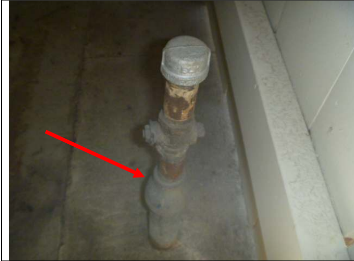
Old gas piping for a previous pool heater.
