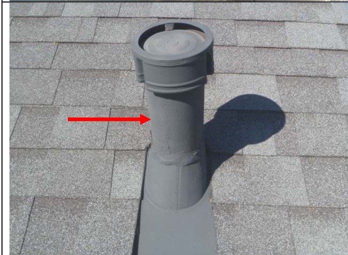
Transite vent pipe (for the original water heater and not in use).
