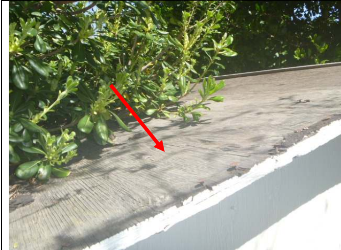
Pool enclosure roof without a roof covering.
