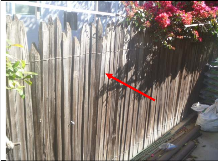
Old north side wood fencing.
