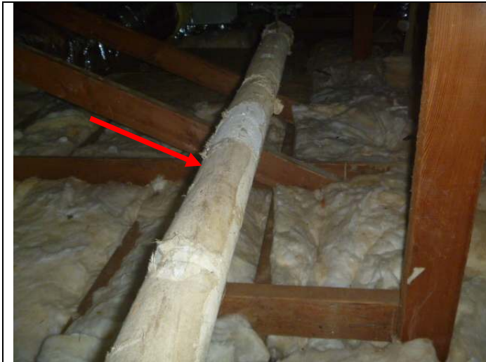
Asbestos pipe insulation in the attic.
