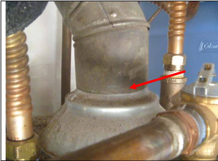
No securing screws for the water heater vent pipe at the downdraft diverter.
