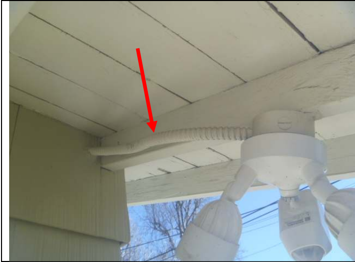
Flexible conduit wiring under the garage left front eave. Note: The wiring is not rated for exterior use, however, this is possibly the original installation.
