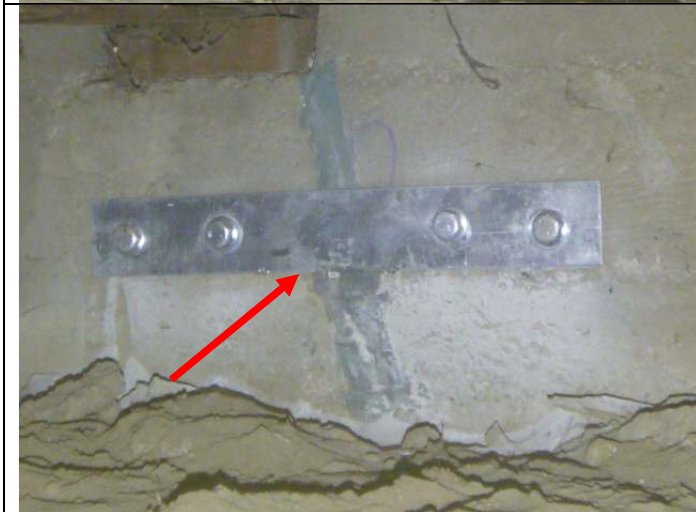
Foundation crack repair (south wall toward the left front).
