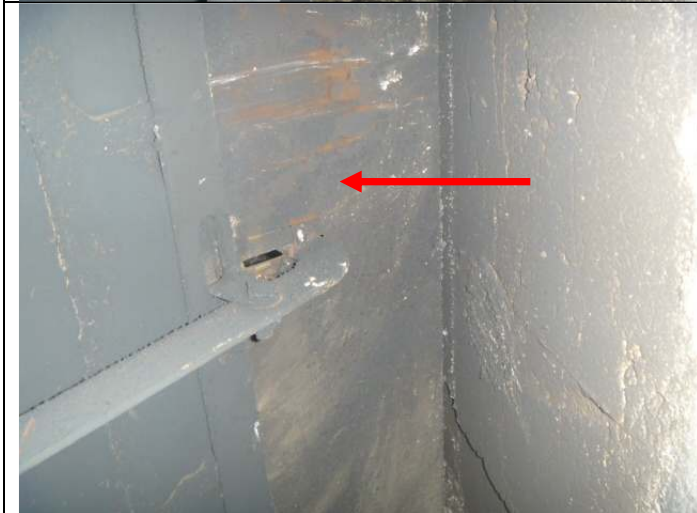
Fireplace damper in the closed position.
