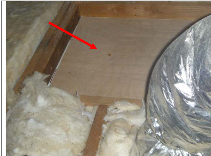
Small area with missing attic insulation.
