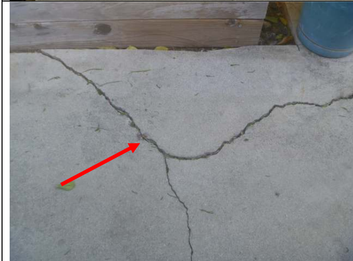
Cracks in the north side walkway.
