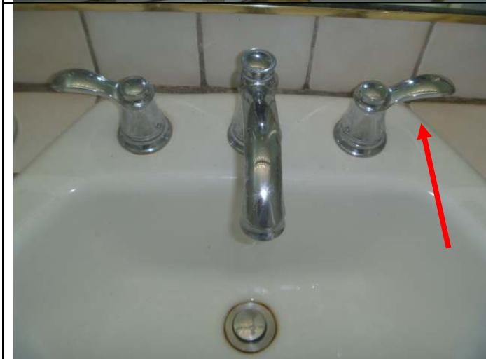
South bathroom sink. Note: The cold water faucet is somewhat stiff (minor).
