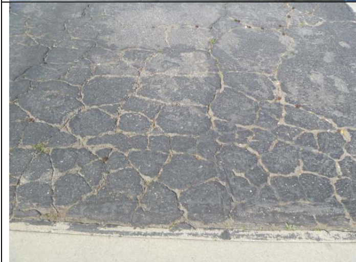
Old and cracked asphalt driveway.
