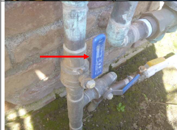
Main water valve.
