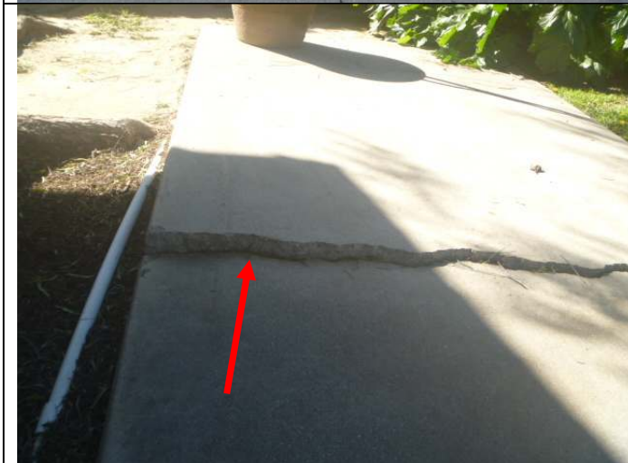
Cracked and lifted left rear walkway.
