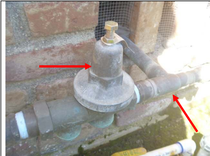
Copper water piping and the water pressure regulator.
