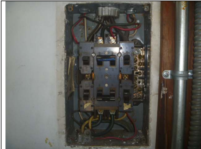
Upper subpanel in the garage.
