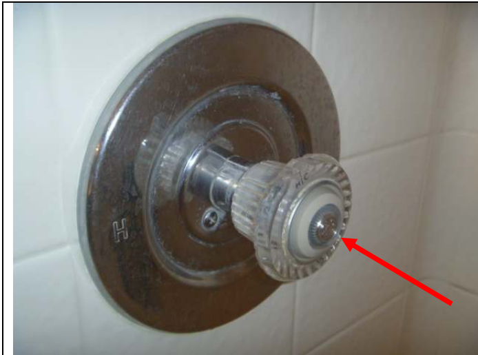
North bathroom shower/tub fixture. Note: The valve (pull type) is somewhat stiff.
