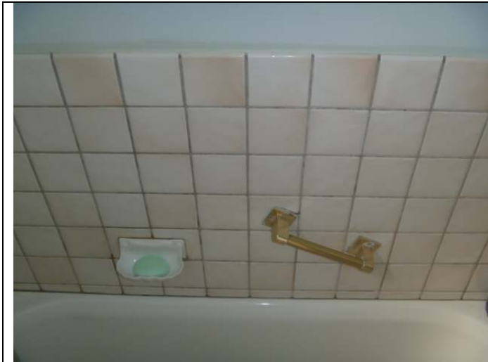
South bathroom tub tiles. Note: The tiles backing type was not determined.
