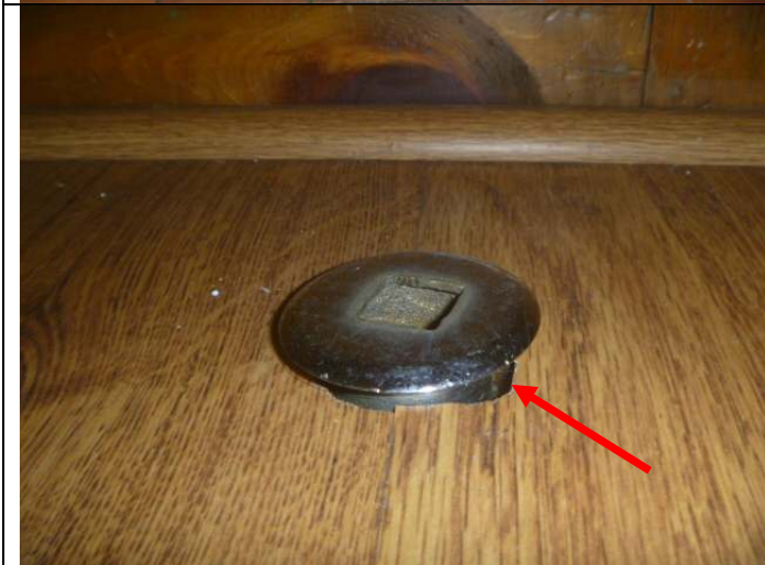
Fireplace gas valve not flush with the floor.
