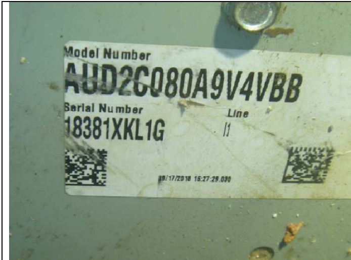
Heater/fan unit model and serial numbers (indicating a 2018 build date).
