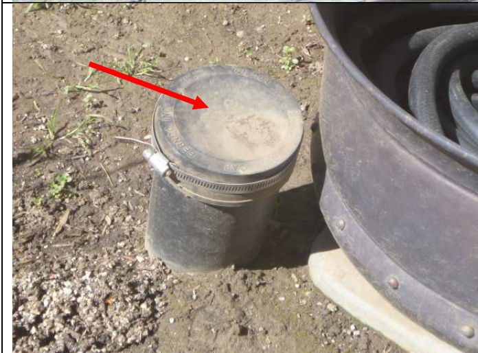
Main drain cleanout at the front exterior.
