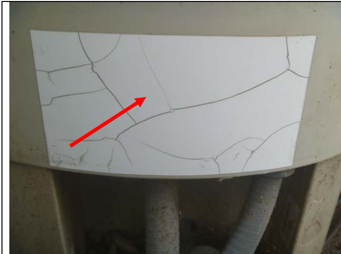
Air conditioner faded and illegible label.
