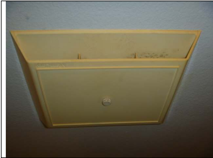
Downstairs 3/4 bathroom vent fan. Note: The fan is relatively noisy.
