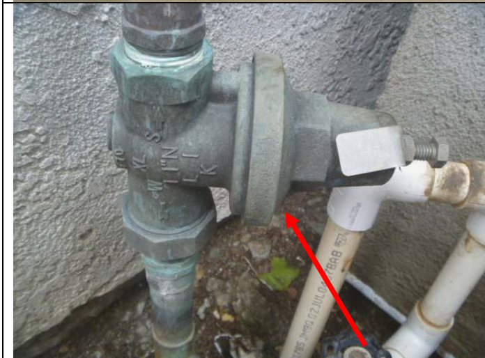
Inoperative water pressure regulator.
