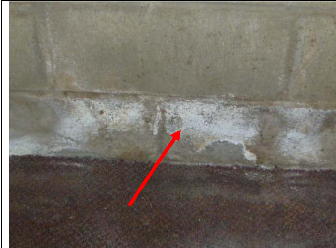
Efflorescence along the sunroom lower rear interior wall.
