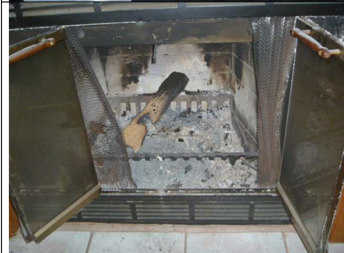
Fireplace. Note: There is no hearth extension (matching floor tiles only) along the front of the fireplace.
