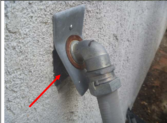
Air conditioning electrical conduit loose at the wall.
