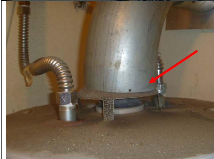
Vent piping (non-powered) immediately above the water heater.
