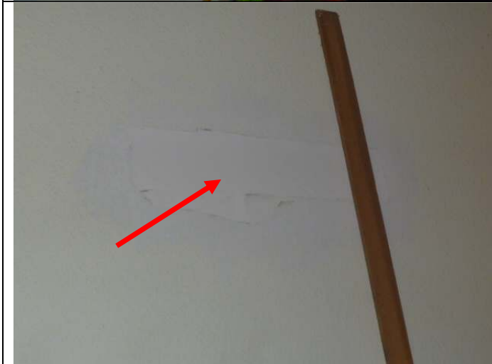
Garage rear wall repair (on the backside of the downstairs 3/4 bathroom shower).
