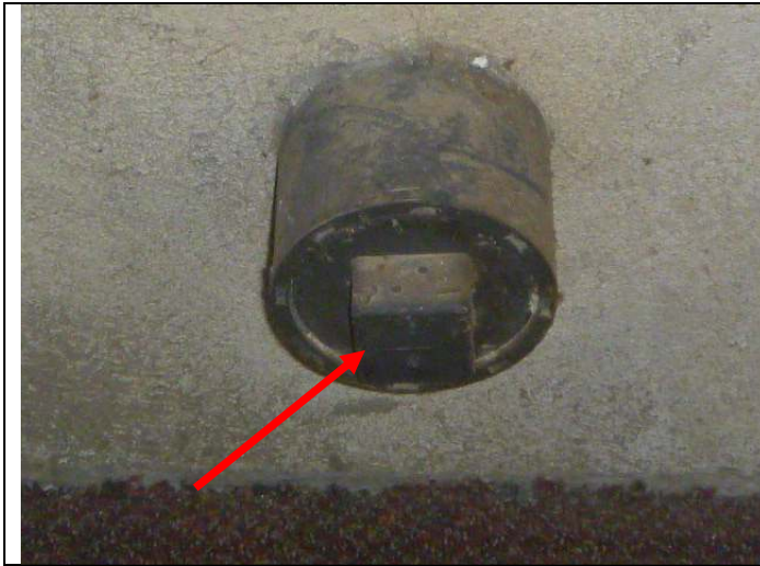
Main drain cleanout the sunroom lower left front wall.
