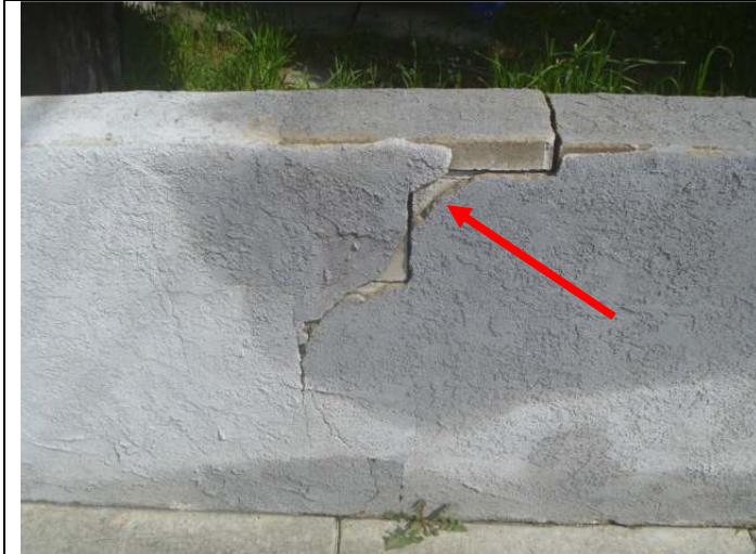
Cracks in the left front block/stucco wall.
