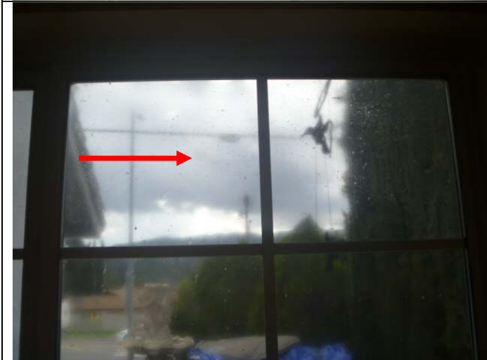
Fogged window pane (dual pane type) at the kitchen sink.
