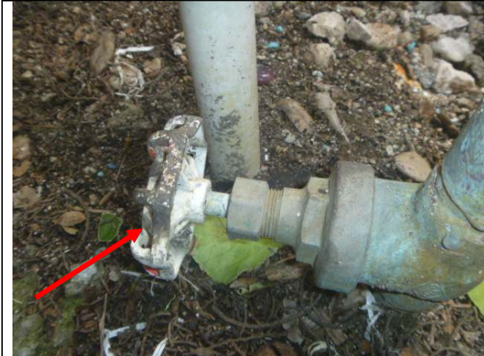
Older gate type main water valve.
