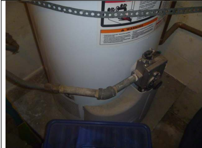
Water heater section.
