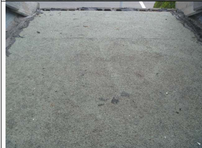
Left front dormer roof (off the west front bedroom). Note: There is a similar area off the east front (primary) bedroom.
