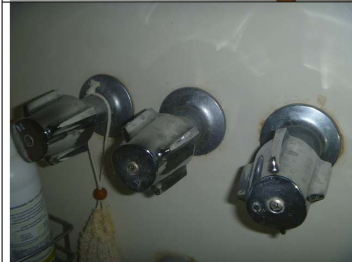
Full bathroom shower/tub fixtures. Note: The hot and cold water valves squeak during operation. The shower/tub diverter valve leaks.
