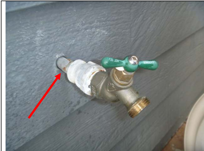
Left front exterior hose bib. Note: The pipe is somewhat loose at the wall.
