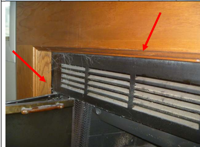
Fireplace mantel without the proper clearance around the fireplace opening.
