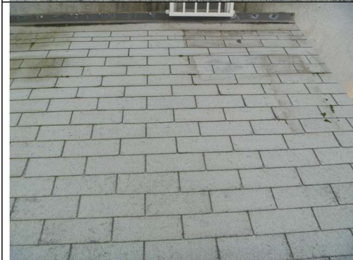
Sunroom roof. Note: The roof slope is insufficient for shingles.
