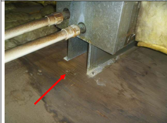
No catch pan below the air conditioner coil. Note: The moisture related discoloration in the plywood
