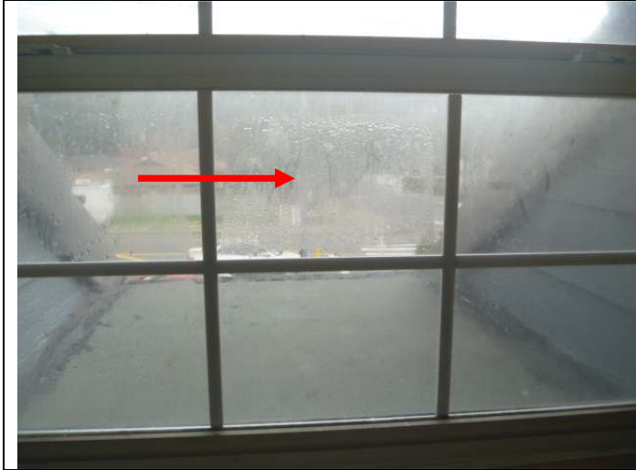
Fogged window pane (dual pane type) at the front of the west front bedroom.
