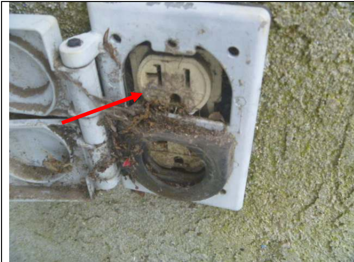
Left rear patio receptacle without ground fault circuit interrupter (GFCI) protection.
