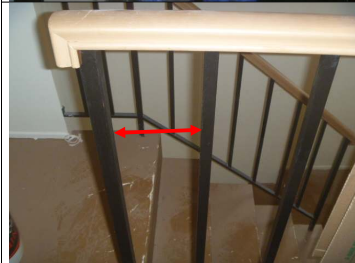
Hallway railing with relatively wide spacing – older style installation.
