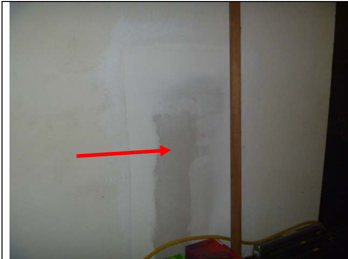
Garage rear wall repair (on the backside of the downstairs 3/4 bathroom shower).
