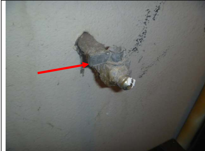
Older gas valve for the dryer.
