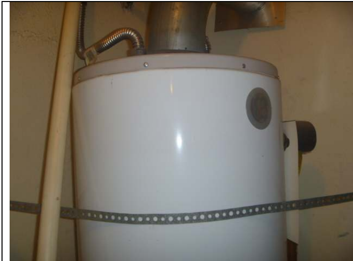
Water heater upper section. Note: The required seismic bracing is to be installed.
