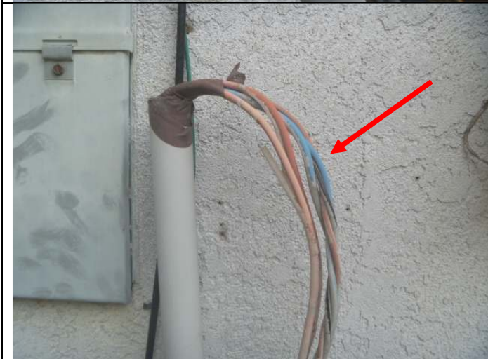
Disconnected larger gauge wiring to the right of the main service panel.
