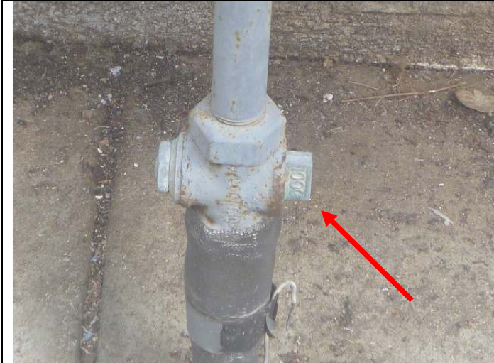
Gas shut off valve.
