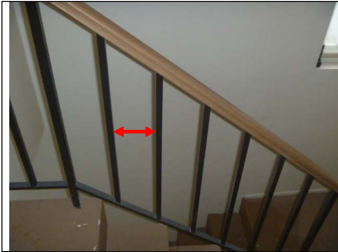
Stairway railing with relatively wide spacing – older style installation.
