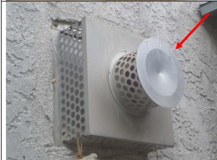
Water heater vent outlet at the side exterior wall.
