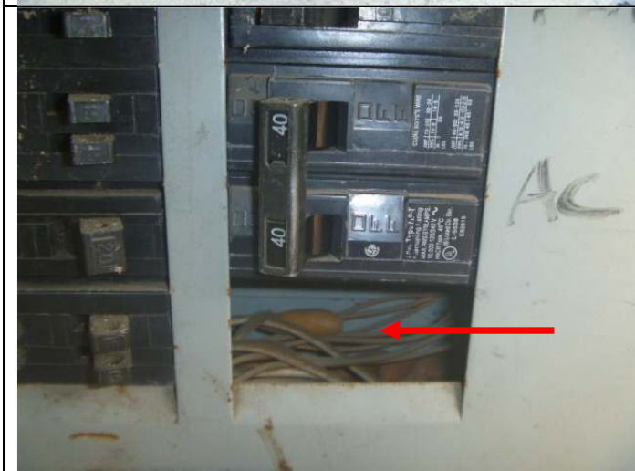
An open knockout in the panel interior cover.
