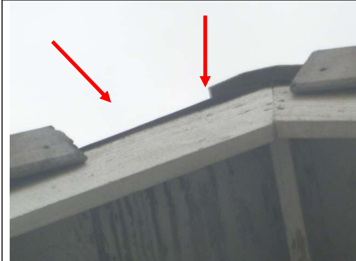
Missing tiles at the east gable end of the upper roof.
