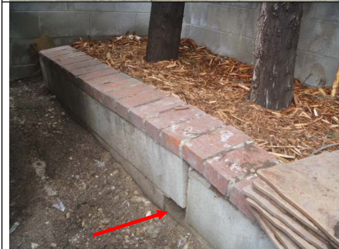
Displacement in the right rear planter wall.
