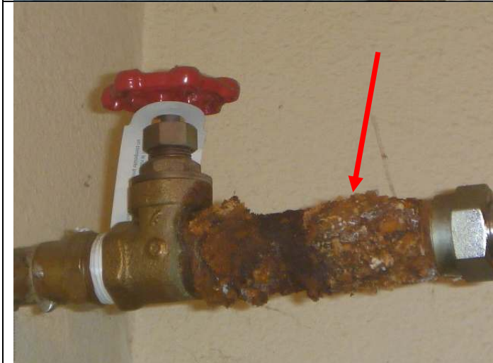
Noticeably rusted water piping at the water shut off valve above the water heater.
