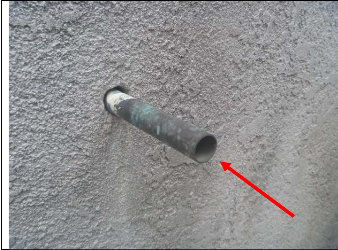
Water heater pressure relief valve outlet pipe pointing outward (vs. downward) at the exterior wall.
