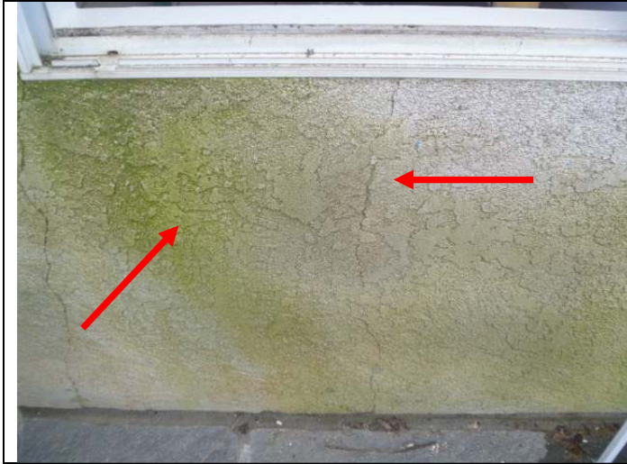
Stucco cracking and discoloration.
