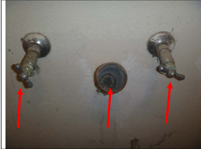
Washer valves and drain. Note: The valves are older and leak.
