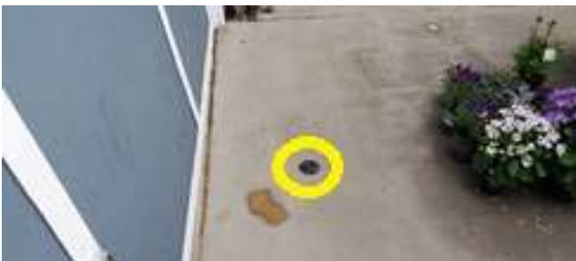
Cleanout in driveway.
