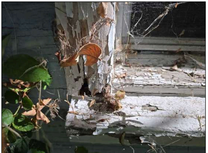
Deteriorated wood trim, consult termite report
