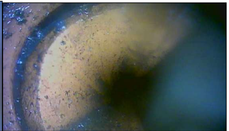
Standing water present in sewer line at 7.5 feet.
