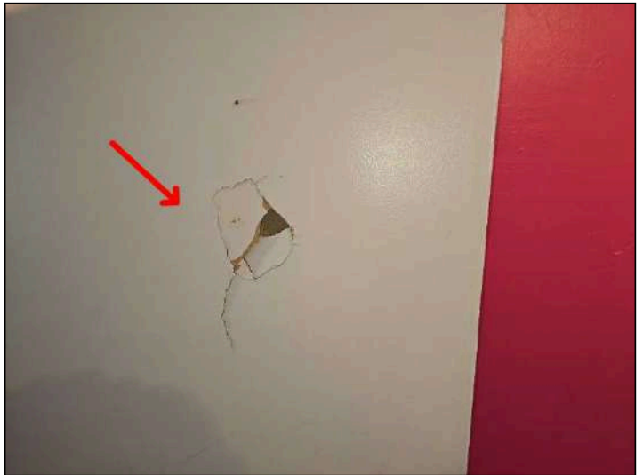
Large hole(s) present, recommend repair or replace east bedroom
