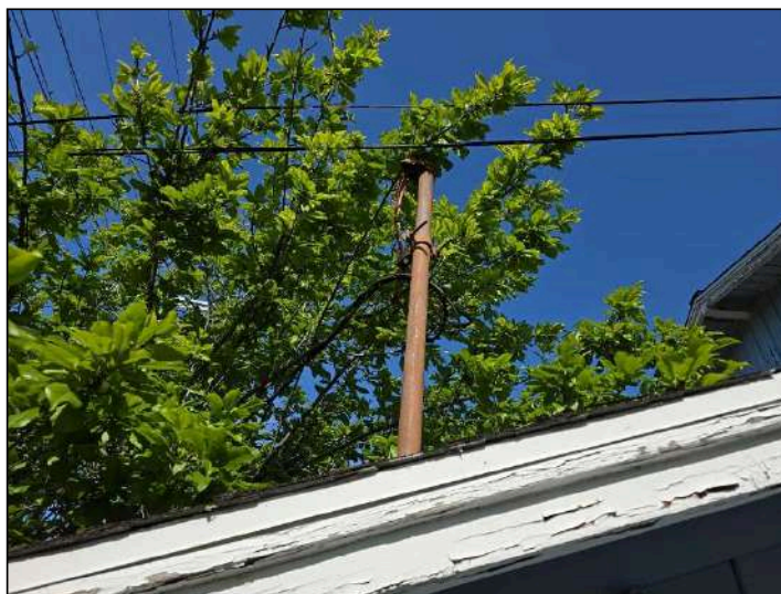
Trees/vegetation close/in contact with service entrance/wires, recommend repair
