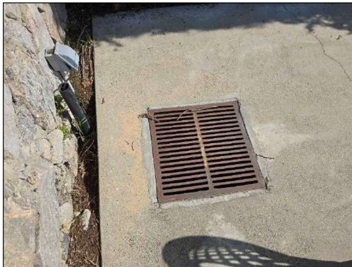
Does not appear to be functioning properly recommend repair
