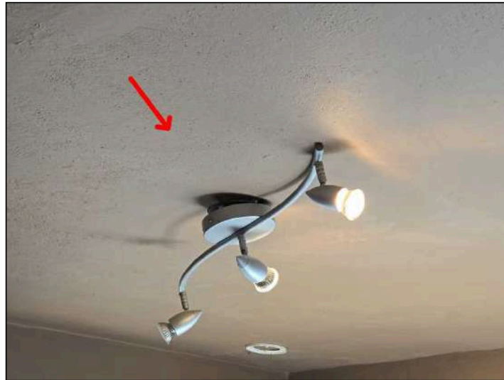
Loose fixtures, recommend repair
