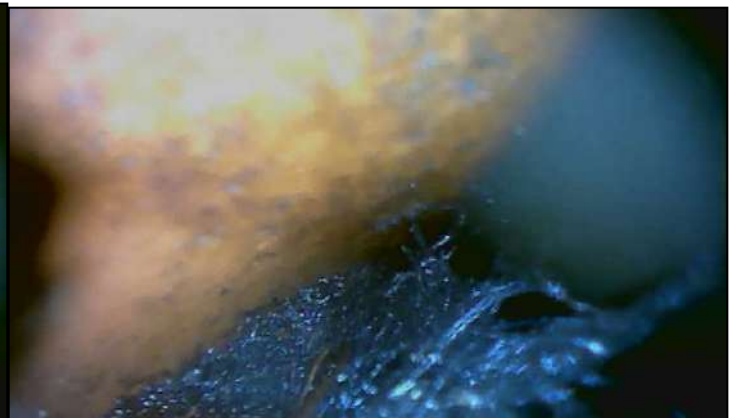
Root intrusion present in sewer line at 10 feet.
