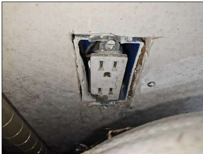
Broken outlet(s) Potential hazard, recommend repair
