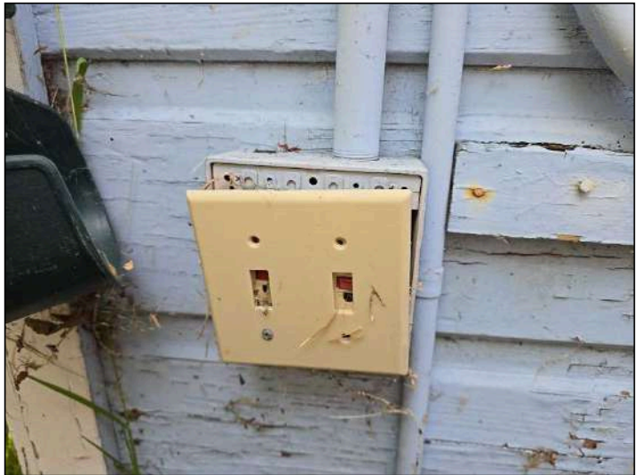
Weather proof cover improper east side recommend repair
