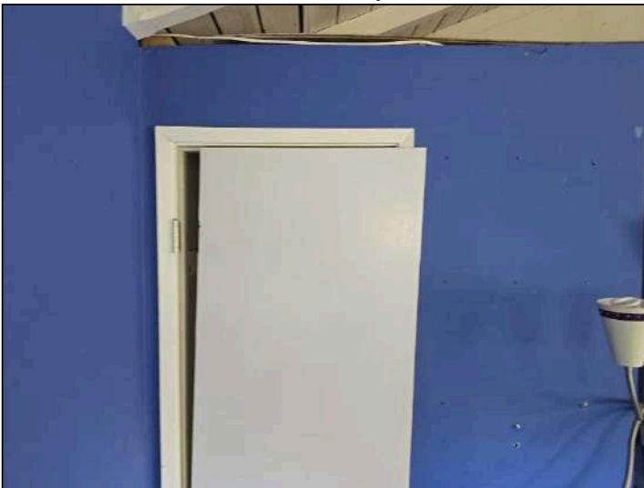
Door off hinges 2nd floor bedroom recommend repair
