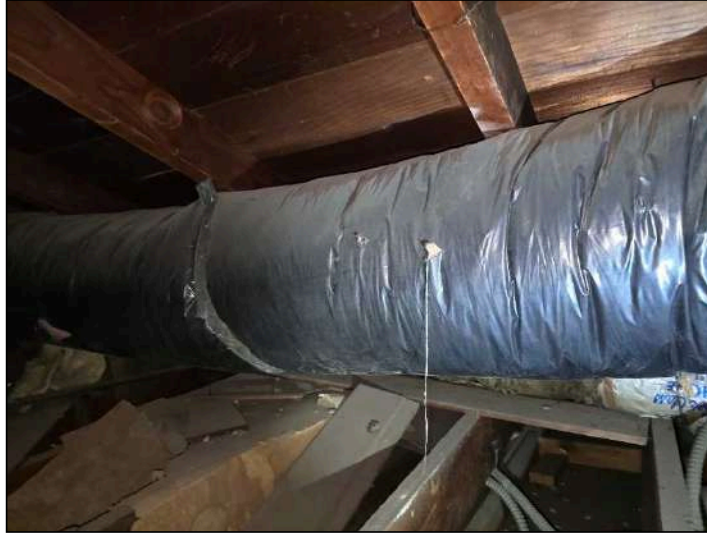
Holes in ducts, recommend repair
