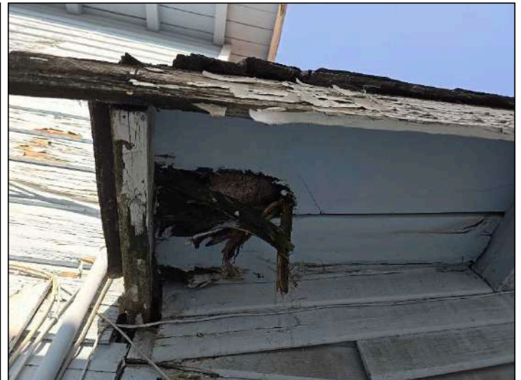
Deteriorated wood observed, recommend repair, consult termite report
