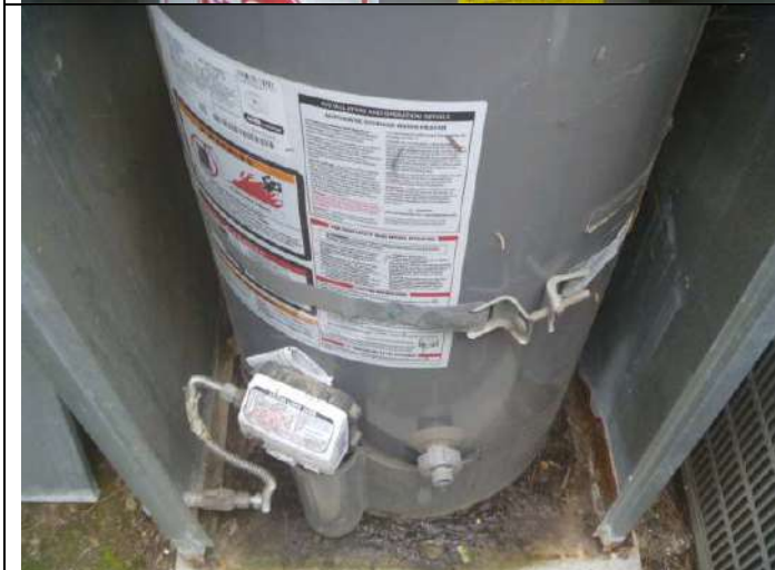
Water heater lower section.
