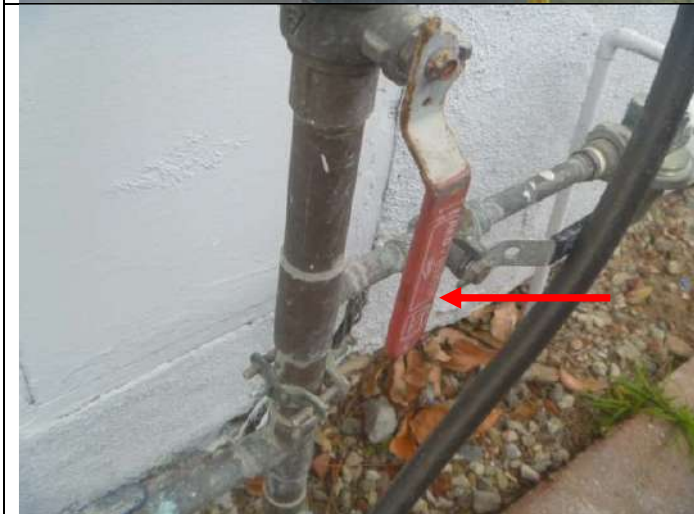
Main water valve.
