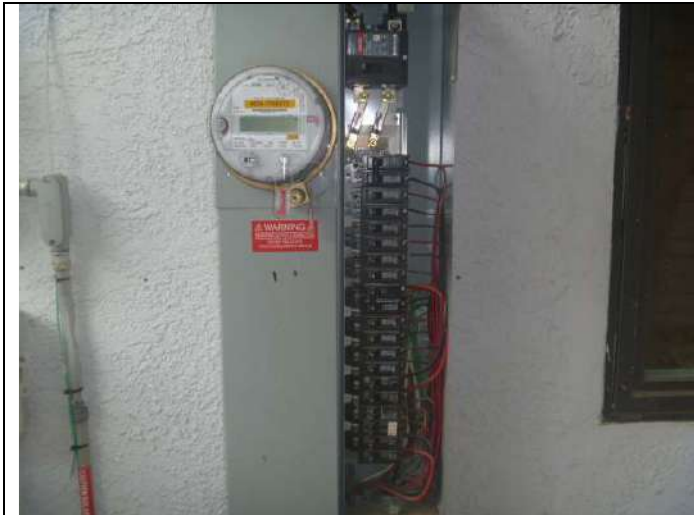
Main service panel.
