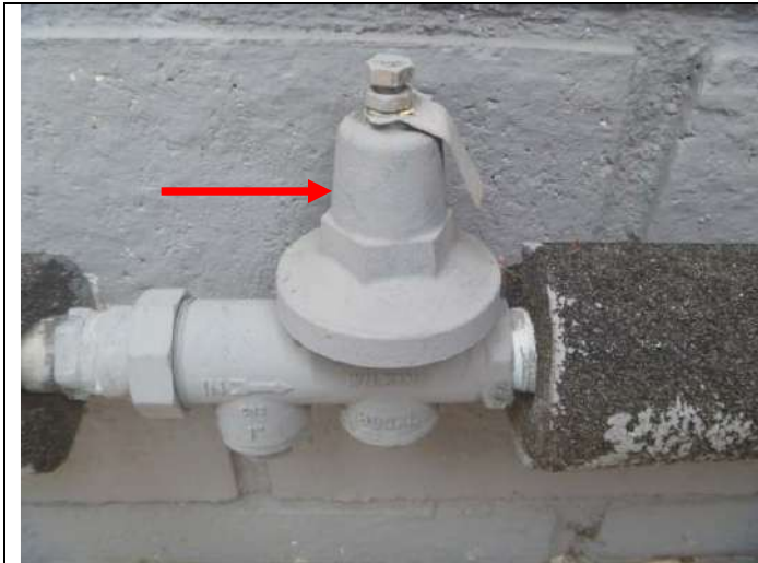
ADU water pressure regulator.
