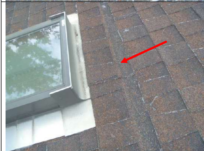
Displaced shingles at the right rear skylight.
