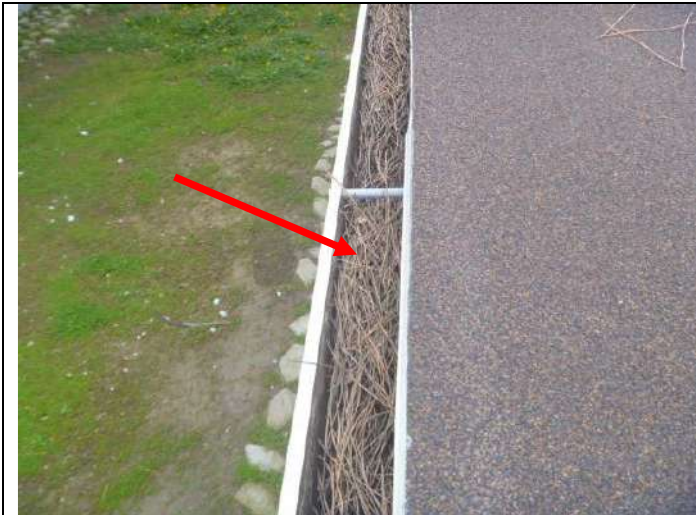
Gutter in need of cleaning.
