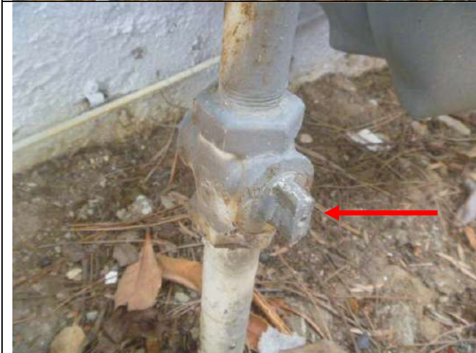
Gas shut off valve.
