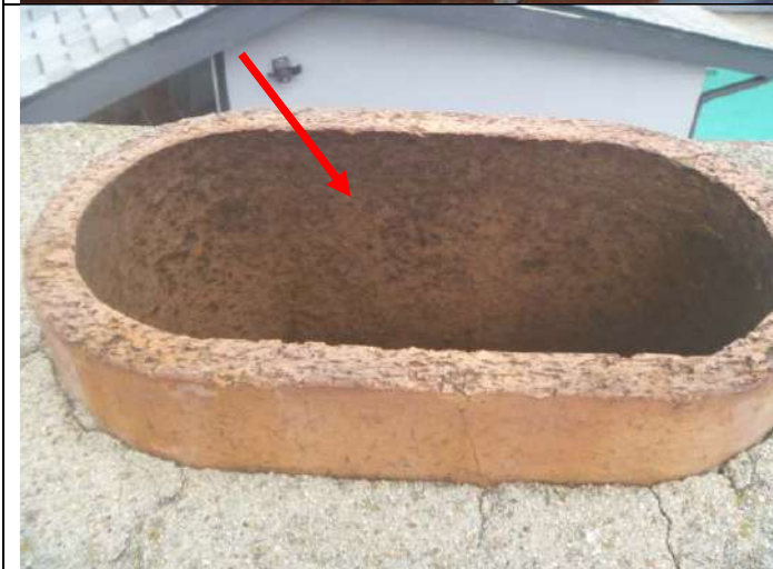
No spark arrestor/rain cap on top of the chimney.
