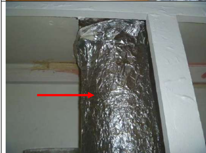
Foil on the range hood vent fan duct within the above cabinet.
