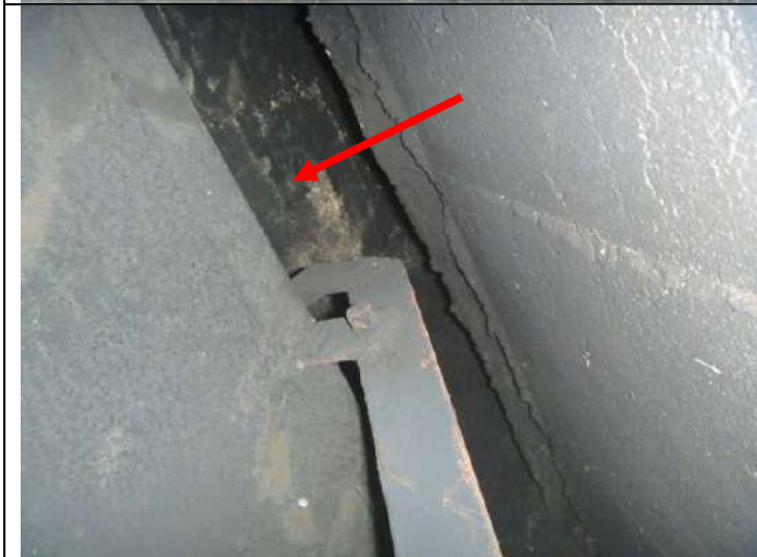
Fireplace damper stuck in the open position.
