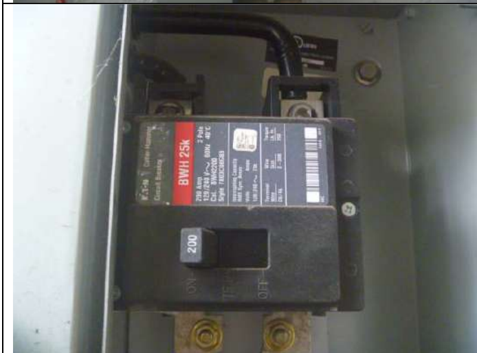
A closer view of the main breaker.
