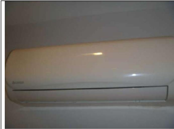
Air handler in the ADU bedroom.
