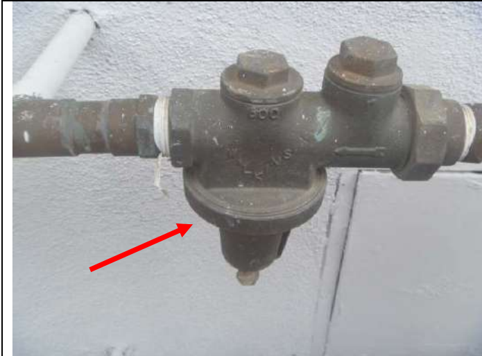
Primary water pressure regulator. See PLUMBING section for related comments.
