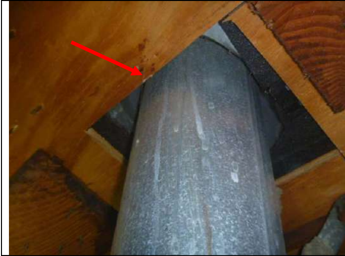
Heater vent pipe without the proper 1" clearance at the roof sheathing.
