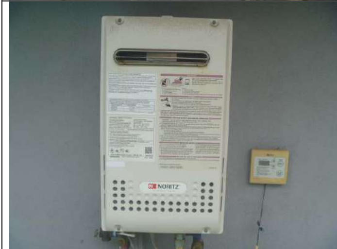
ADU tankless water heater.
