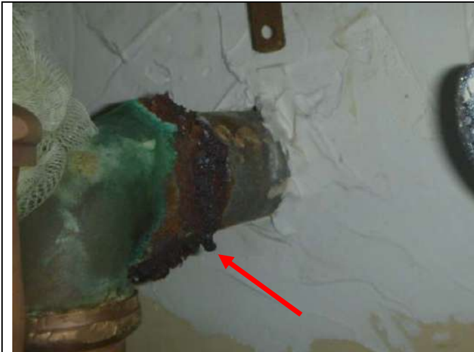
Rusted drain piping below the full bathroom sink.
