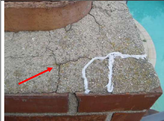
Chimney crown cracking.
