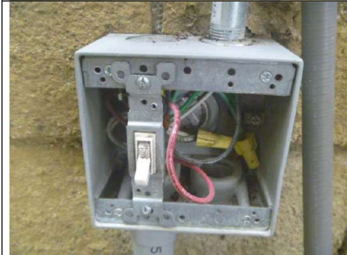
Open electrical box at the pool equipment.
