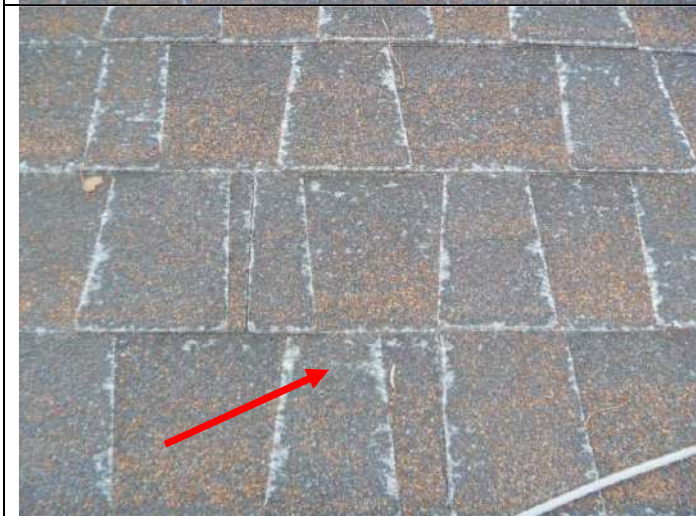
Shingle close-up of a more noticeably deteriorated area.
