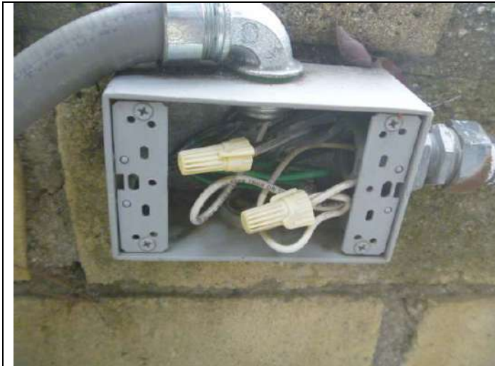
Open electrical box at the pool equipment.
