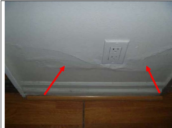
Wall damage at the lower left of the rear bedroom entry door.
