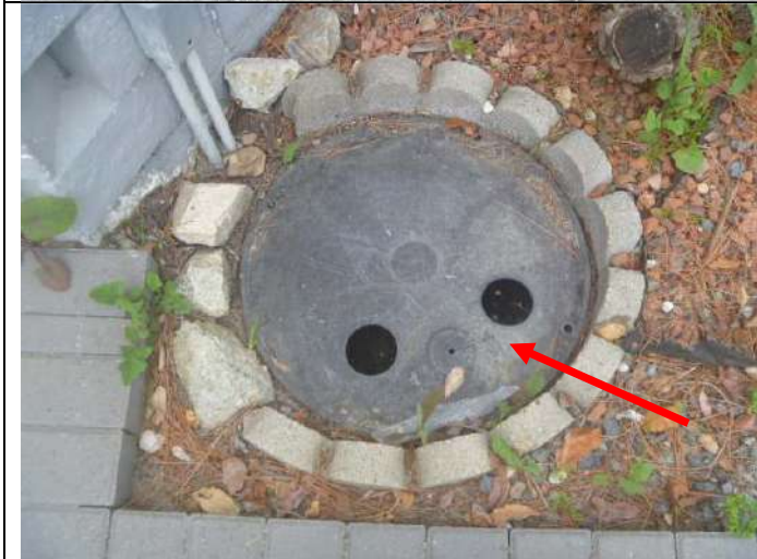
Exterior drain sump pump location.
