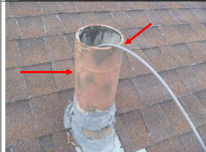
Missing cap for an original transite vent pipe (not in use). Note: The cable routed through the vent pipe.
