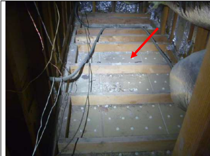
Missing attic insulation.
