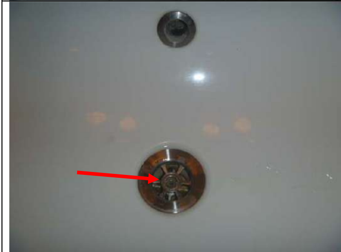
3/4 bathroom sink with missing sink stopper (screw-in type).
