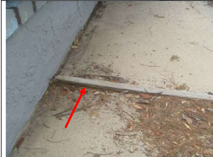
Pool deck lifted spacer.
