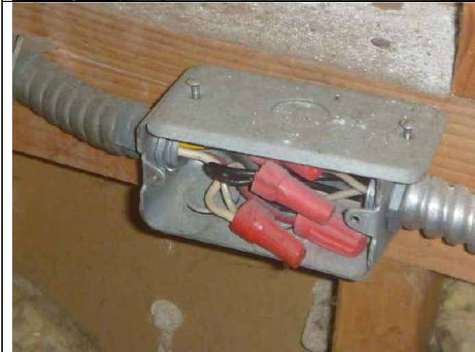
Open electrical box in the attic.
