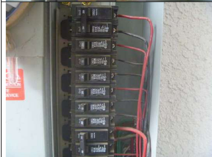
A closer view of the upper breakers.
