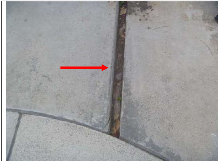
Pool deck missing spacer.
