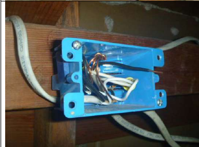
Open electrical box in the attic.
