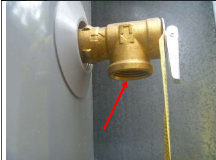
Water heater pressure relief valve without a drain pipe.
