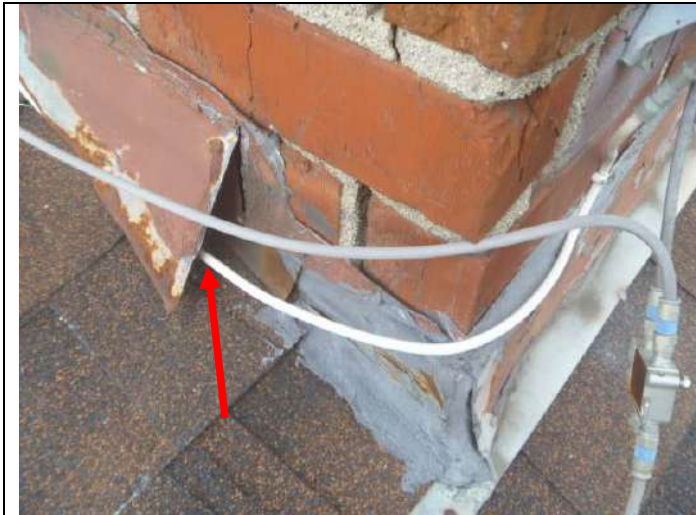
Separated flashing at the chimney.
