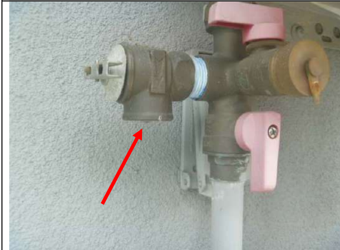
No drain pipe for the pressure relief valve below the water heater.
