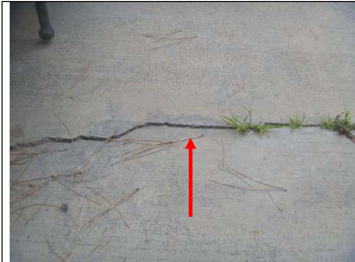
Rear patio cracking.
