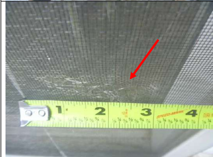
A torn window screen (off the rear bedroom).
