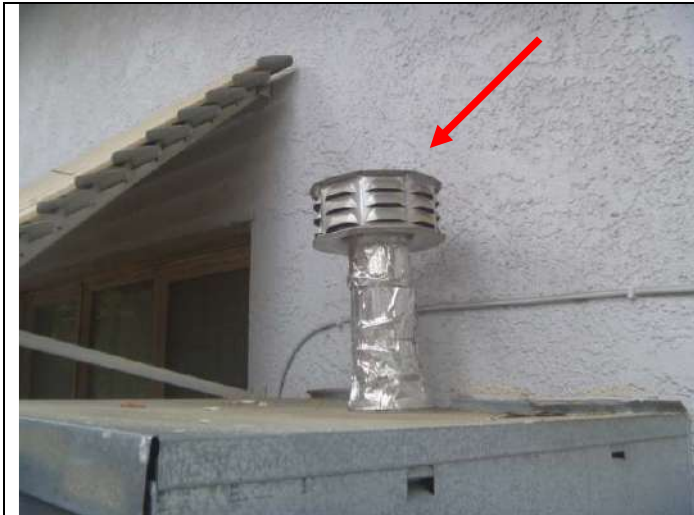
Water heater vent pipe terminating immediately above the compartment.
