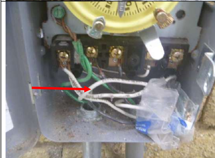
Missing insulating cover below the pool timer switch.
