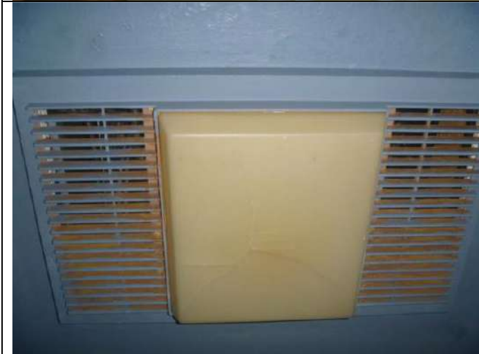
Full bathroom light/heater/fan. Note: The cracked light fixture cover.
