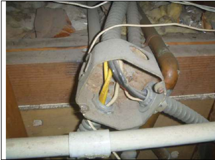
Open electrical box in the attic.
