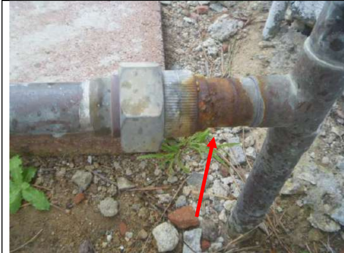
Rusted water piping joint at the front exterior.
