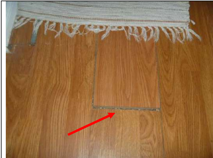
Gap in the hallway flooring.
