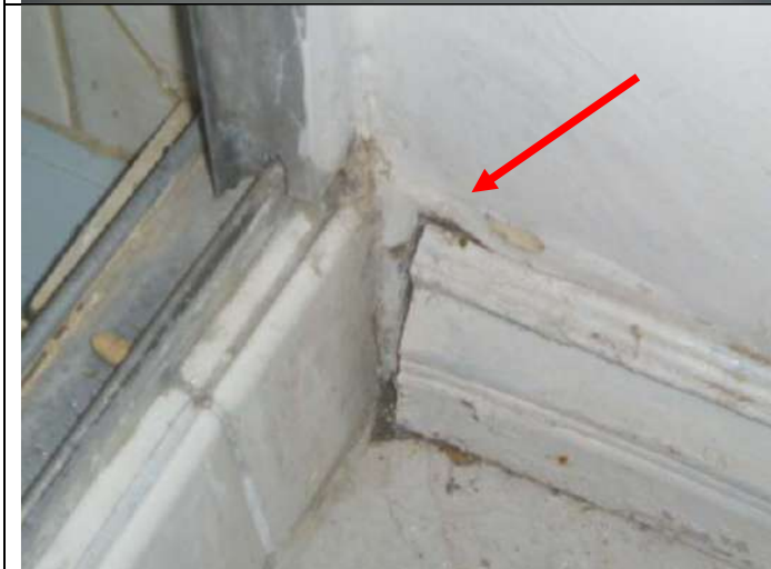
Wall damage at the lower right of the 3/4 bathroom shower.
