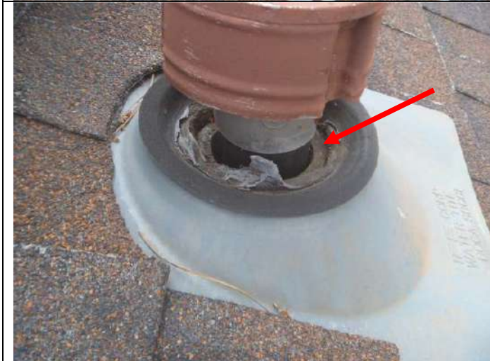
Damaged and inverted plumbing vent collar (neoprene type).
