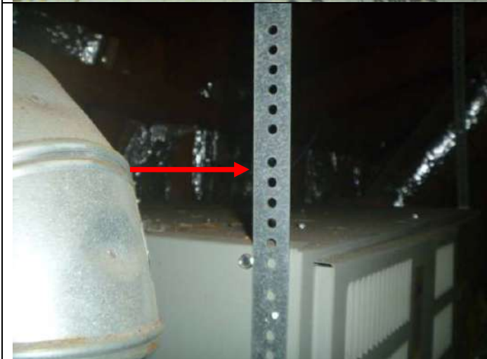
Heater/fan unit hanging from plumber's tape.
