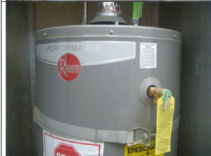
Water heater upper section.
