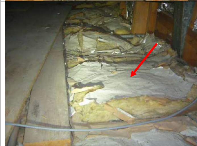
Older attic insulation installed upside down.
