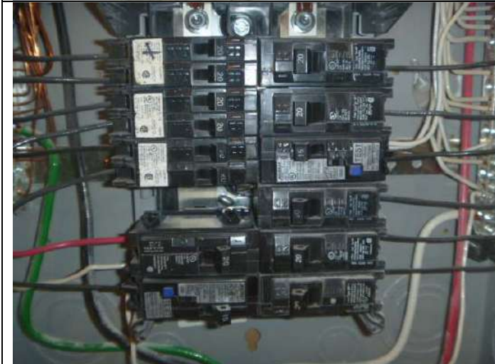
A closer view of the breakers.
