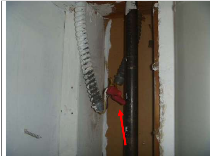
Opening in the wall within the cabinet above the range hood. Note: The exposed wiring splices.
