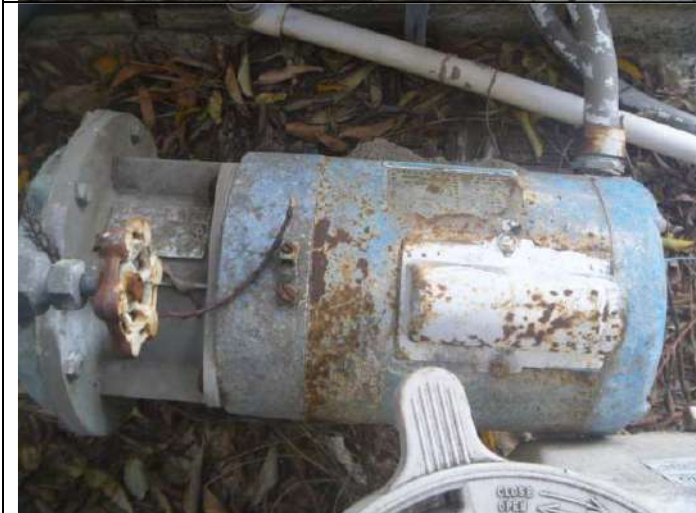
Pool sweep pump (inoperative and not in use).
