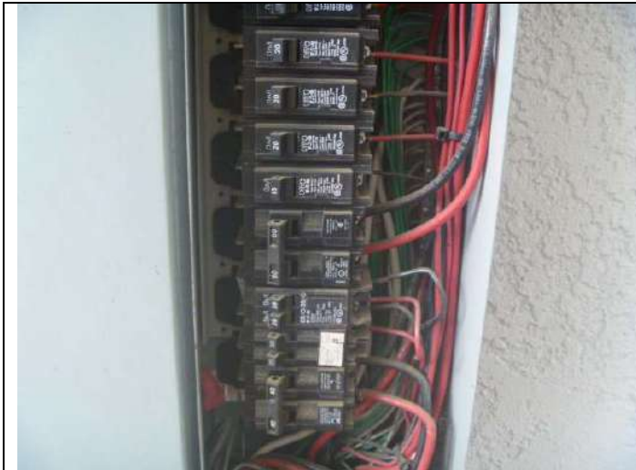
A closer view of the lower breakers.
