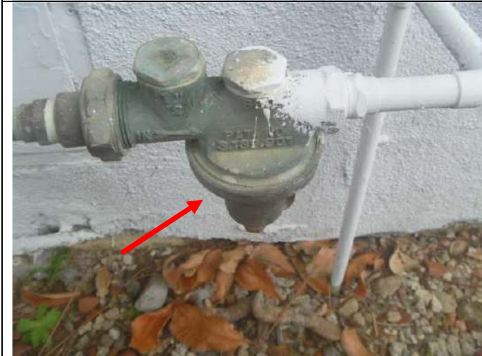
Second water pressure regulator (for irrigation piping). See PLUMBING section for related comments.
