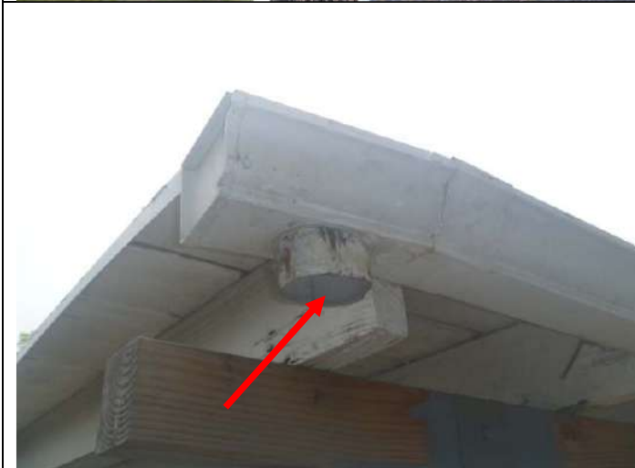
Missing downspout at the right rear.
