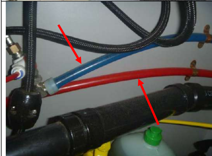
PEX water piping below the ADU kitchen sink.
