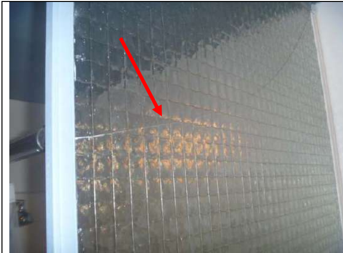
Cracked shower/tub enclosure pane.
