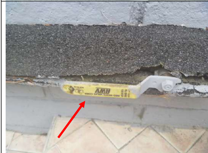
ADU main water valve.
