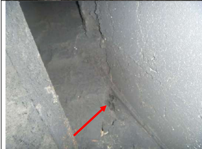
Gap at the fireplace upper interior.
