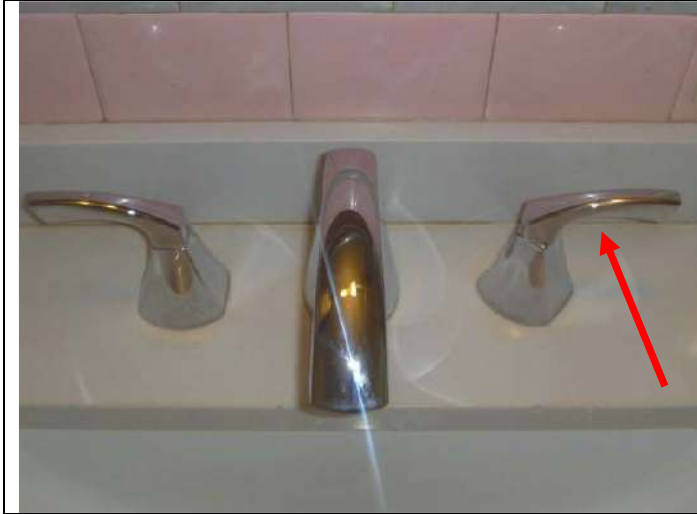
Full bathroom sink faucets. Note: The cold water valve is stiff.
