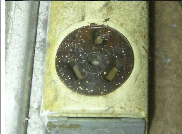
240 volt receptacle for an electric dryer.
