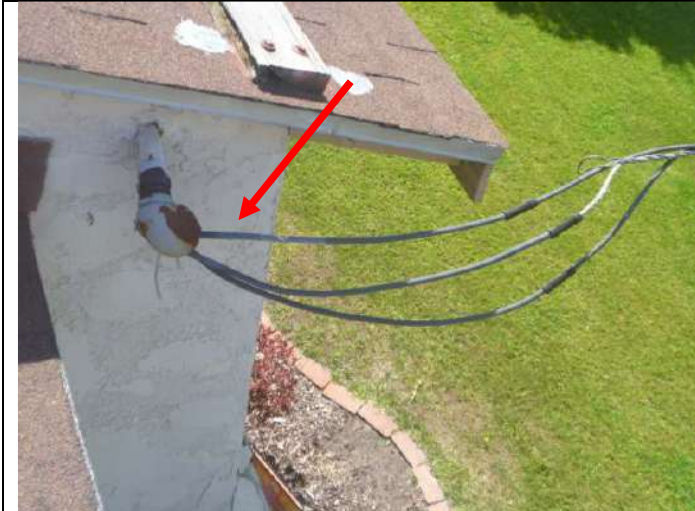
Older electrical service entrance (with disconnected tension relief).
