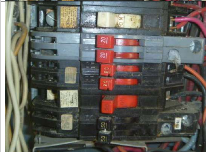
A closer view of the lower breakers.
