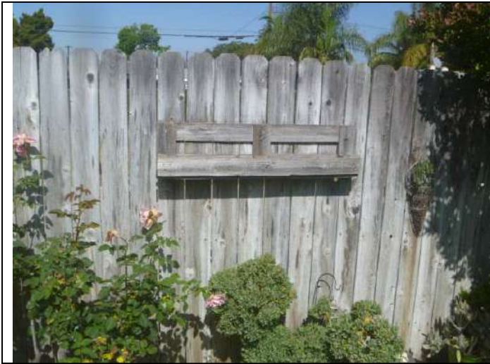
Weathered west side wood fence.
