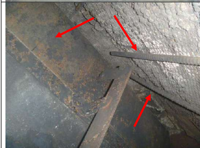
Fireplace damper in the closed position. Note: The exposed rebar at the upper right.
