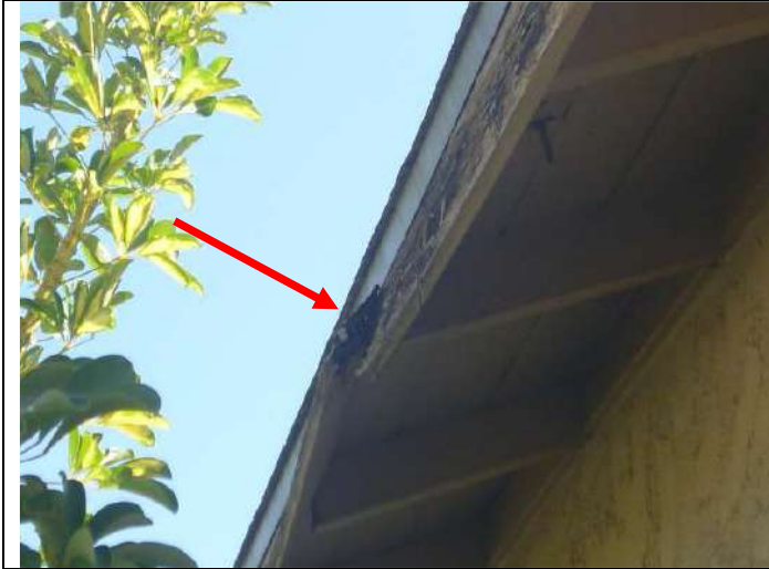
Damaged wood along the west side eave.
