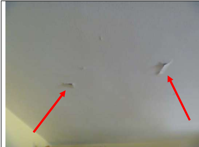
Paint peeling on the living room ceiling.
