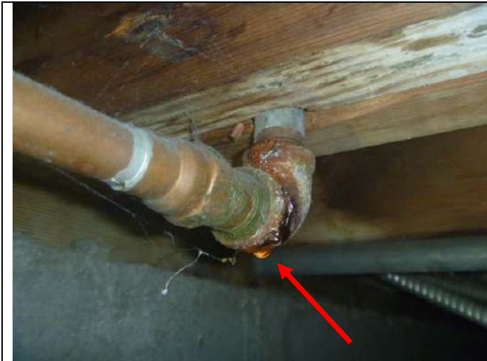
Slowly leaking water pipe in the foundation crawlspace below the laundry room.
