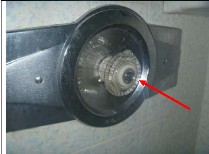
3/4 bathroom shower fixture (pull type). Note: The valve is somewhat stiff (minor).
