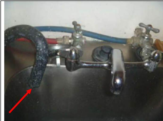
Laundry sink faucet and washer valves. Note: The washer draining into the sink.
