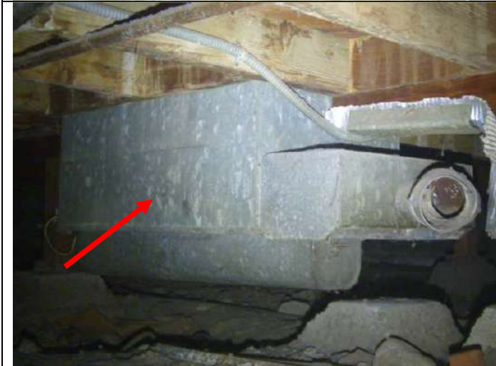
Original gravity floor heater (not in use) in the main foundation crawlspace.
