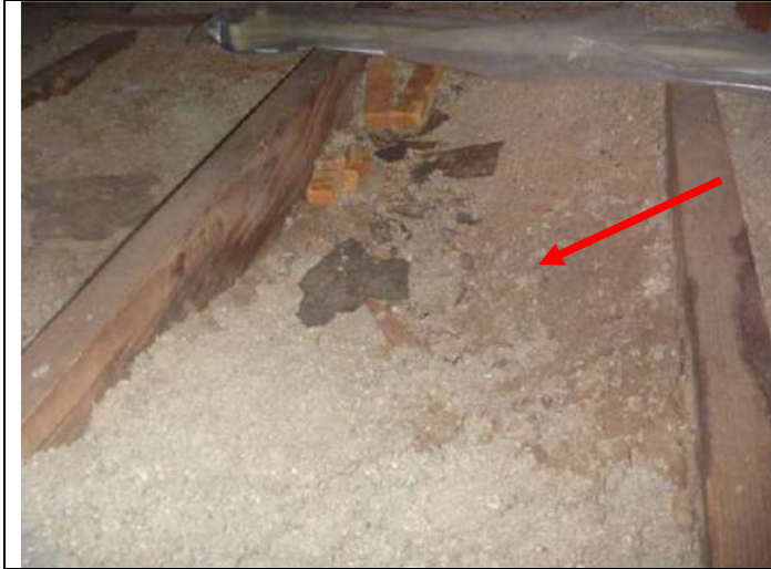
Old and thin attic insulation.
