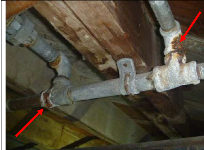
Rusted and corroded galvanized water piping.
