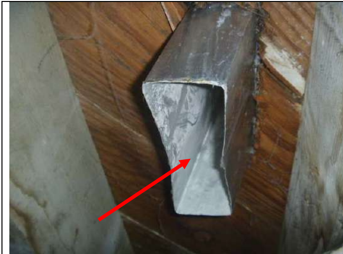
Dryer venting into the foundation crawlspace.
