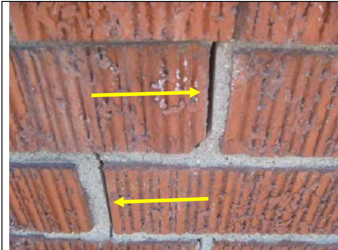
Cracking in the chimney upper exterior.
