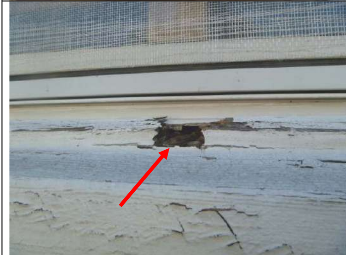
Damaged wood at the west front bedroom west window.
