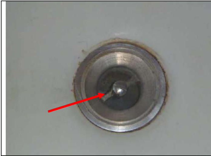
Shower/tub drain without a functional stopper.
