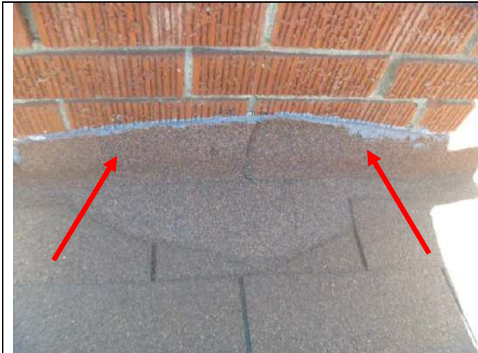
Added rolled composition or similar roofing material at the chimney.
