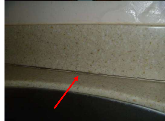
Cracked sealant along the countertop wall splash at the kitchen sink.
