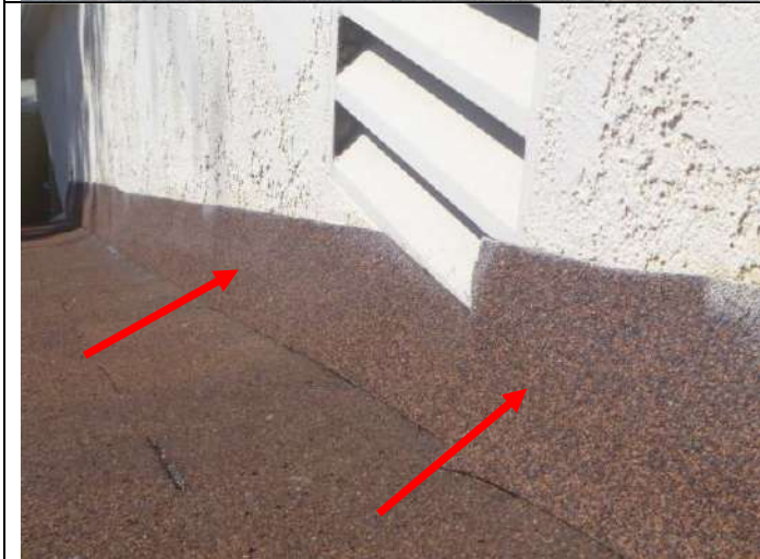
Added rolled composition or similar roofing material at the carport roof/stucco wall connection.
