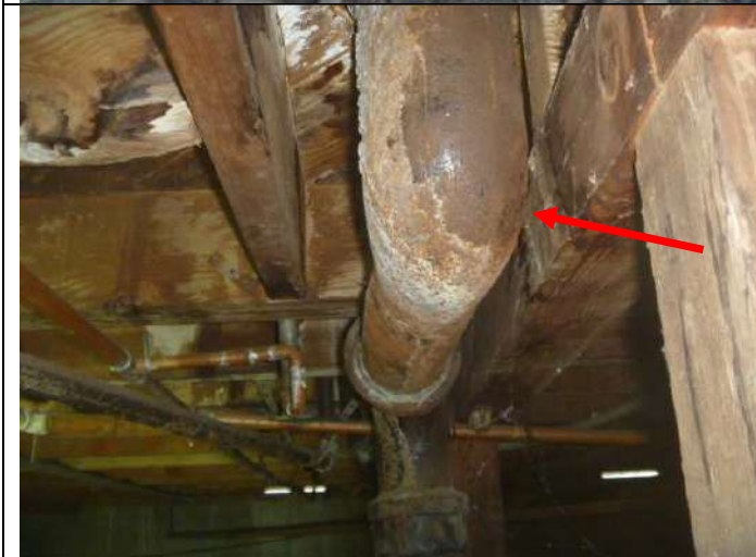
Original cast iron drain piping.
