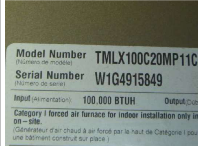
Heater/fan unit model, serial number (indicating a 2014 build date) and capacity.
