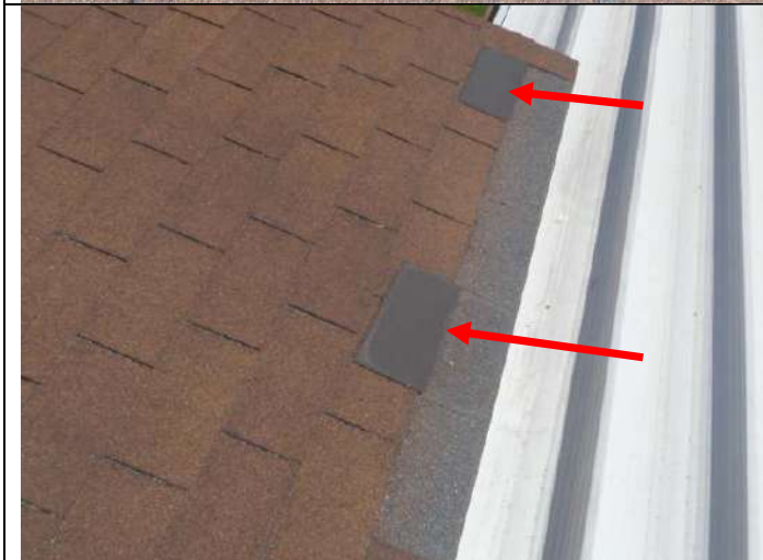
Missing and folded back shingles.
