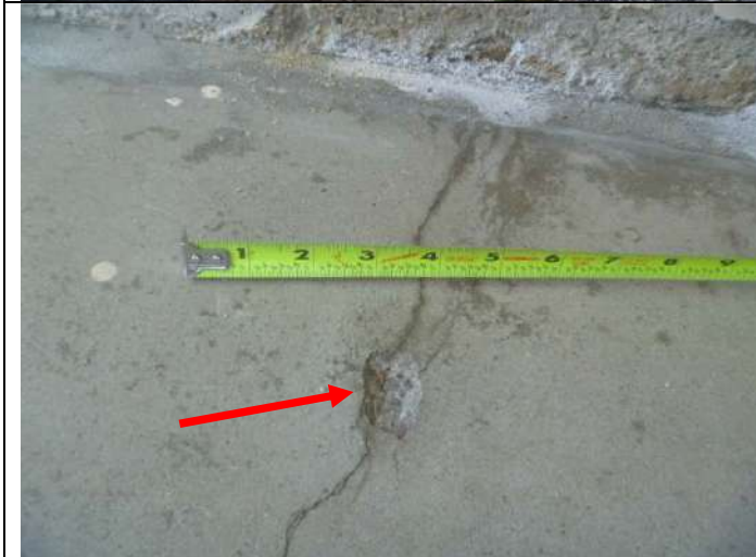
Front porch cracking.
