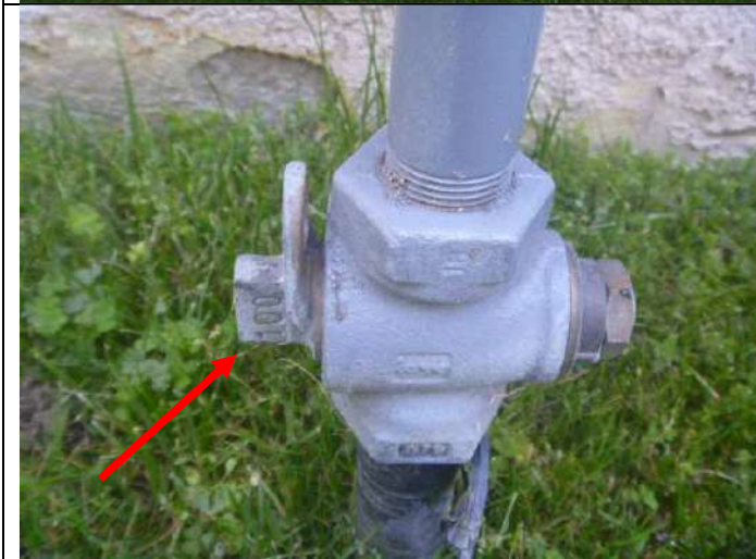
Gas shut off valve.
