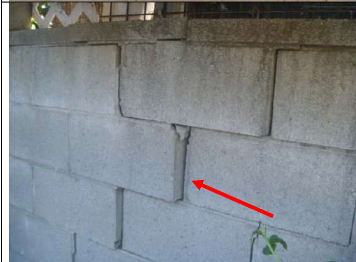
Cracking and displacement in the east block wall.
