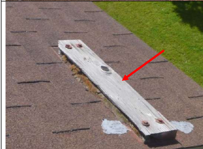
Wooden mount for a previous electrical service entrance.
