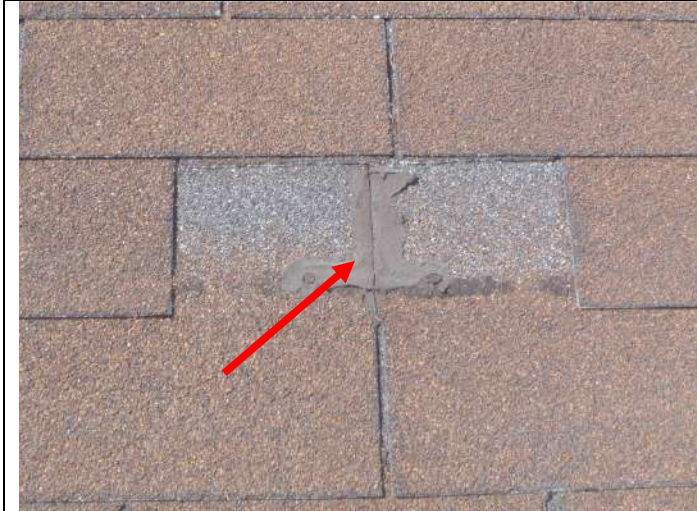
A missing shingle.
