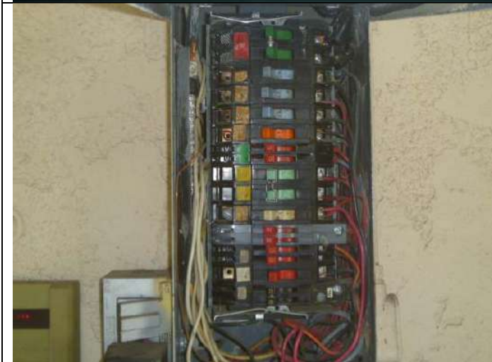
Main electrical panel (with interior cover removed for inspection).
