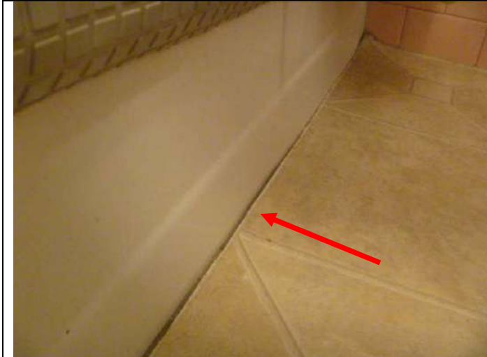
Lifted flooring at the tub.
