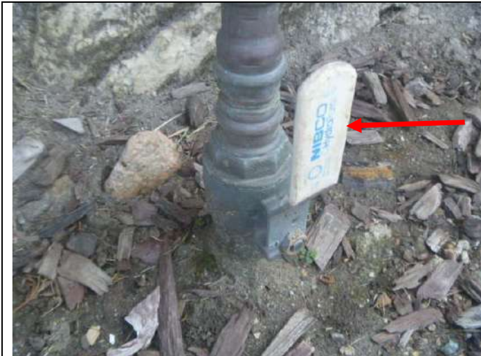
Main gas valve.
