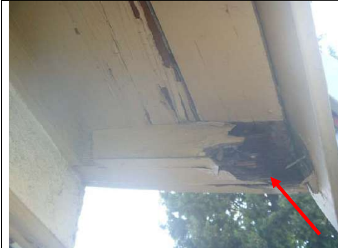
Damaged wood at the right front eave.
