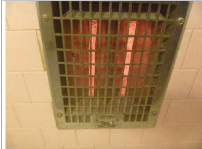
Full bathroom old wall heater (electric).
