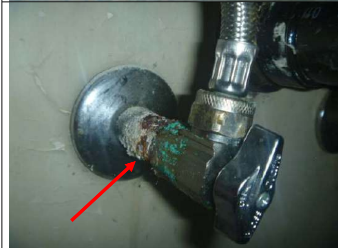
Rusted and corroded water pipe at the hot water shut off valve below the 3/4 bathroom sink.
