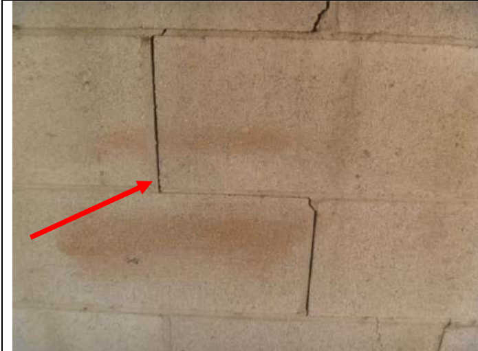
Cracking in the east block wall.
