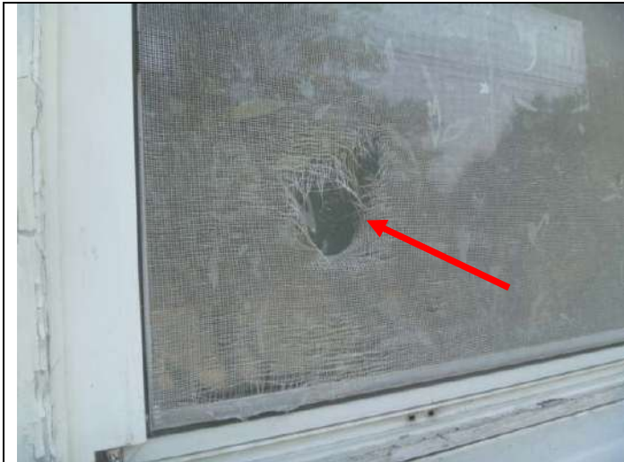
West front bedroom torn front window screen.
