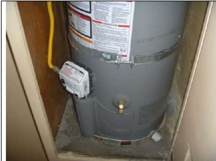
Water heater lower section.
