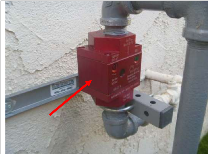
Seismic shut off valve for the gas piping.
