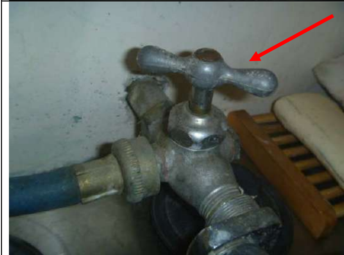
Washer cold water valve (which is stuck or stiff).
