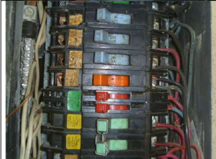
A closer view of the upper breakers.
