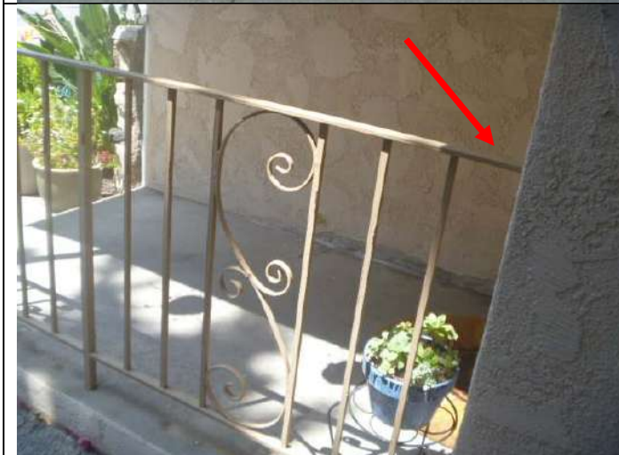
Front porch railing which is loose at the wall.
