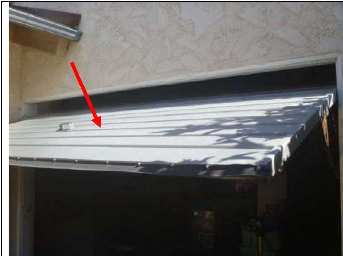
Garage door not staying in the completely open position.
