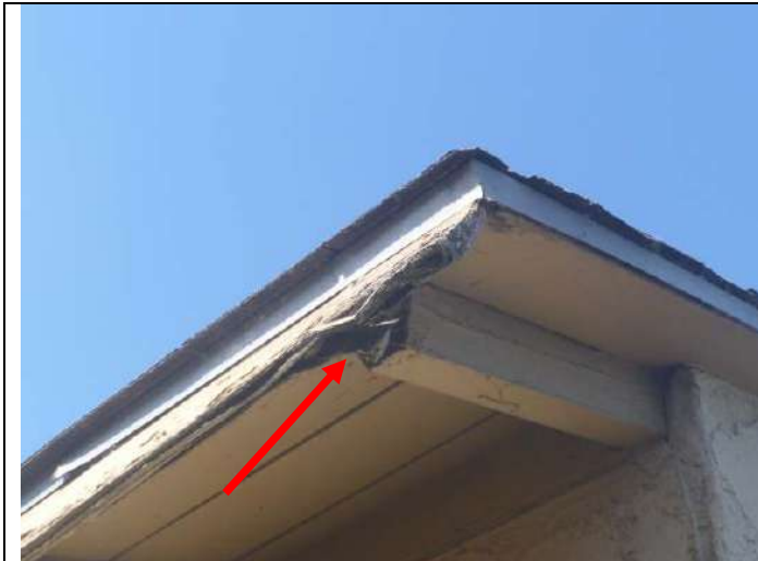
Damaged wood at the garage right rear eave.
