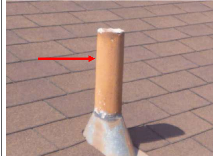
Main plumbing vent pipe (transite type).
