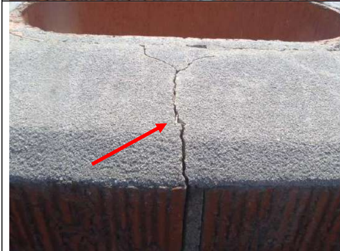
Cracking in the chimney mortar crown.
