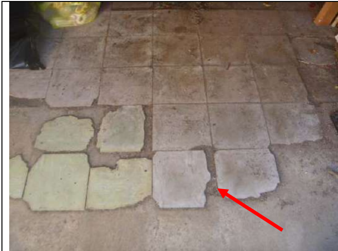
Old and damaged vinyl flooring tiles (with likely asbestos content) in the garage.
