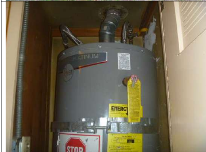
Water heater upper section.
