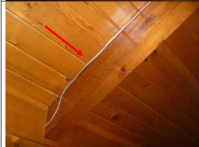
Unprotected nonmetallic cable (Romex) wiring to the family room ceiling light/fan.
