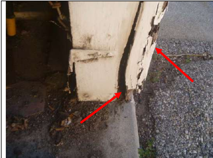
Damaged wood at the base of the garage doorjamb.
