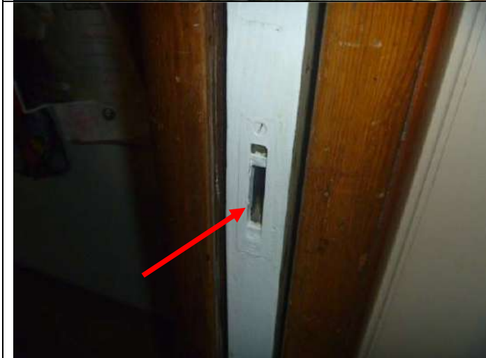
Broken off pull handle for the kitchen pocket door to the laundry room. Note: This door and the door to the living room are off track.
