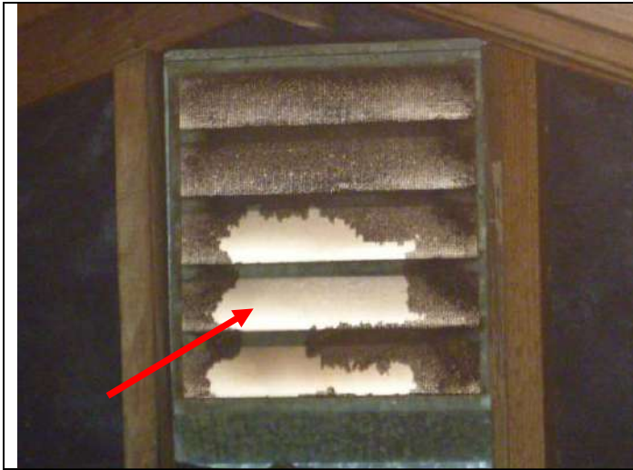
Attic torn east gable vent screen.
