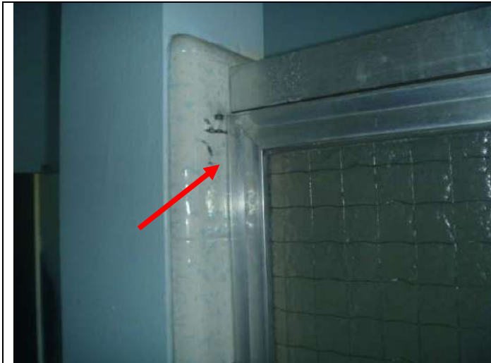
3/4 bathroom shower door rubbing along the wall.
