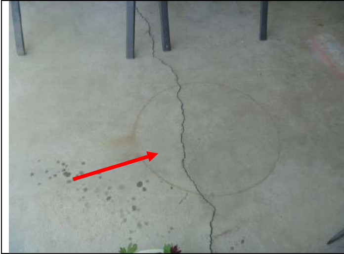
Main rear patio cracking.
