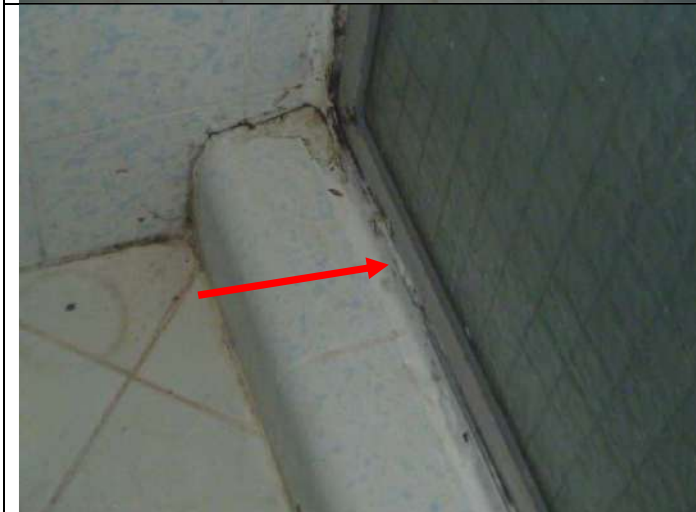
Sealant at the base of the 3/4 bathroom shower enclosure.
