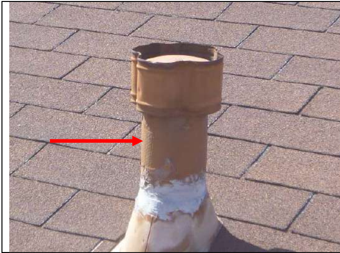
Water heater vent pipe (transite type).
