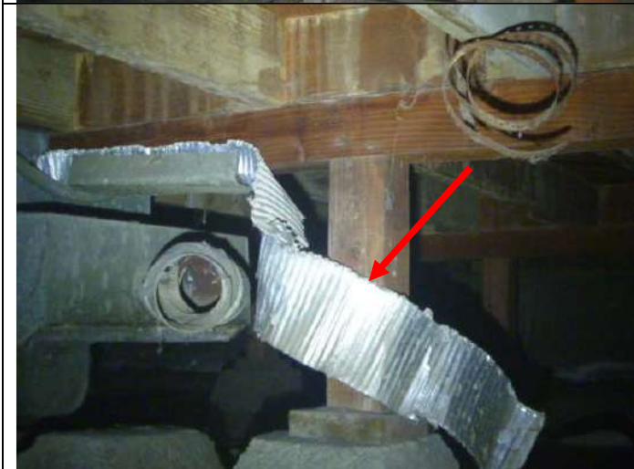
Asbestos insulation at the above noted original gravity heater.
