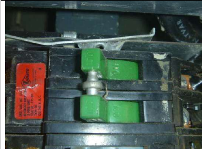
A closer view of the main breaker.
