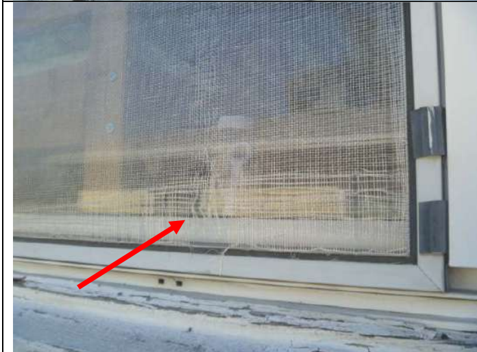
West front bedroom torn side window screen.
