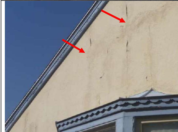
Example of stucco cracking, damage and repair related irregularities.
