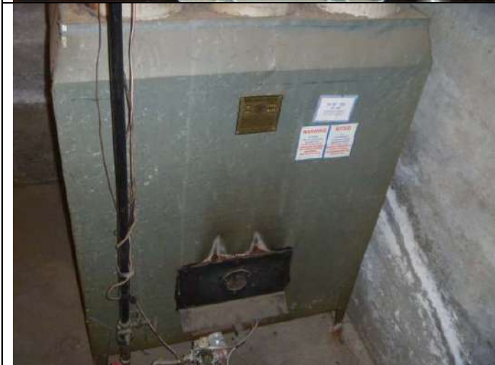
Central gravity heater.
