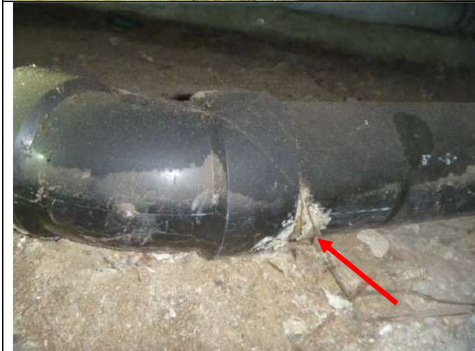
Leaking drain pipe joint at the right front of the basement area.
