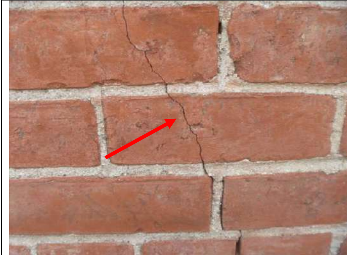
Chimney exterior cracking.
