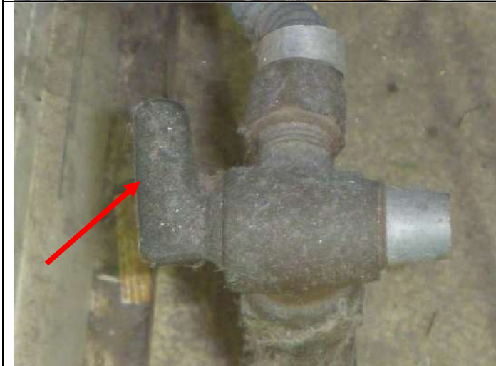
Older gas valve for the dryer.
