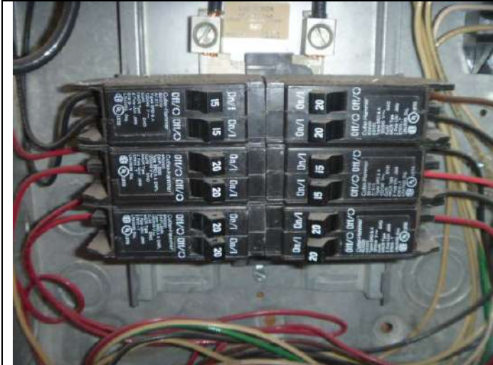
A closer view of the breakers.
