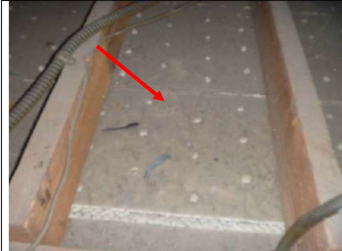
No attic insulation.
