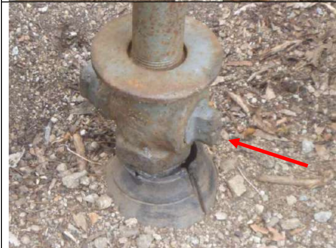
Gas shut off valve.
