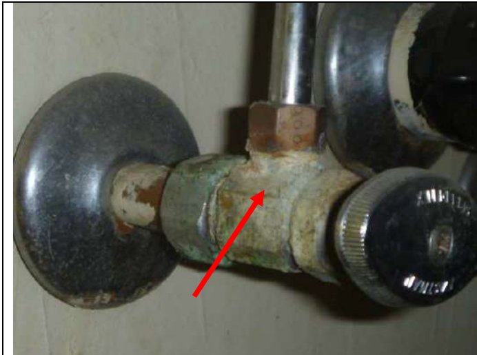
Corrosion on the hot water shut off valve below the rear bathroom right sink.
