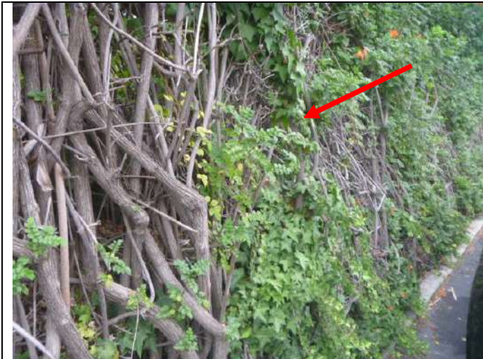
Leaning left side chain link fencing obstructed by vegetation.
