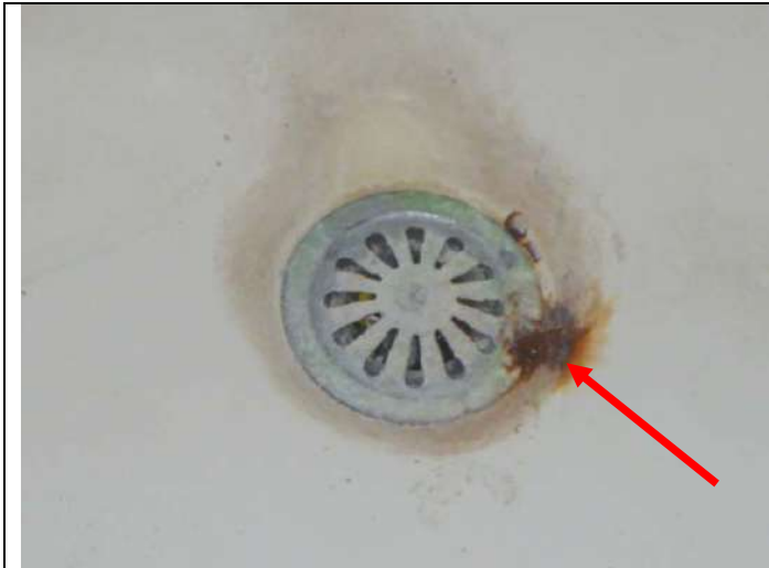
Front bathroom tub rust.
