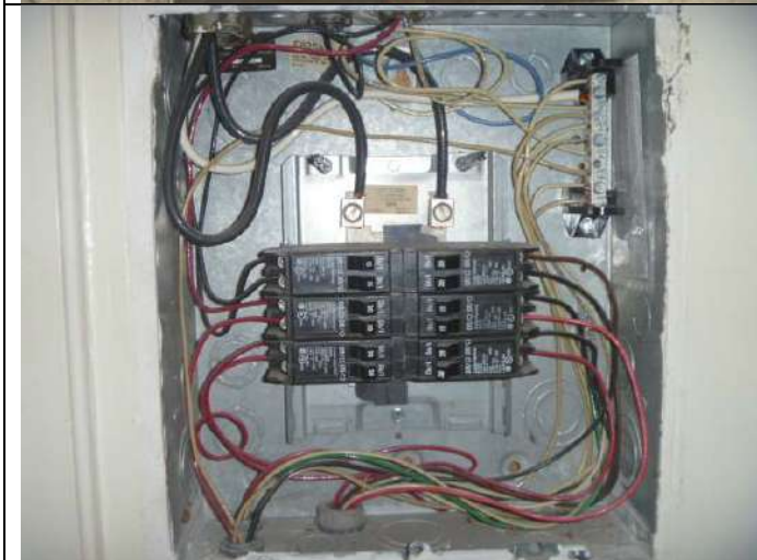
Primary subpanel (with cover removed for inspection).
