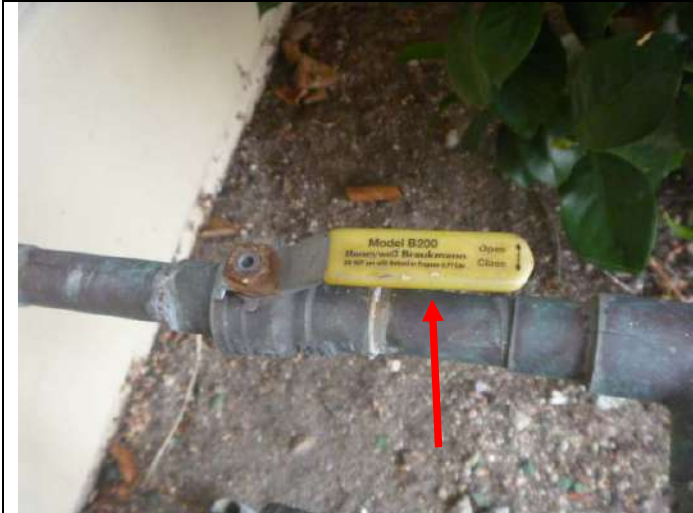
Main water valve.
