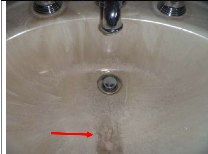
Discoloration in the rear bathroom right sink.
