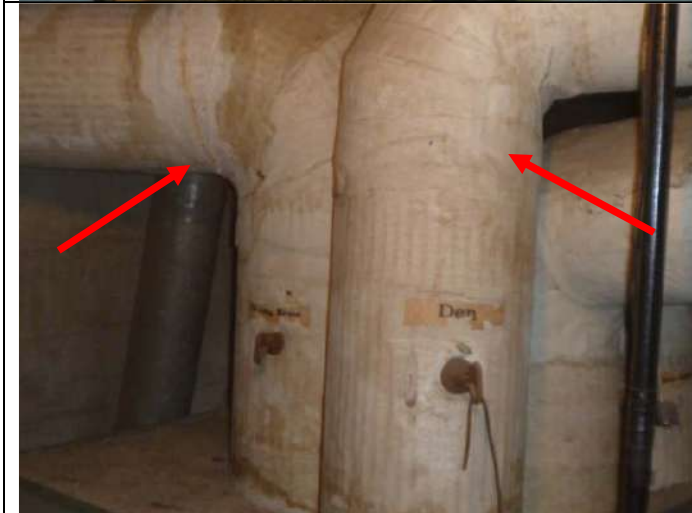
Asbestos insulated ductwork.
