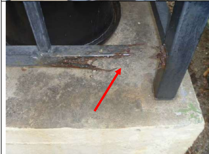
Rusted out wrought iron railing at the front porch.
