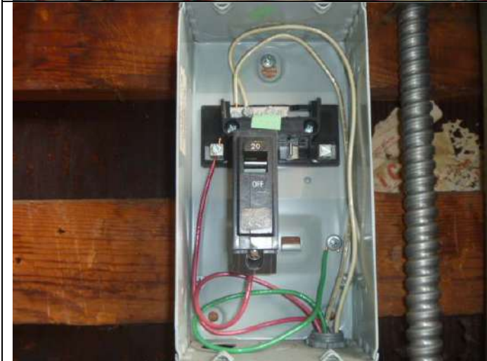
Subpanel (with cover removed for inspection) in the garage. Note: The panel is wired for only 120 volts (vs. 120/240 volts).
