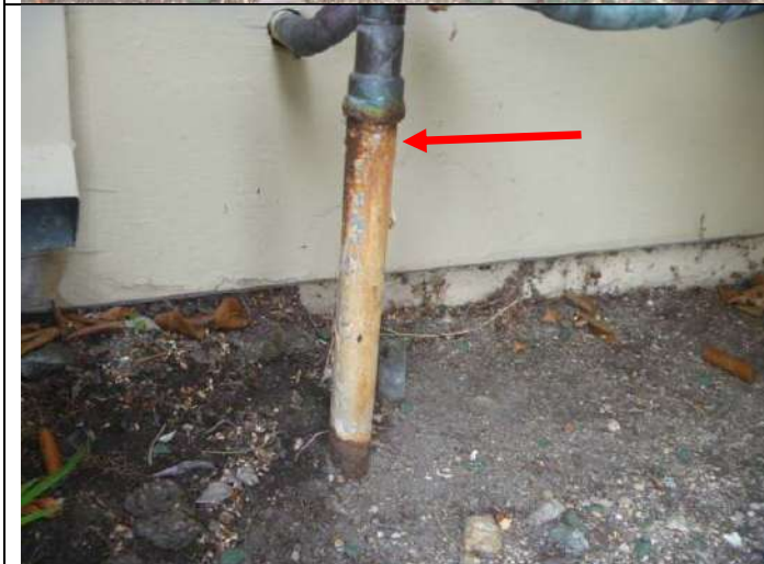
Rusted irrigation system piping at the front exterior.
