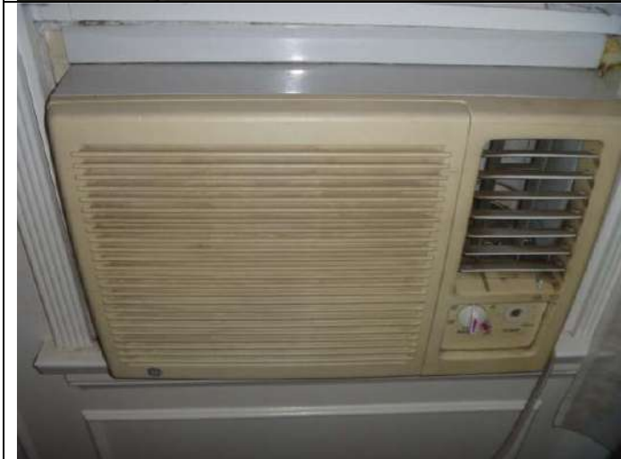
Dining room air conditioner.
