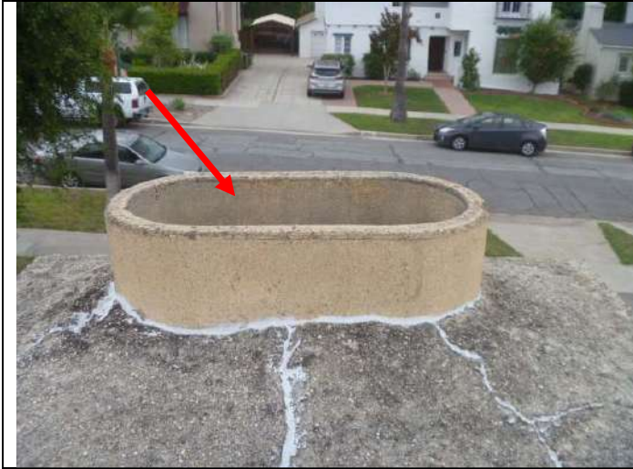
No spark arrestor/rain cap.
