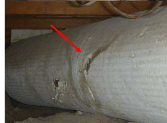
Asbestos insulated ductwork.
