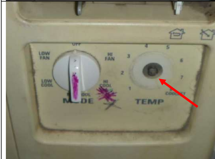
Dining room air conditioner controls with missing temperature adjustment dial.
