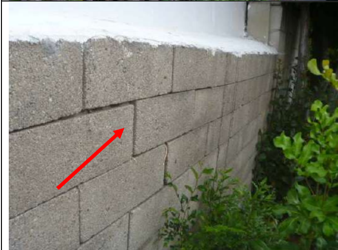
Cracked and leaning far rear block wall.
