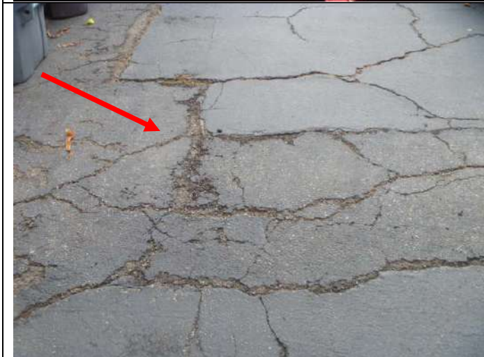
Old and cracked asphalt driveway.
