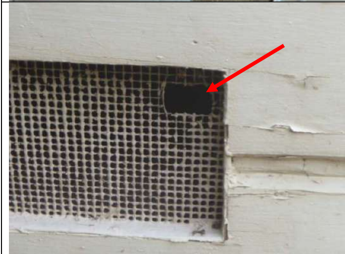
Damaged foundation vent screen.
