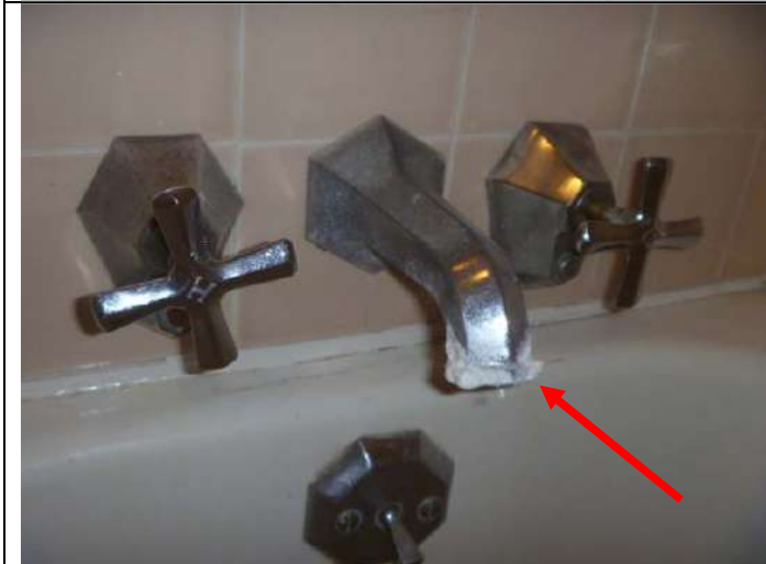
Front bathroom tub fixtures. Note: The corrosion on the tub spout.
