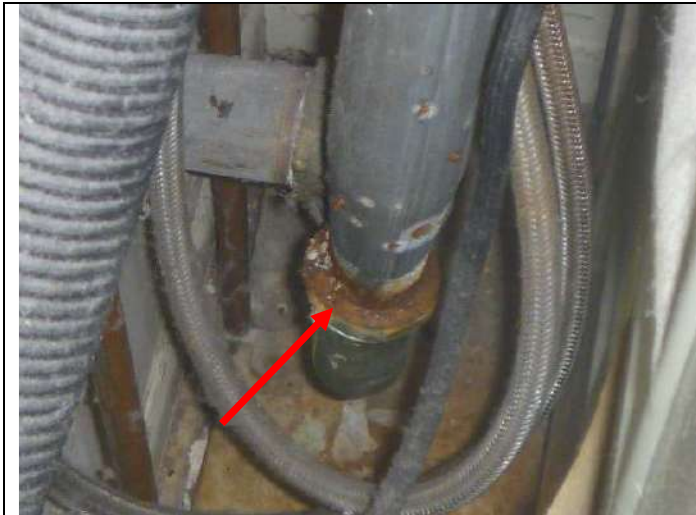
Rusted and corroded washer drain standpipe.
