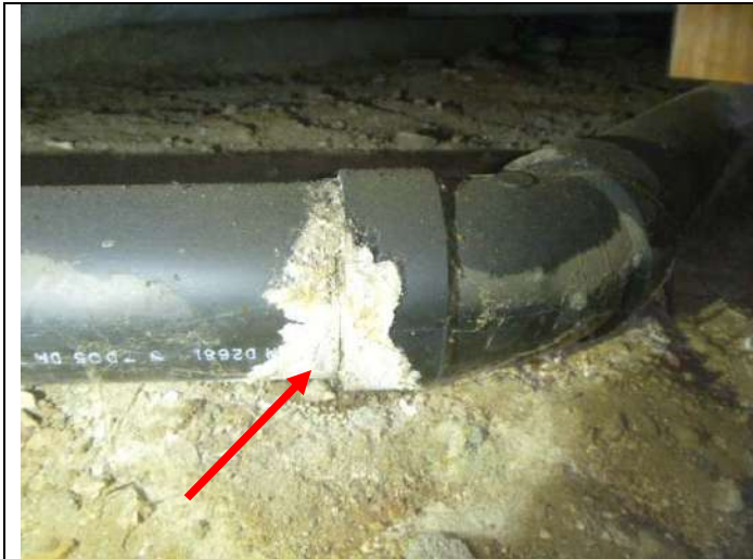
Leaking drain pipe joint at the right front of the basement area.
