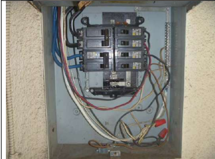
Main service panel (with interior cover removed for inspection).
