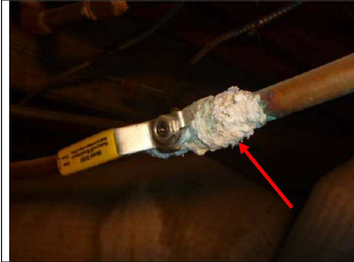
Corroded water valve at the upper right of the water heater.
