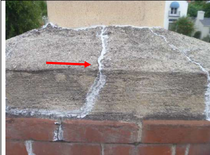
Cracks in the chimney crown.
