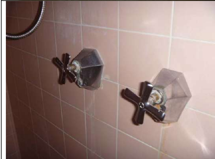
3/4 bathroom shower fixtures.
