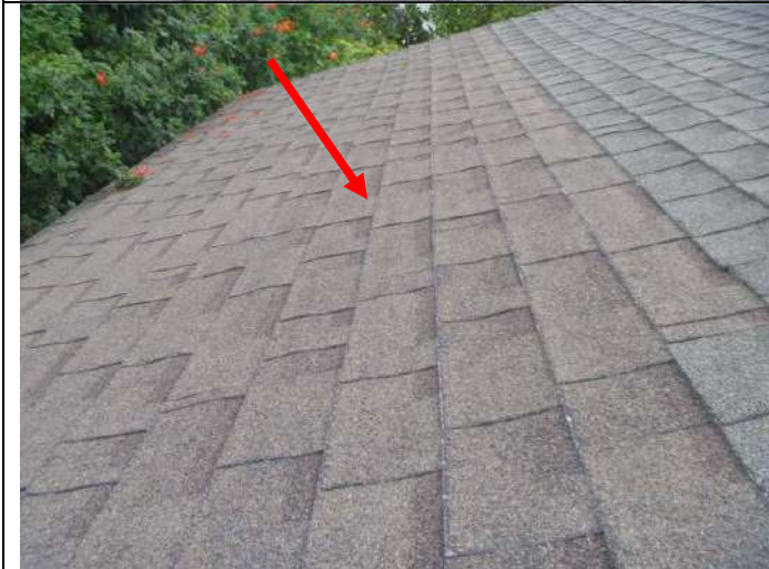
Garage roof older shingles.
