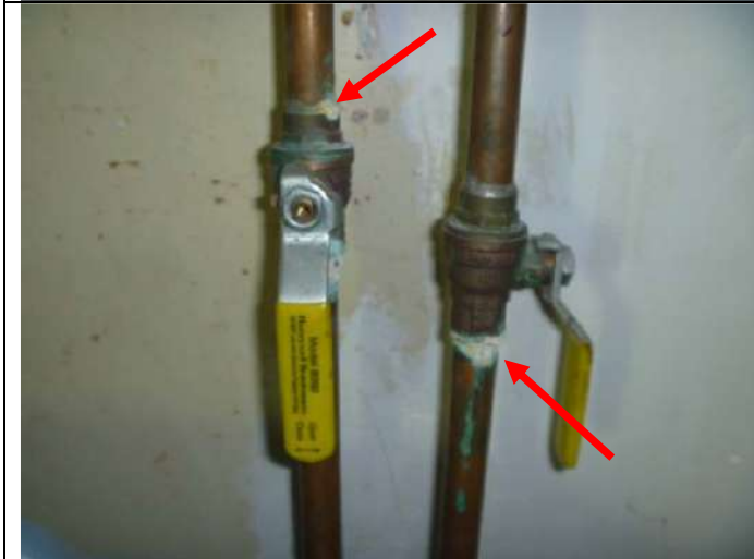
Surface mounted water piping below the kitchen sink. Note: The corrosion on the piping.
