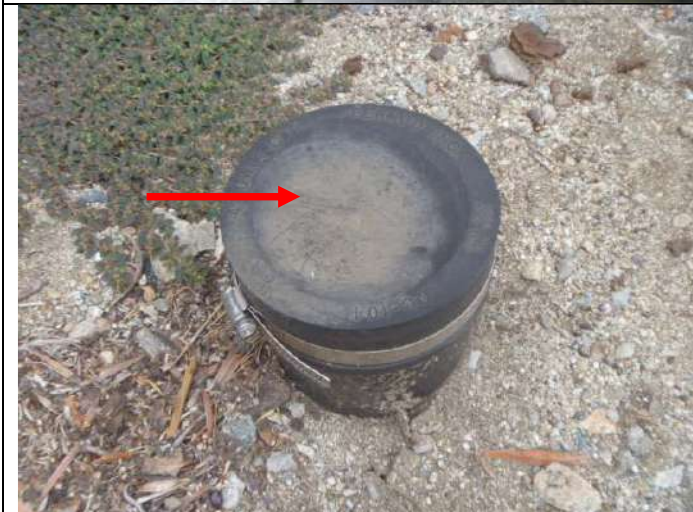
Main drain cleanout at the left side exterior.
