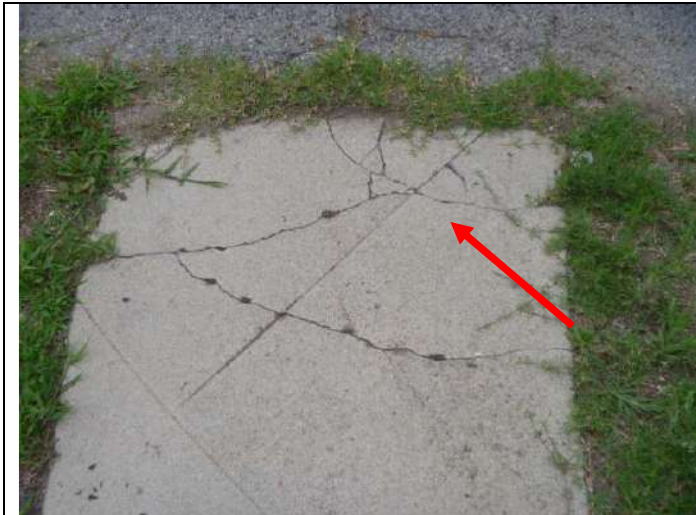
Front walkway cracking.
