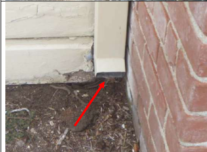
Downspout terminating immediately adjacent to the chimney.
