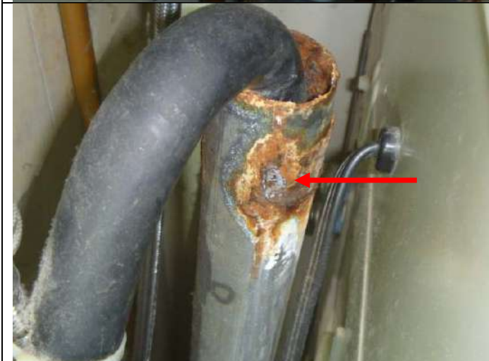
Rusted and corroded washer drain standpipe.
