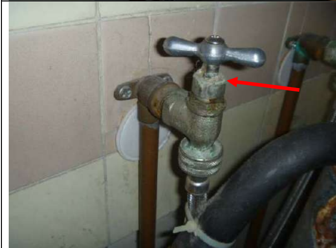
Older washer hot water valve. Note: The surface mounted water piping.
