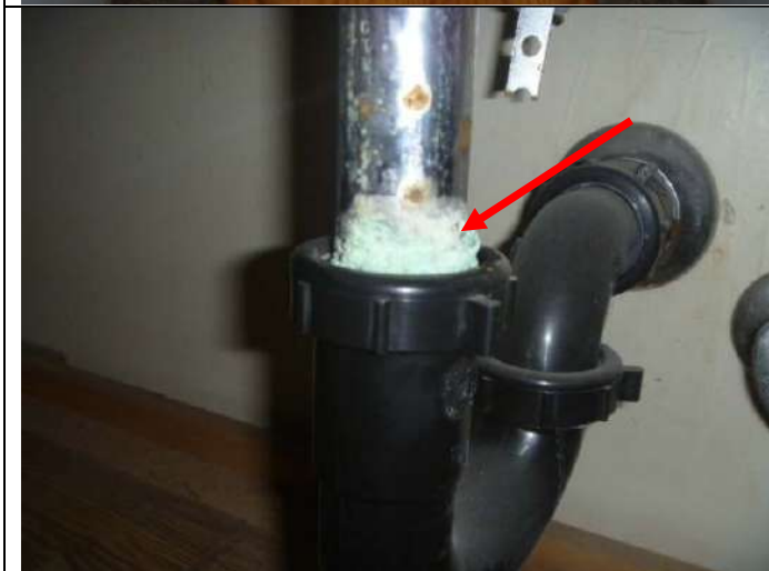
Corrosion on the drain piping below the rear bathroom right sink.
