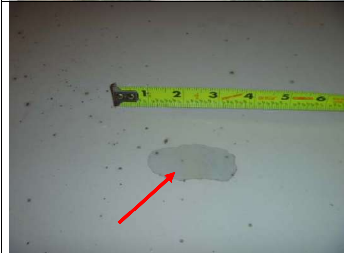
Front bathroom tub surface peeling.
