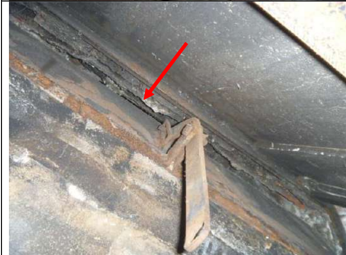
Fireplace damper stuck in a midway position (not forced).
