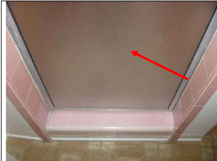
3/4 bathroom shower door. Note: The door did not appear to be a tempered glass type (impact hazard).
