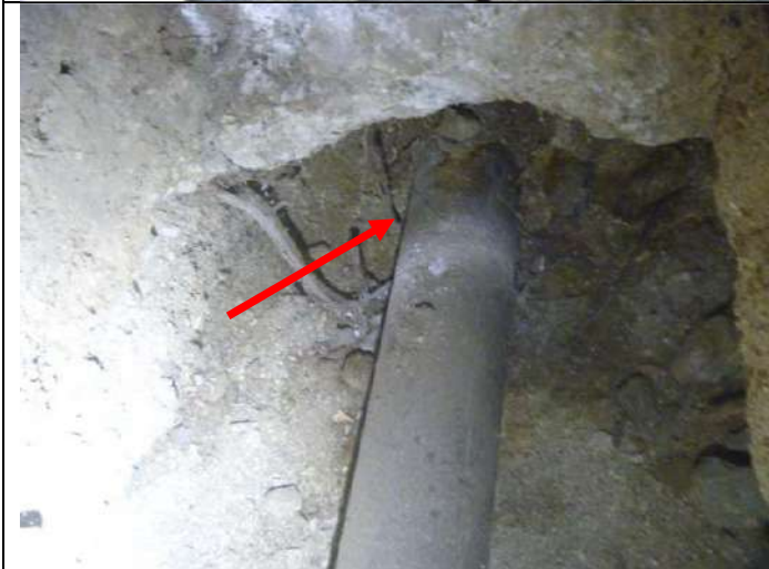
Main drain piping exiting the left side of the main foundation crawlspace.
