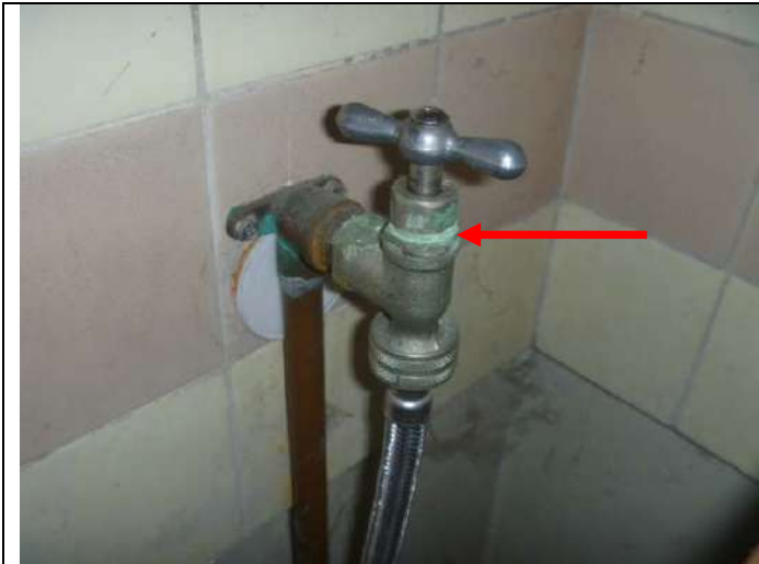
Older washer cold water valve. Note: The surface mounted water piping.
