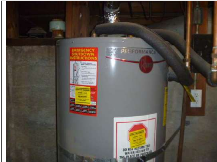
Water heater upper section.
