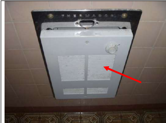
Heater installed over an older heater in the front bathroom.
