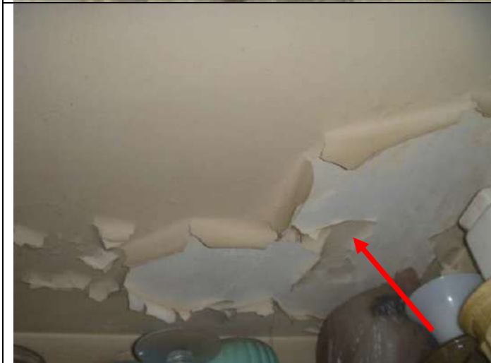
Paint peeling on the laundry area ceiling.
