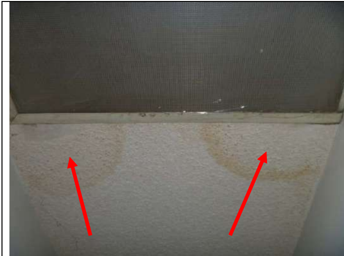
Moisture related discoloration (from previous roof leakage) in the third bedroom closet ceiling.
