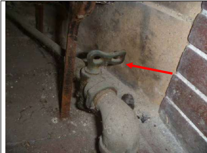
Old gas valve at the right front interior of the fireplace (vs. outside the hearth extension).
