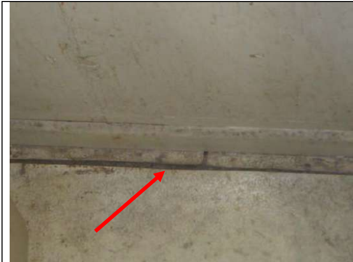
Laundry area old and damaged vinyl flooring.
