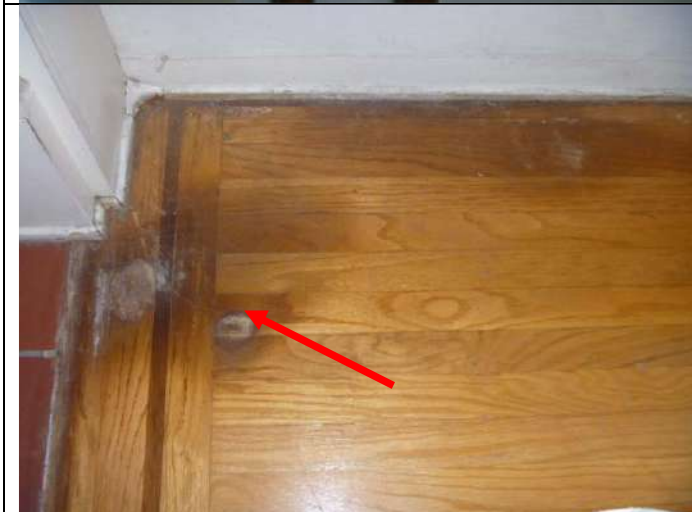
Living room hardwood flooring discoloration.
