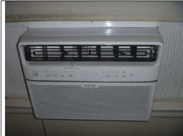
Living room air conditioner.
