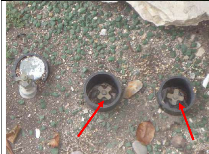
Old front sprinkler valves without anti-siphon valves.
