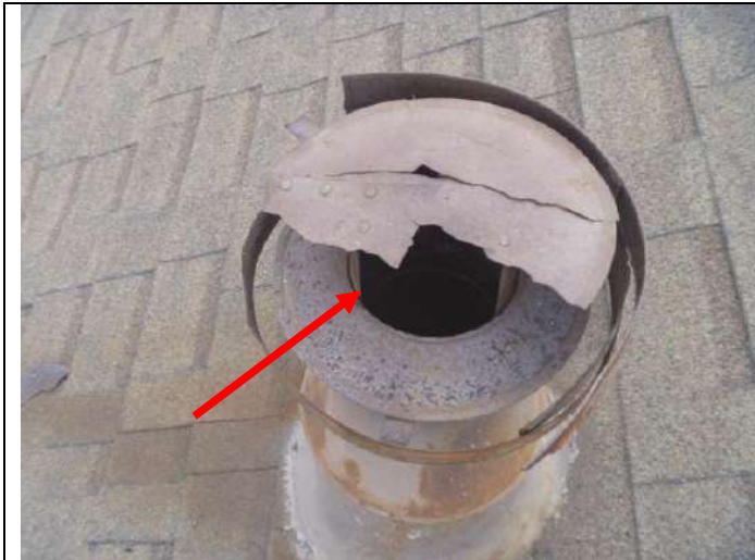
Rusted out vent cap (for the central gravity heater vent pipe).
