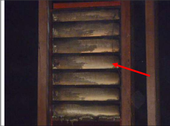
Attic torn gable vent screen.
