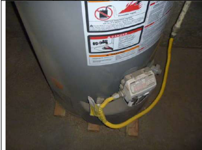
Water heater lower section.
