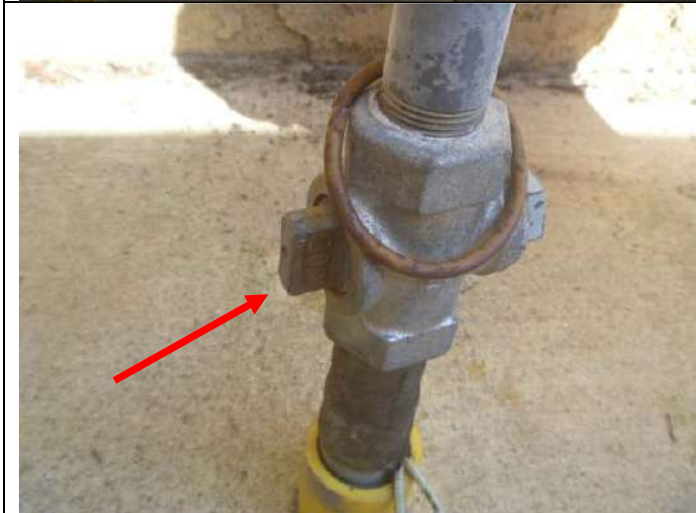
Gas shut off valve.
