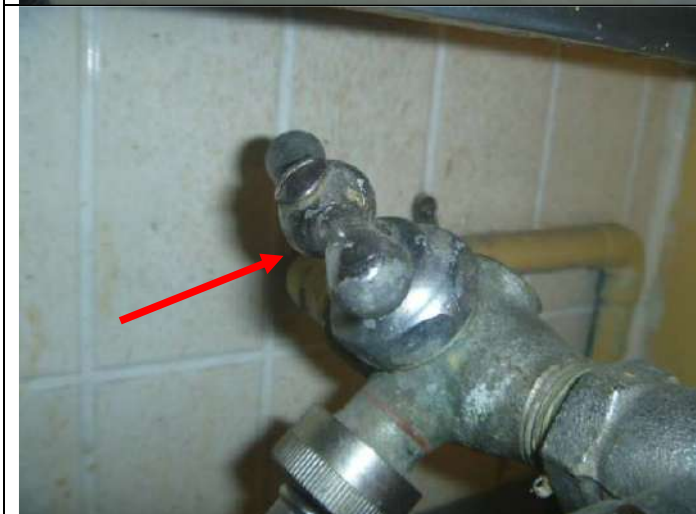
Washer cold water valve.
