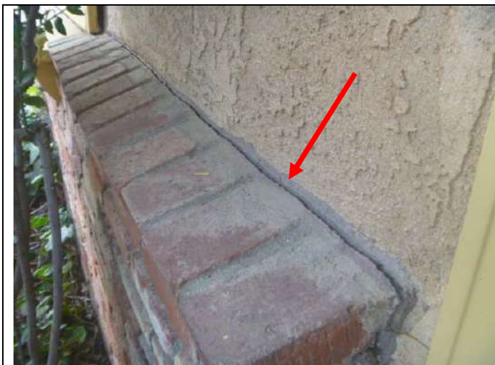
Gap along the top of the brick wall to the left of the front porch.
