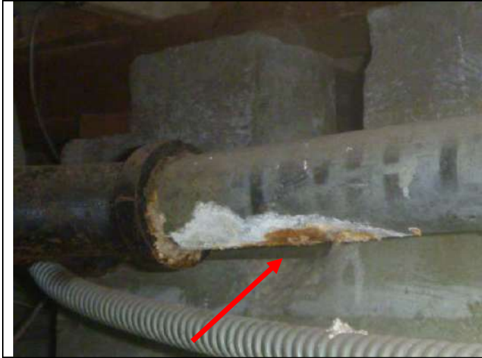
Rusted drain piping.
