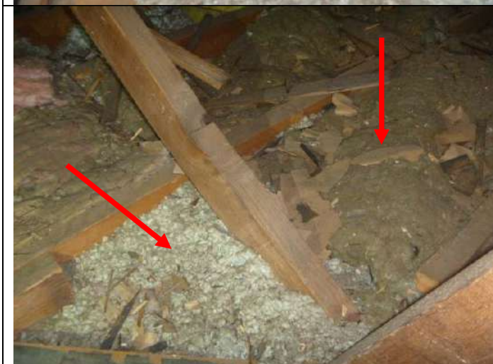
Old and thin attic insulation.
