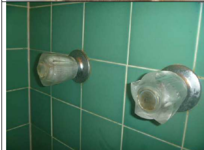
3/4 bathroom older shower fixtures. Note: The hot water valve squeaks during operation. The cold water valve is relatively stiff.
