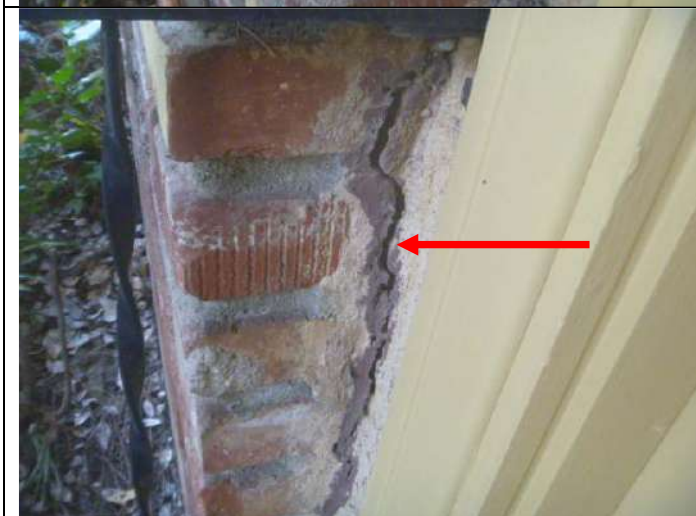
Gap along the side of the brick wall to the left of the front porch.
