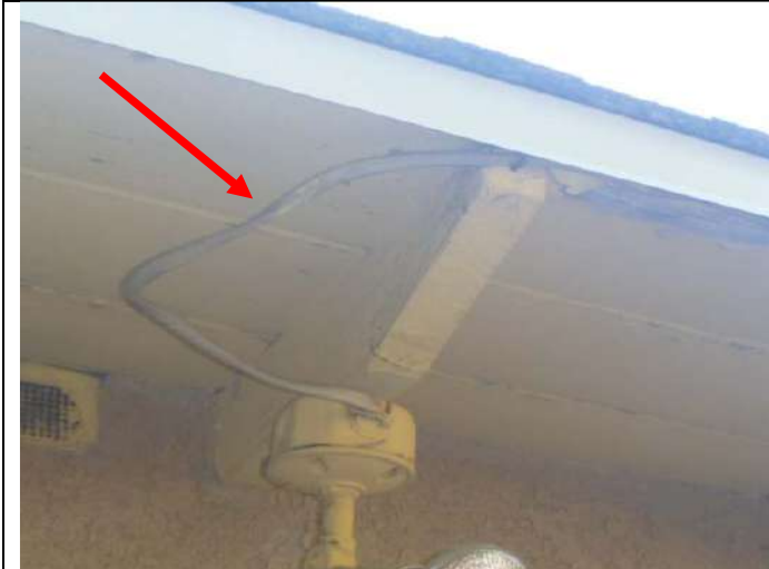
Unprotected nonmetallic cable (Romex) wiring and plug assembly along the east eave.
