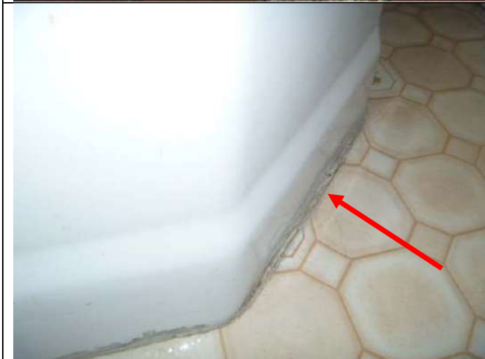
Slightly lifted flooring at the tub.
