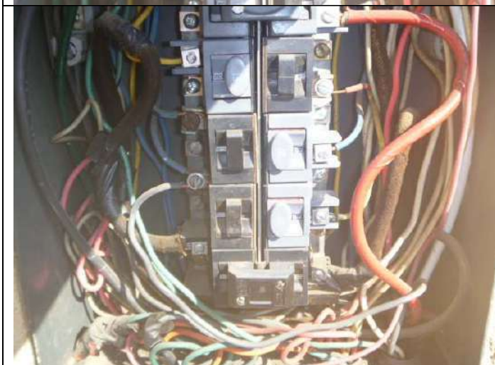
A closer view of the lower breakers.
