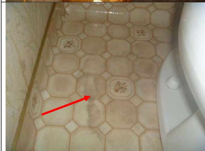
Discoloration in the flooring at the 3/4 bathroom toilet.
