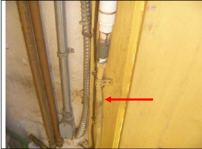
Underside drain for the water heater pressure relief valve.
