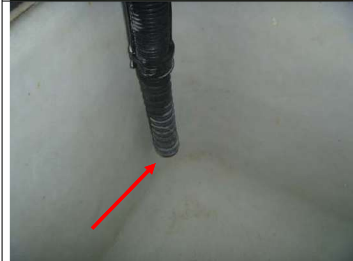
Washer draining into the sink.
