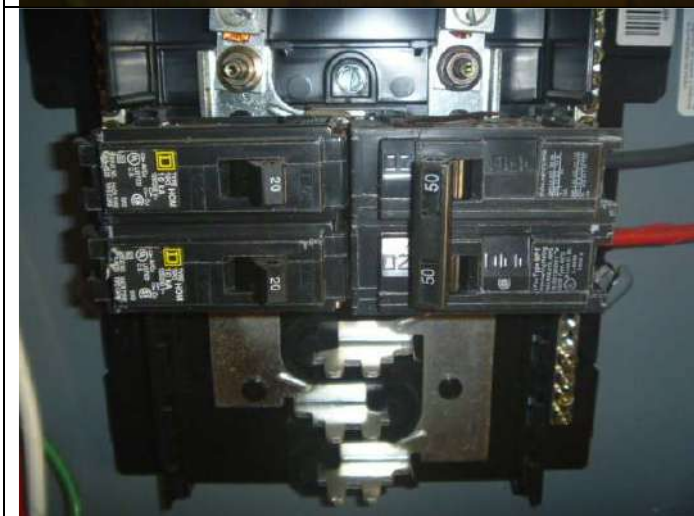
A closer view of the breakers. Note: The 20 amp breakers are not in use.
