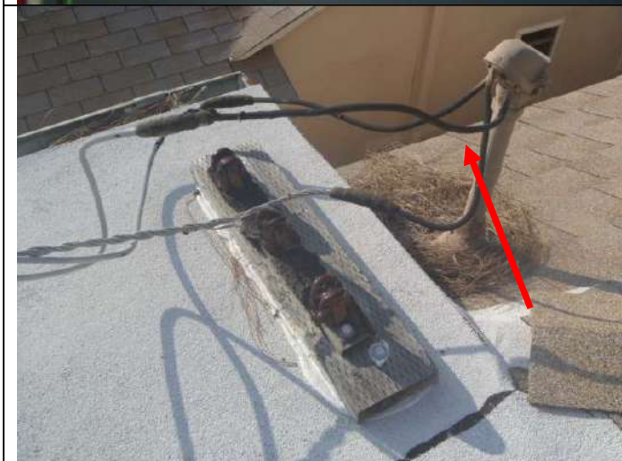
Older style electrical service entrance.
