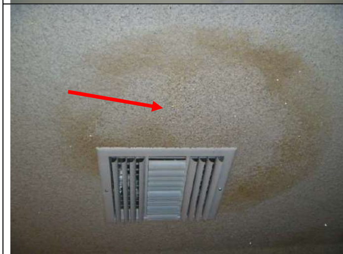
Family room ceiling discoloration at the heating/air conditioning register.
