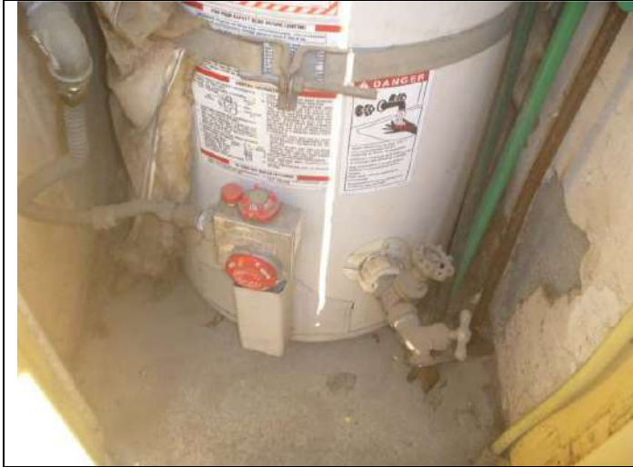
Water heater lower section.
