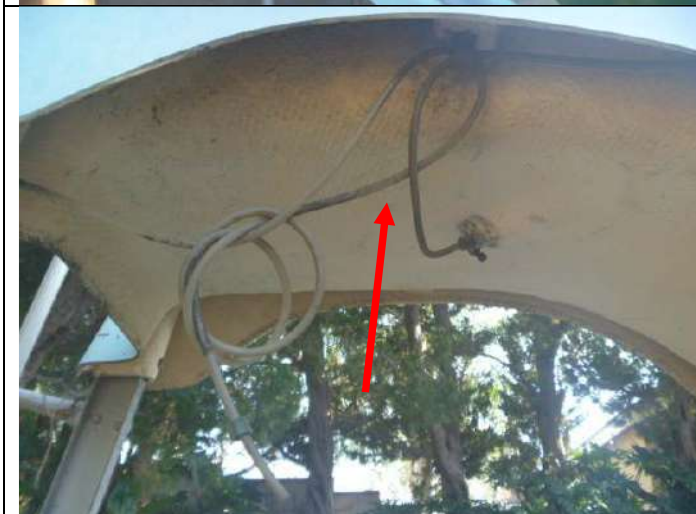
Pool slide disconnected water line.
