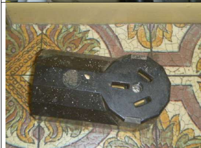
240 volt receptacle for an electric dryer.
