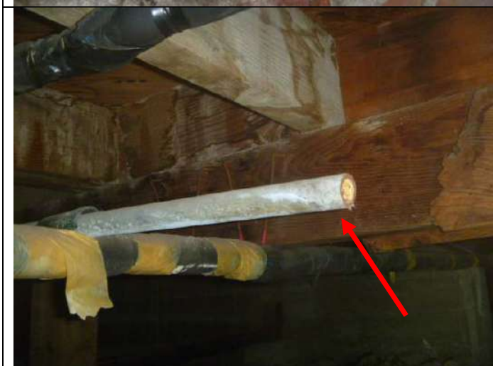
Old galvanized water piping (not in use) not removed from the foundation crawlspace.
