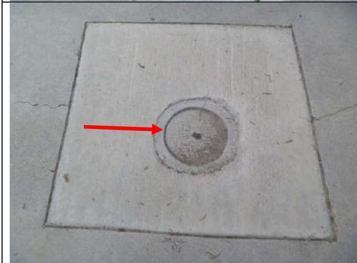
Drain cleanout at the left front exterior.
