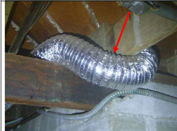
Dryer vent flexible duct in the foundation crawlspace.
