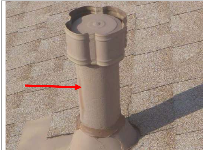
Water heater vent pipe (transite type).
