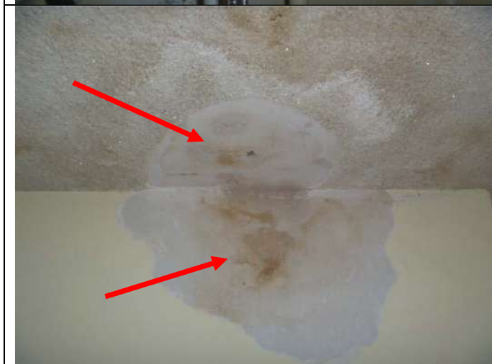
Living room wall and ceiling damage at the upper rear.
