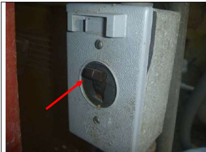
Missing switch cover at the pool equipment.
