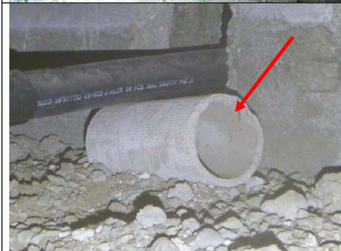
Transite vent piping remnant (from the original heater) in the foundation crawlspace.
