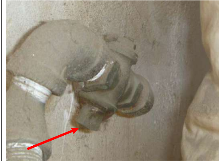
Water heater gas shut off valve requiring a tool for operation.
