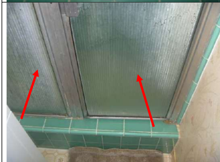
3/4 bathroom shower enclosure (older non-tempered glass type).
