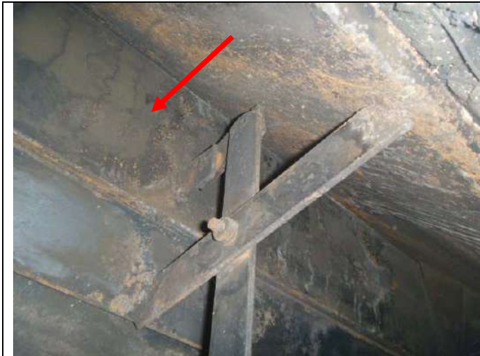
Fireplace damper in the closed position. Note: The damper should be secured open as natural gas logs are in use.
