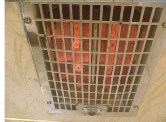
3/4 bathroom older heater.
