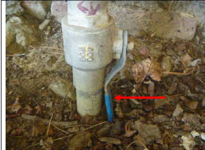
Main water valve.
