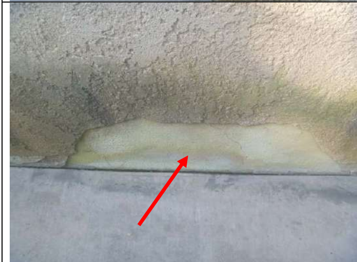
Stucco damage and discoloration at the lower left rear exterior wall.
