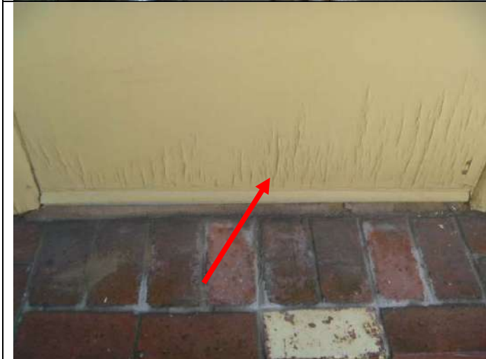
Deterioration in the full bathroom exterior door.
