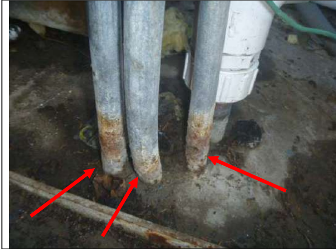
Rusted electrical conduit at the pool equipment.
