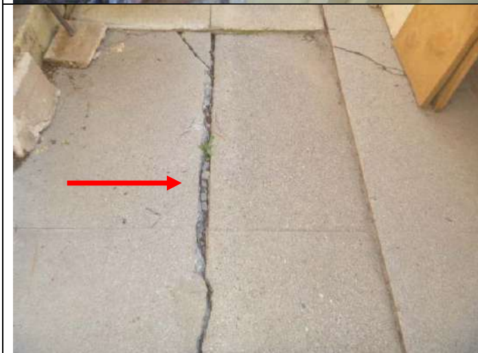
West side walkway cracking and unevenness.
