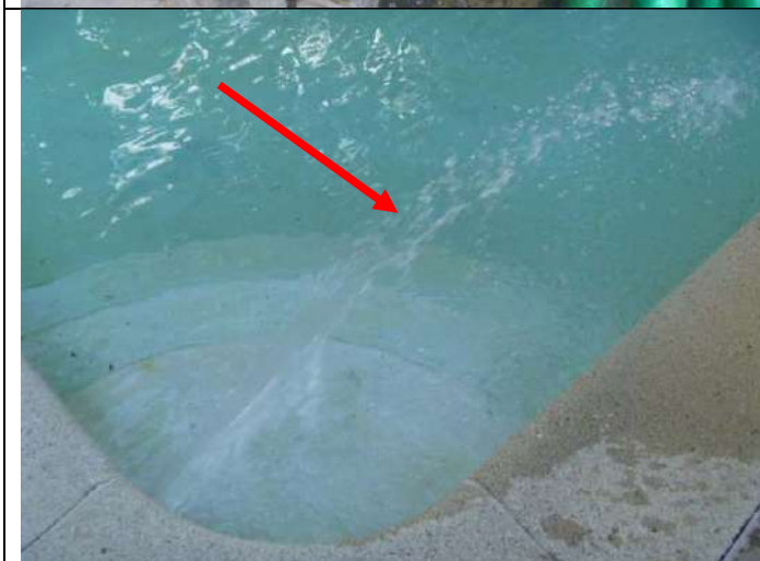
Pool fill valve water with irregular spray pattern.
