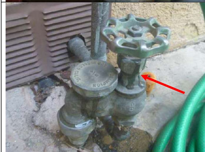
Pool water fill valve leaking during operation.
