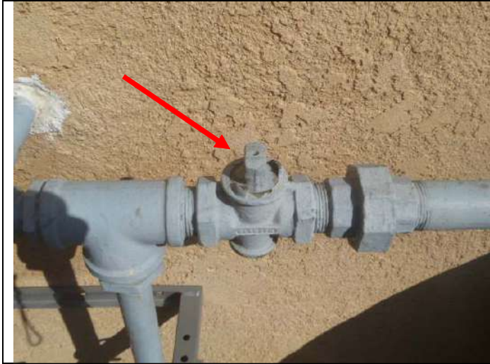
Pool heater gas shut off valve turned off.
