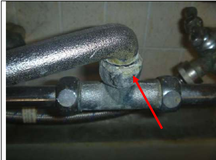
Leak at the base of the laundry sink spout.
