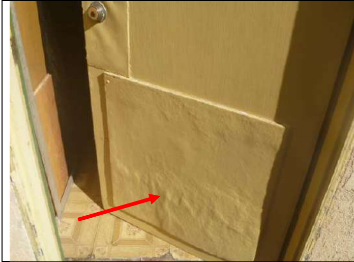
Garage damaged side exterior door.
