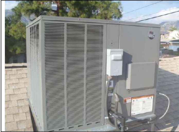
Heating/air conditioning unit.
