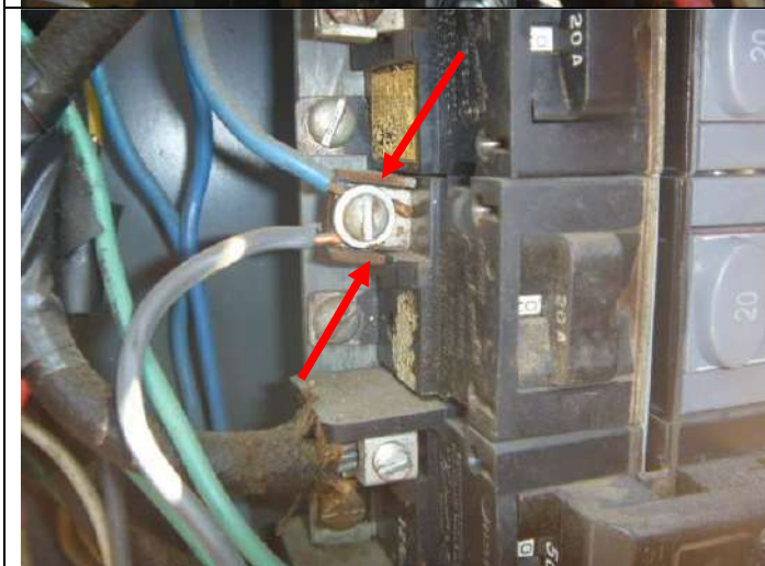
Double tapped 20 amp breaker.
