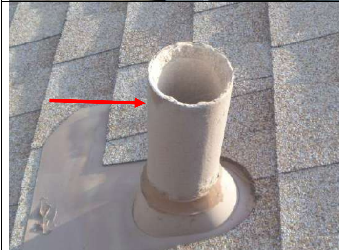
Main plumbing vent pipe (transite type).
