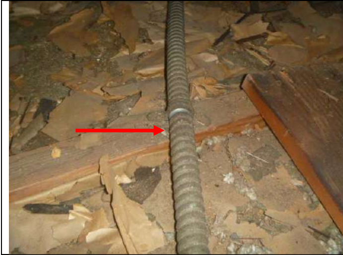
Flexible conduit electrical wiring. Note: The majority of the wiring is this type.
