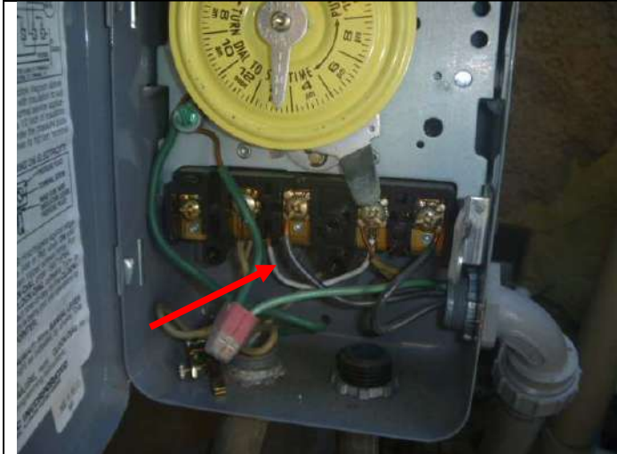
Missing insulating cover below the pool timer. Note: The timer is no longer needed.
