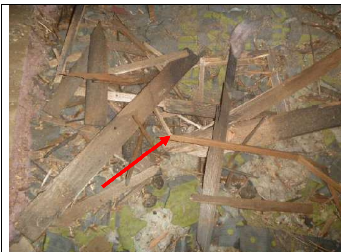
Loose wood debris (from the original wood shingle roof) in the attic.
