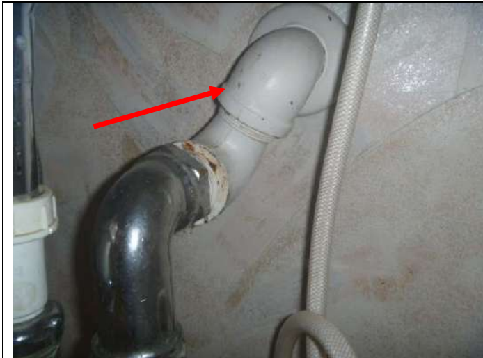
Full bathroom sink drain piping with upward section at the wall.
