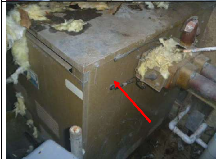
Pool heater (old and inoperative).
