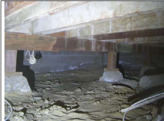
Foundation crawlspace. Note: The wet soil.
