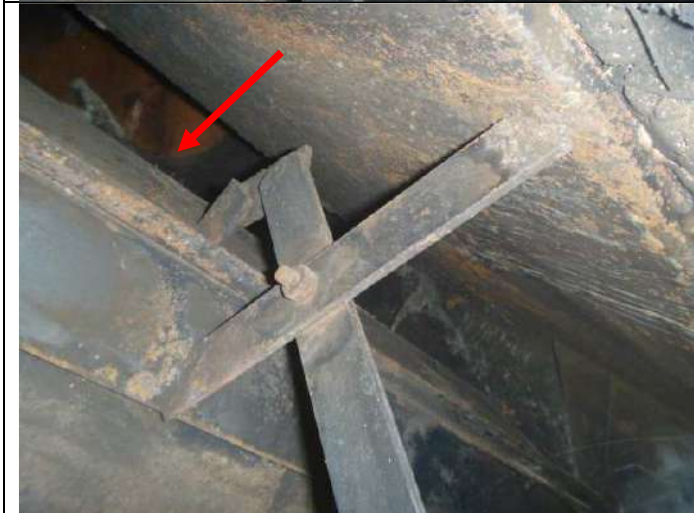
Fireplace damper in the open position.
