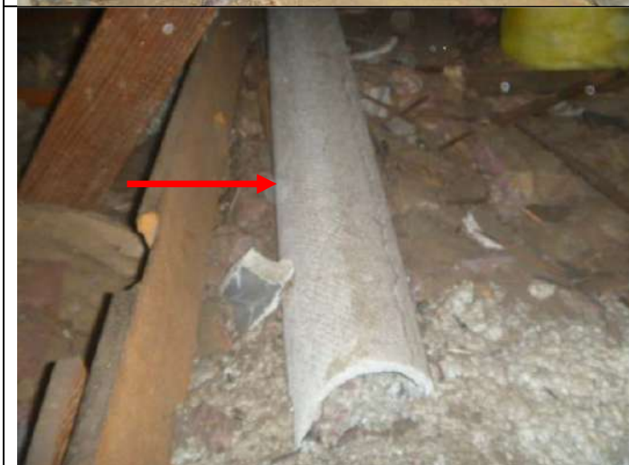
Transite vent piping remnant in the attic.
