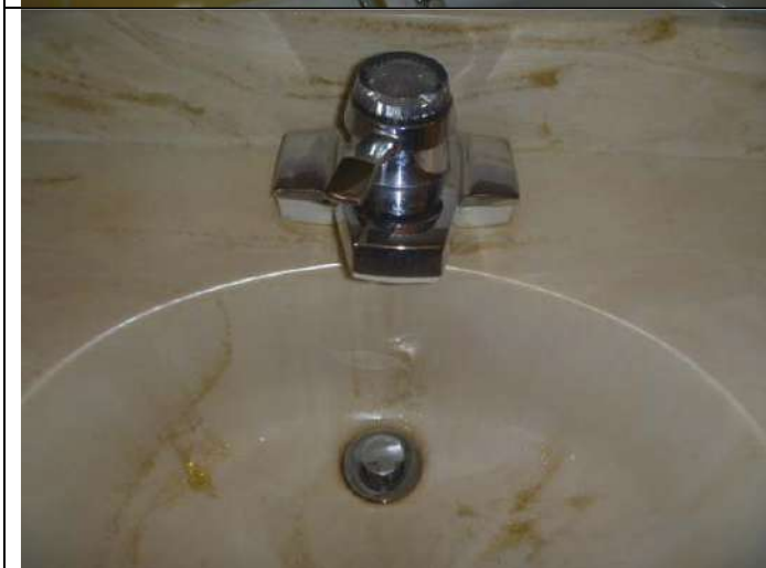
Full bathroom older sink faucet.
