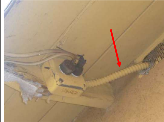
Flexible conduit wiring, not rated for exterior use, under the east eave.
