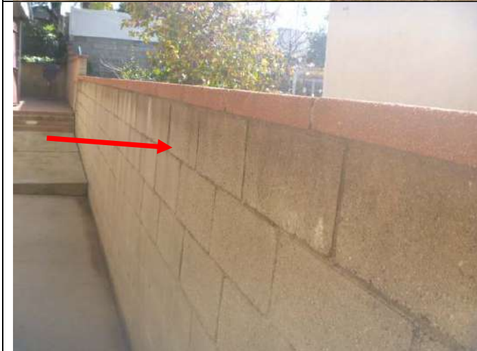
Slightly leaning west side block wall.
