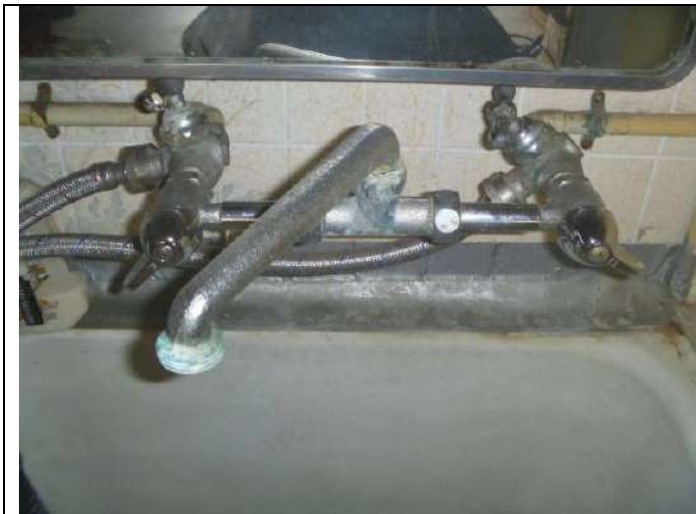
Laundry sink faucet and washer valves.
