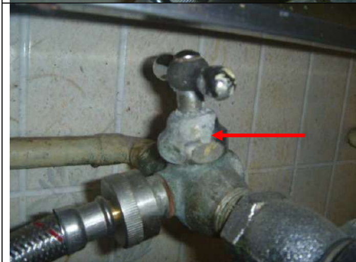
Washer hot water valve.
