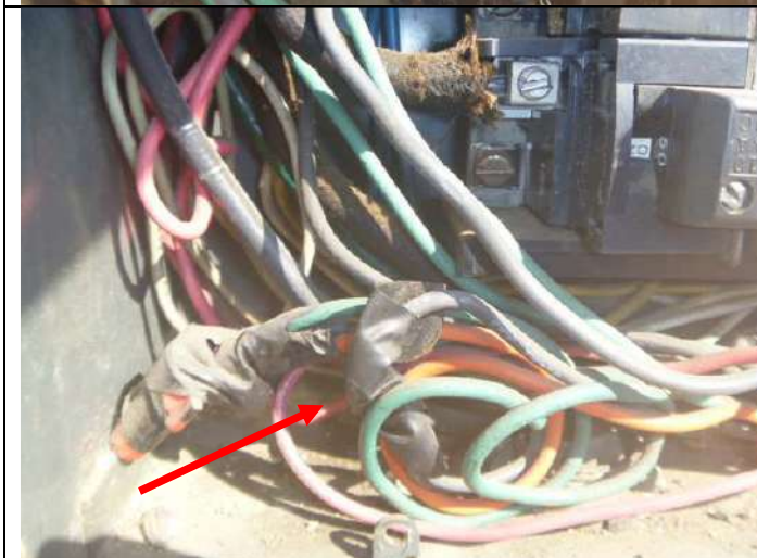
Relatively "messy" wiring within the panel
