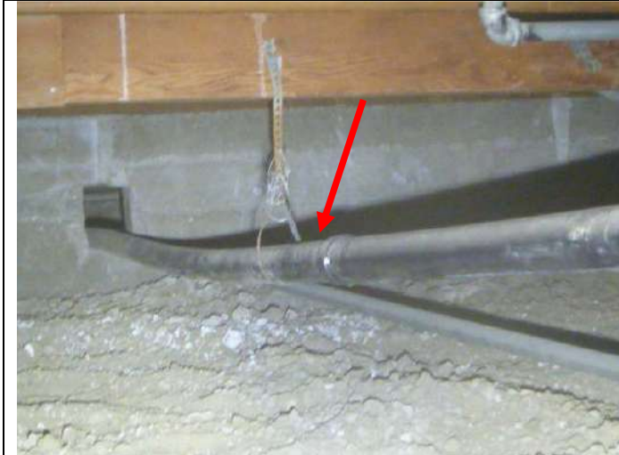
A sagged replacement ABS drain pipe.
