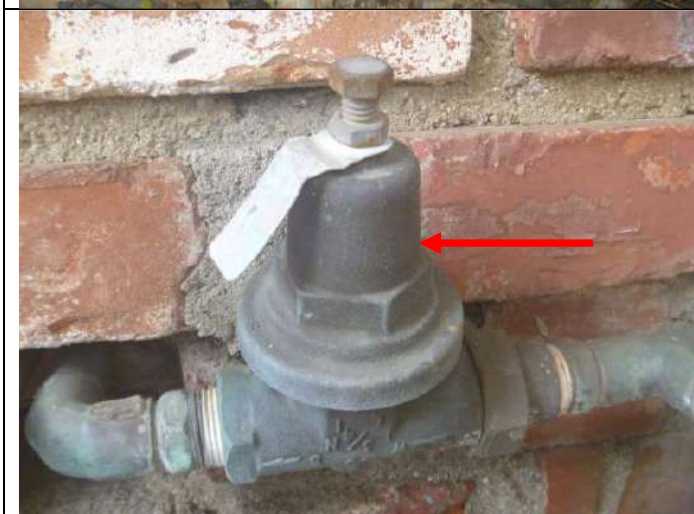
Water pressure regulator and copper water piping.
