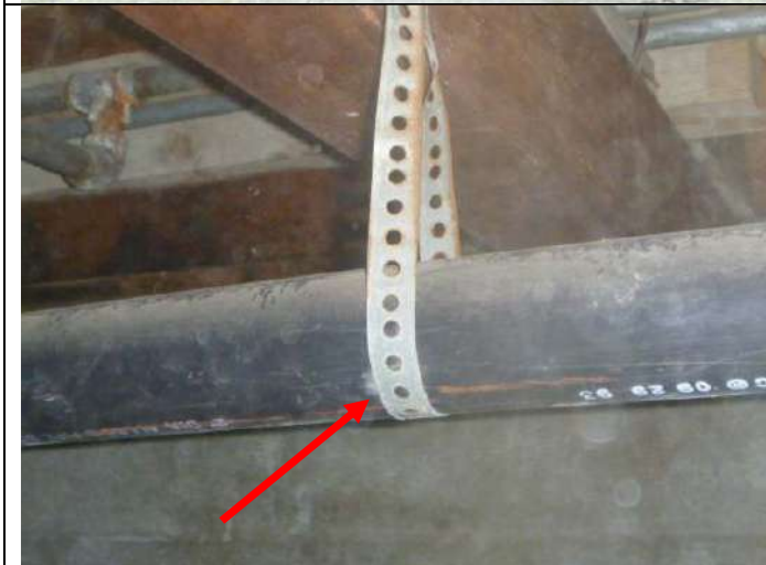
ABS drain piping braced with metal (vs. nonmetallic) strap.
