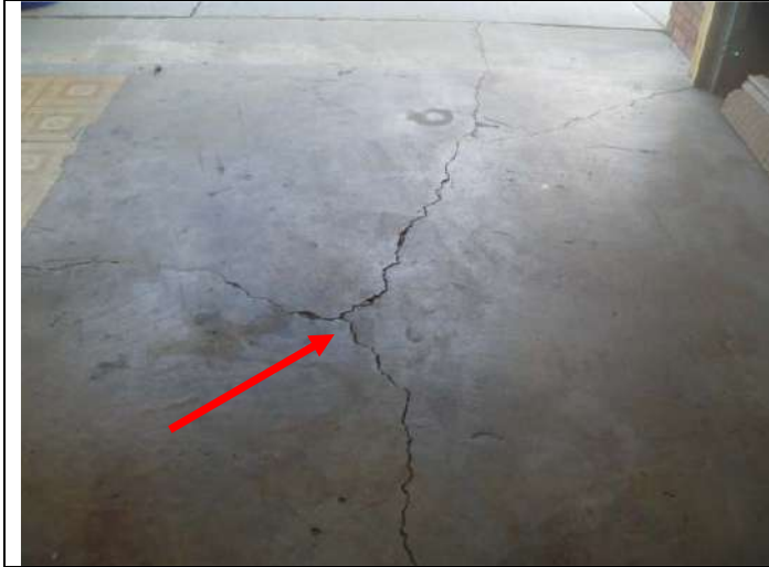
Settlement cracks in the garage slab floor.
