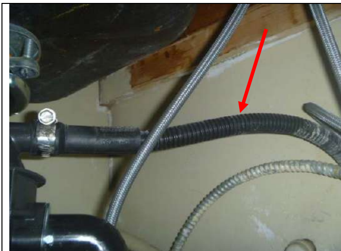
Dishwasher drain line without an air gap.
