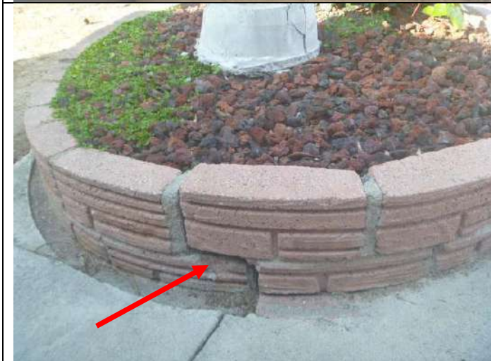
Displacement in the left front planter (at the tree).
