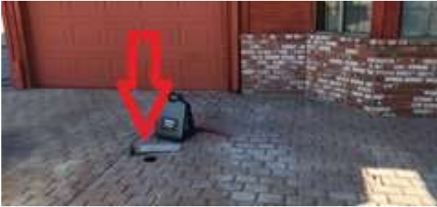
Location of driveway cleanout
