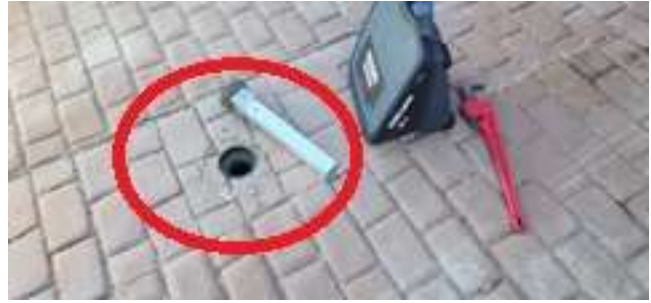
Cleanout in driveway
