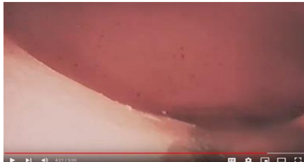
City sewer connection
