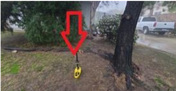
Location of heavy root in line. About 5 ft deep
