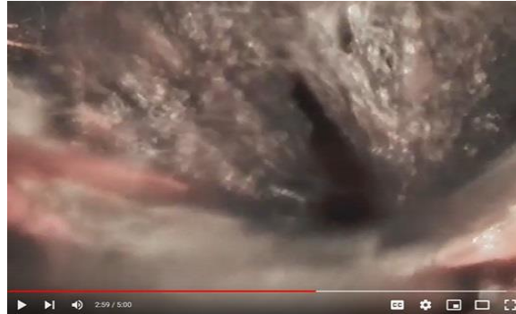
Roots in sewerline
