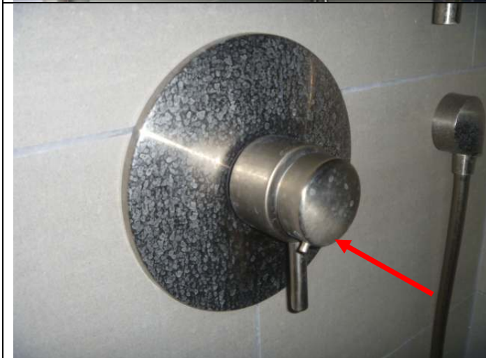
3/4 bathroom shower fixtures. Note: The valves are relatively stiff.
