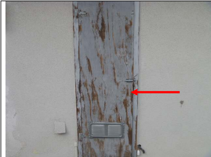
Water heater compartment door. Note: The door is in poor condition and without an upper combustion air opening.
