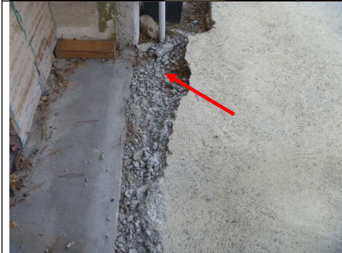
Driveway breakage and unevenness at the right front of the garage.
