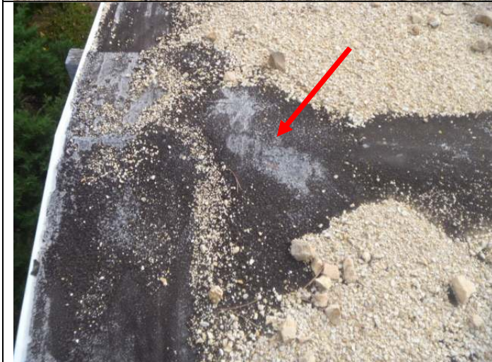
Missing gravel and deteriorated roofing material.
