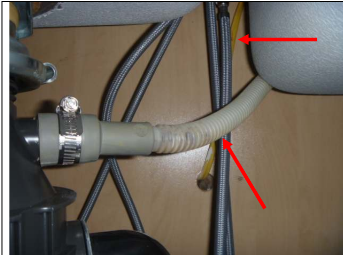
Dishwasher drain line without an air gap. Unprotected nonmetallic cable (Romex) wiring below the sink.
