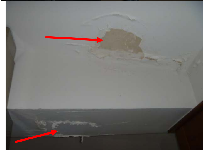
Kitchen ceiling damage to the right of the range hood.
