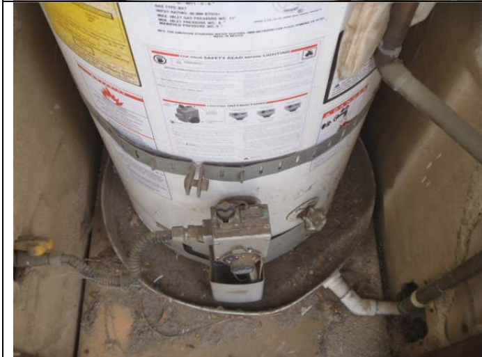
Water heater lower section.
