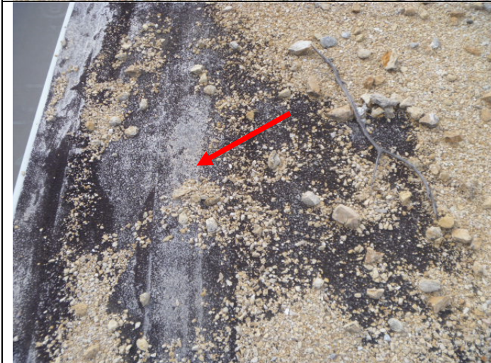
Missing gravel and deteriorated roofing material.
