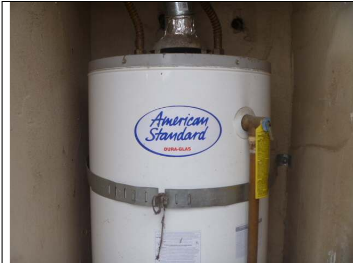
Water heater upper section.
