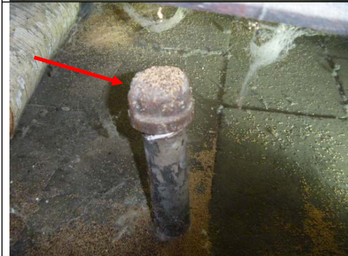
Capped gas pipe in the fireplace.
