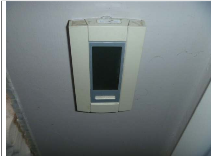
Control for the full (primary) bathroom floor heater.
