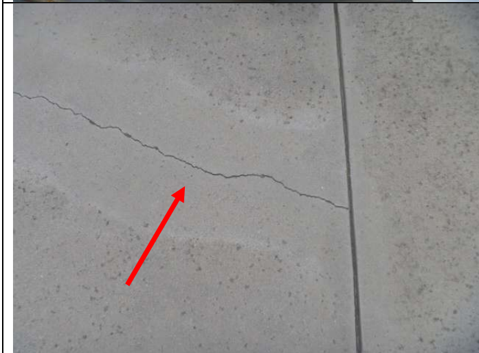
Minor crack in the right rear patio.
