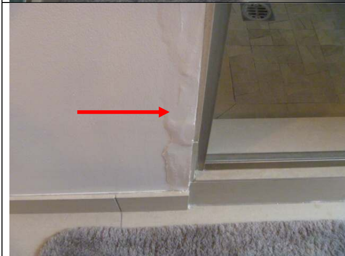
Wall damage at the lower left of the 3/4 bathroom shower door.
