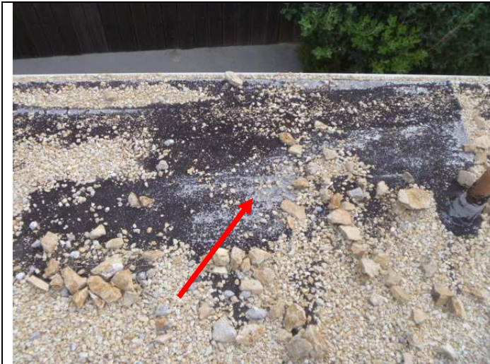
Missing gravel and deteriorated roofing material.
