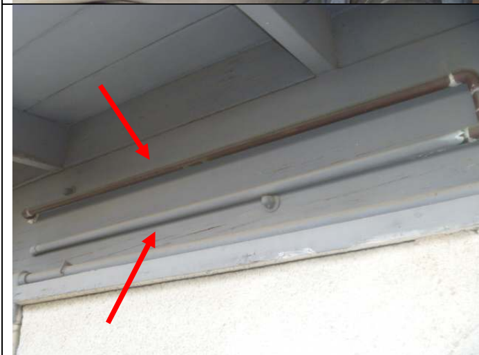
Surface mounted water piping along the upper east exterior wall (off the kitchen).
