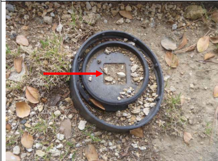
Drain cleanout at the left front exterior of the garage.
