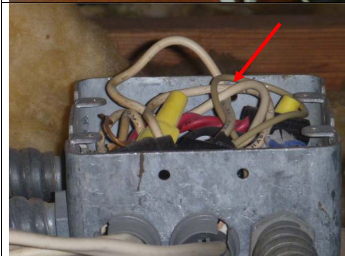
Open electrical box in the attic.
