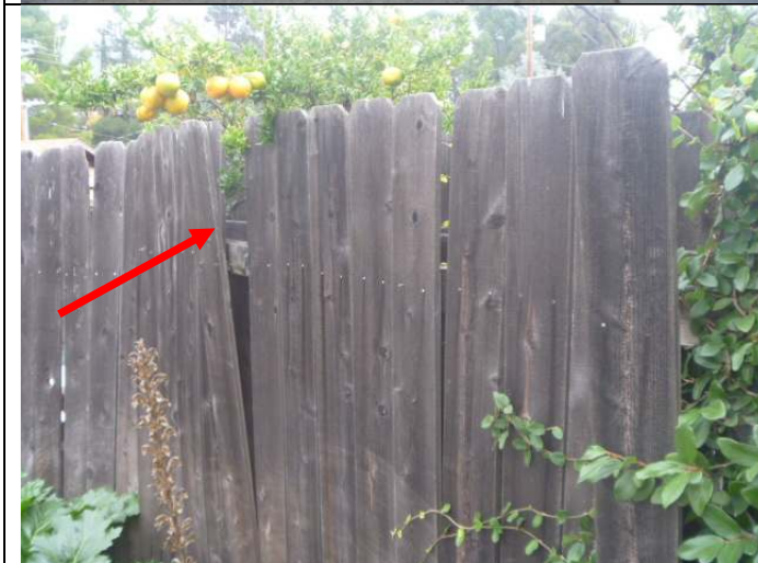
Damaged east side wood fencing.
