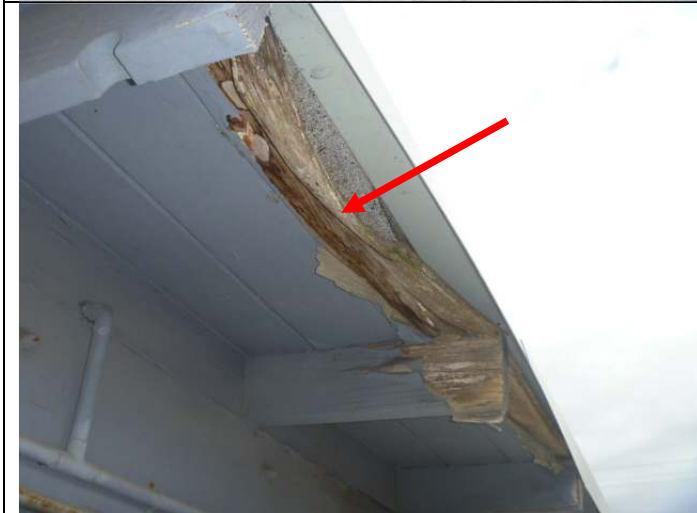
Example of damaged wood along the east eave. Note: There is additional damaged wood in multiple areas (including along the garage eaves).
