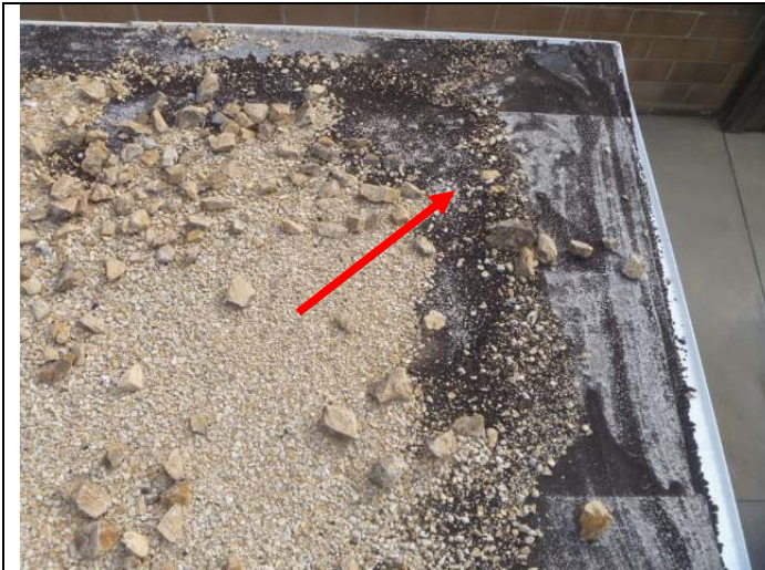
Missing gravel and deteriorated roofing material.
