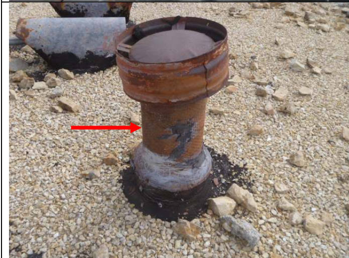
Original heater transite vent pipe (not in use).
