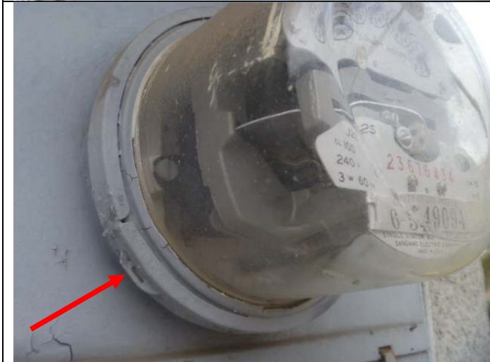
Electric meter not locked in place.
