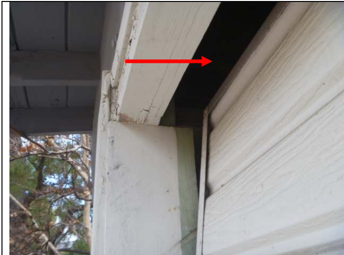
Garage door not closing completely.
