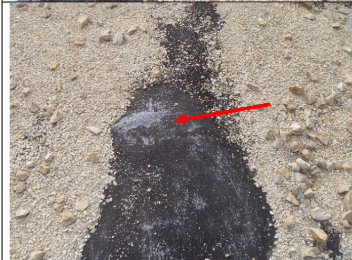
Missing gravel and deteriorated roofing material.
