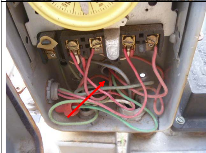
Missing insulating cover below the pool/spa timer. Note: The timer is not needed as the pump has an integral timer.
