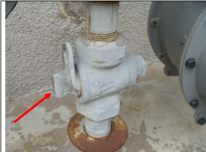
Gas shut off valve.
