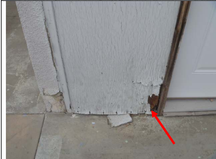
Damaged siding at the garage lower rear wall.
