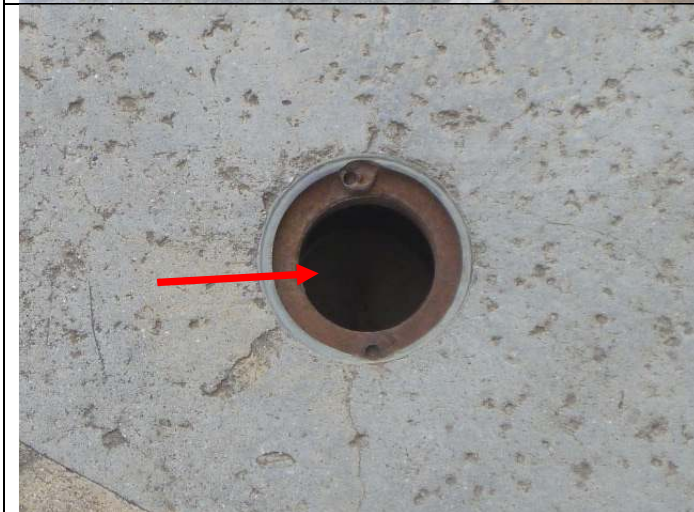
A missing exterior surface drain cover.
