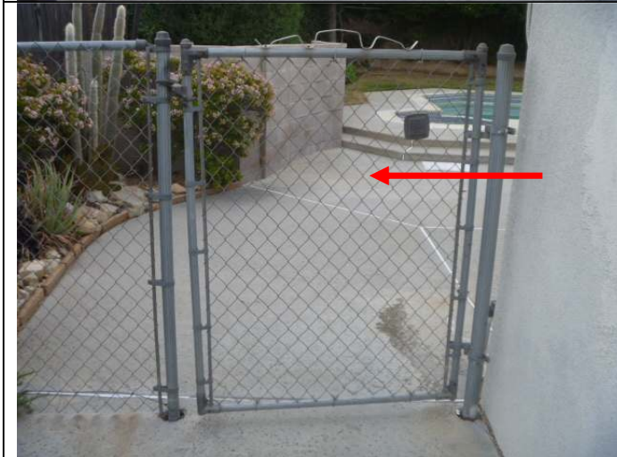
Left rear gate with pool/spa area access. Note: The gate is not properly self-closing and must be lifted to latch.
