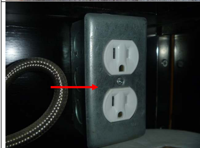
Surface mounted receptacle, without ground fault circuit interrupter (GFCI) protection, below the 3/4 bathroom sink.
