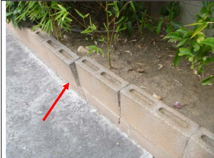
Leaning west block planter wall (toward the right rear).
