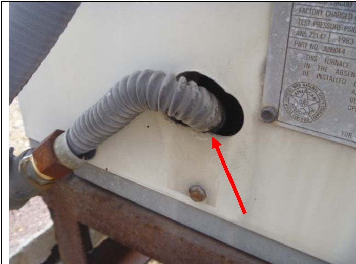
Flexible gas connector, subject to damage, routed through the heating/air conditioning unit housing.
