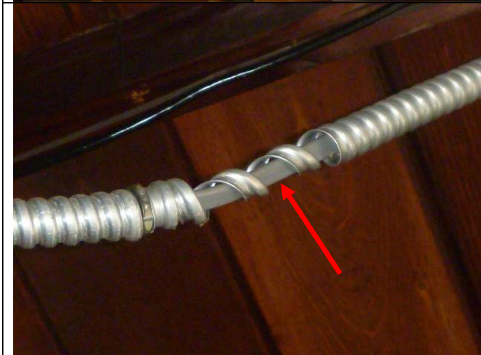
Separated electrical conduit (overhead toward the left rear) in the garage.
