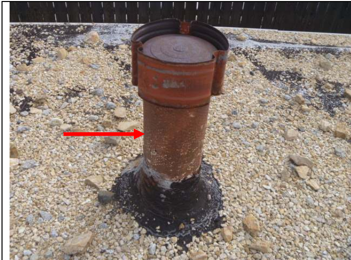
Water heater transite vent pipe.
