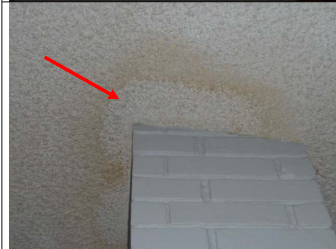
Discoloration in the living room ceiling at the fireplace.
