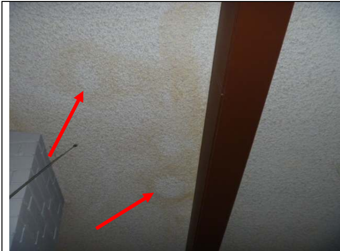
Discoloration in the dining room ceiling.
