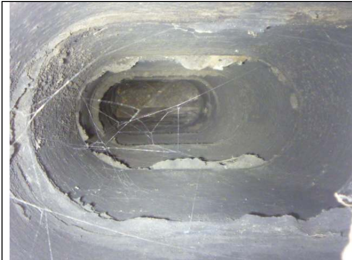
View down the chimney flue.
