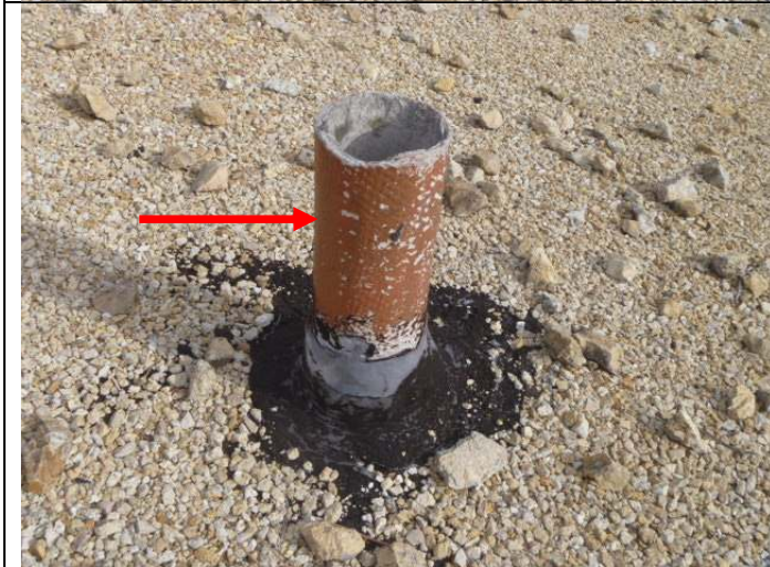
Main plumbing vent pipe (transite type).
