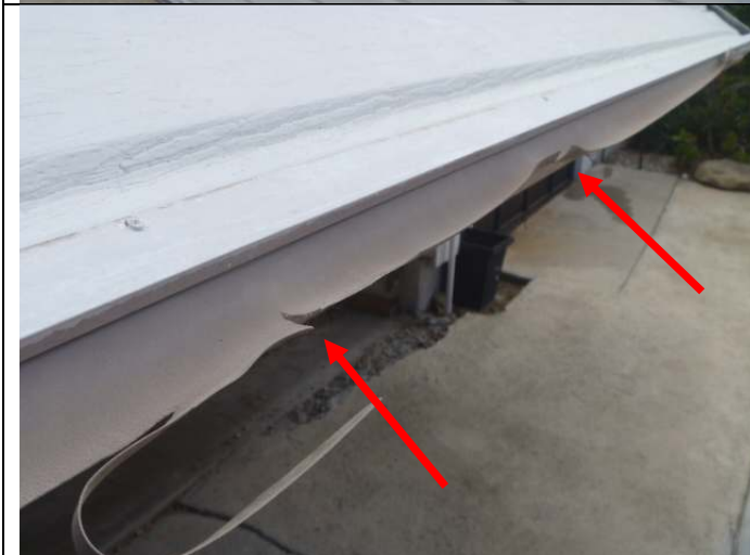
Damaged weather stripping along the bottom on the garage door.
