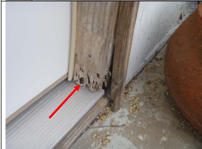
Damaged wood at the garage rear exterior doorjamb.
