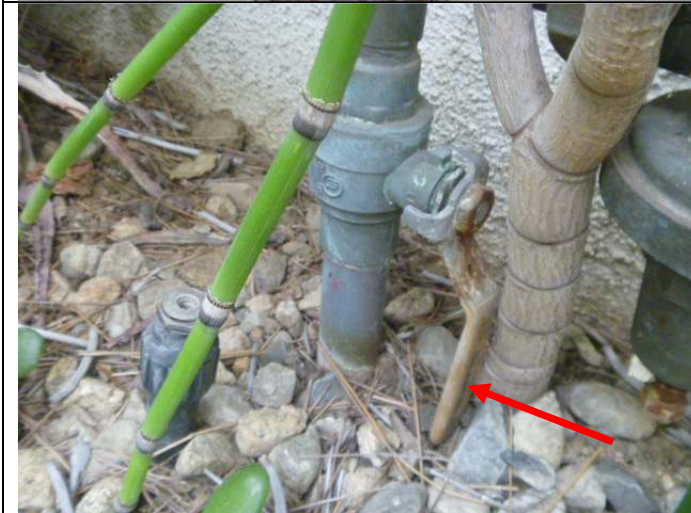
Main water valve.
