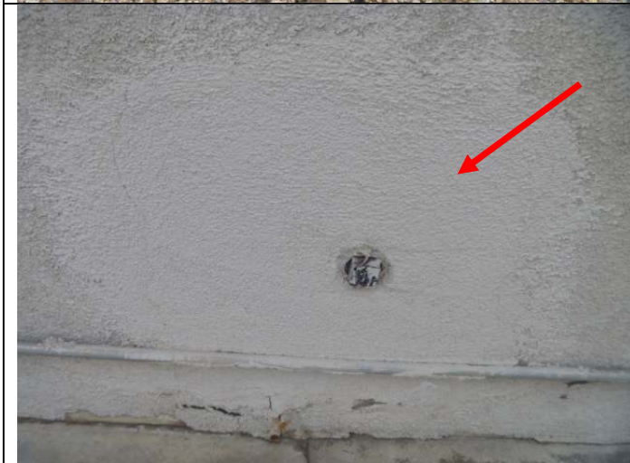
Stucco repair at the lower north exterior wall.
