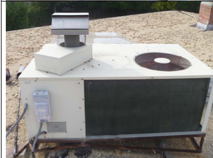
Heating/air conditioning unit.
