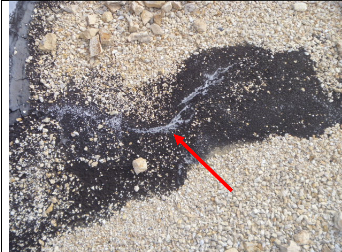
Missing gravel and deteriorated roofing material.
