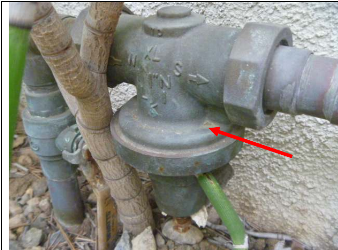
Water pressure regulator.
