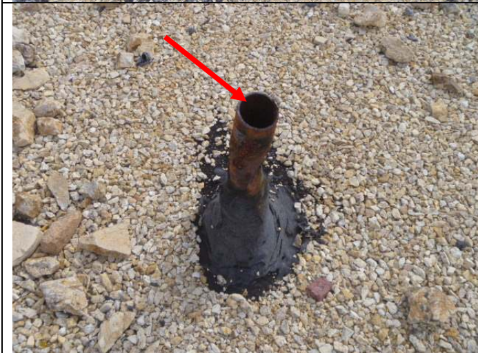
Open pipe (possibly for a previous roof mounted antenna) toward the left rear.
