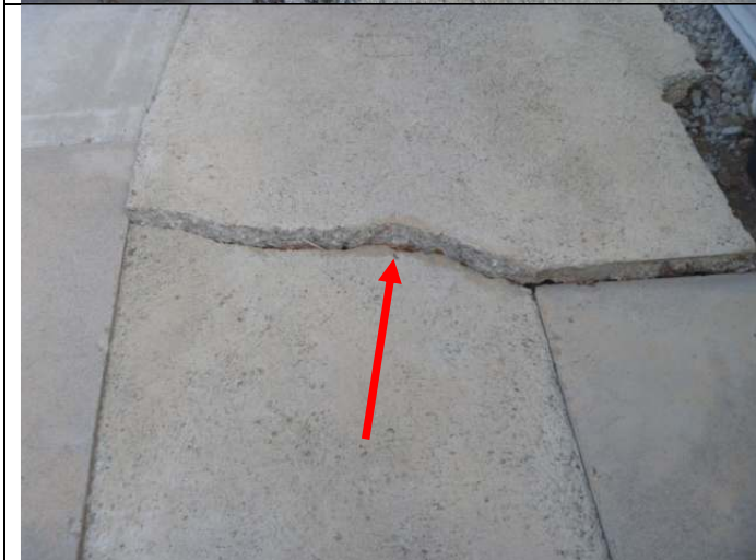
Driveway cracking and unevenness at the right front of the garage.
