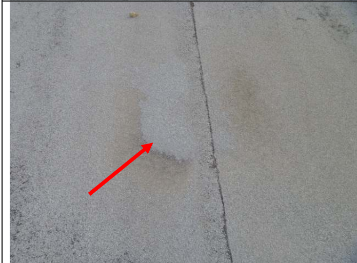
Evidence of standing water.
